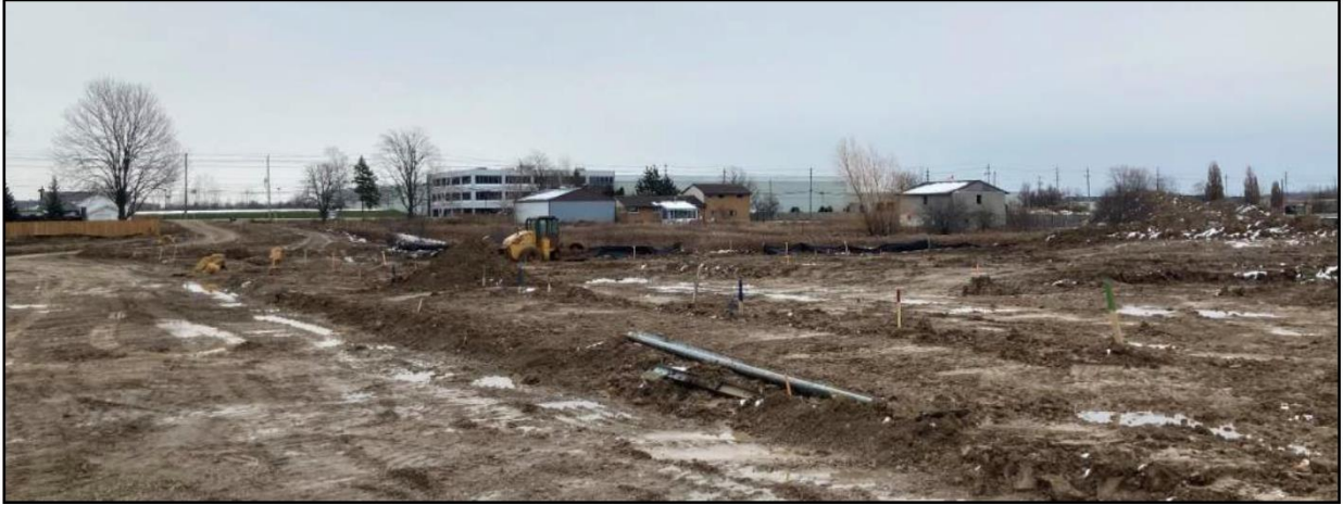
Viewing from the northwest of the site looking east toward White Oak Road. *Note, the extension of Petty Road currently under construction in the foreground.
