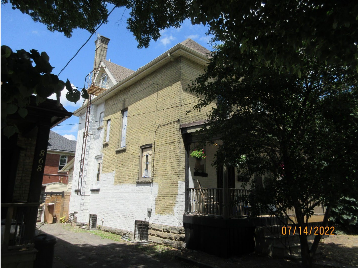
Image 6: Photograph of the heritage designated property at 870 Queens Avenue, on July 14, 2022, showing painting on the west façade.
