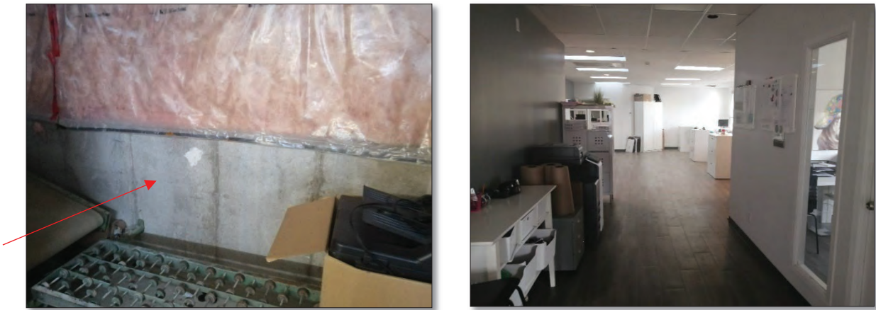
Figures 32 & 33: (left) View of poured concrete foundation in basement; (right) View of interior of second floor (MHBC, 2022).
