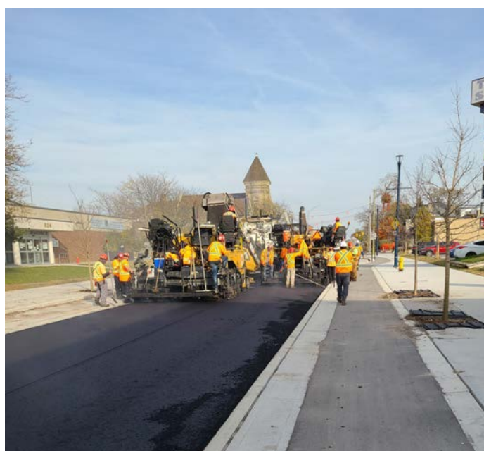
Paving top surface on Dundas Street in OEV
