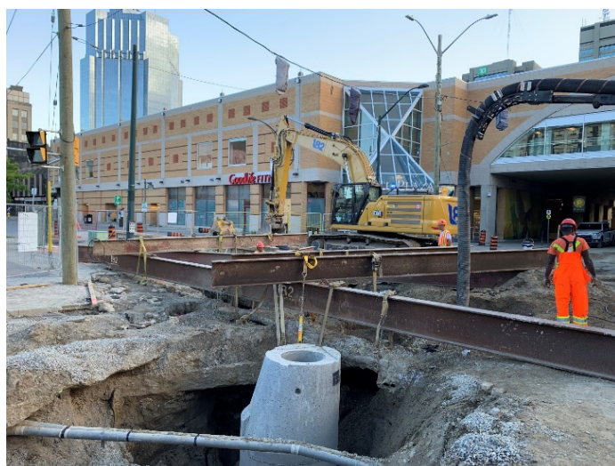
New maintenance hole structure supported by multiple beams at Clarence and King intersection
