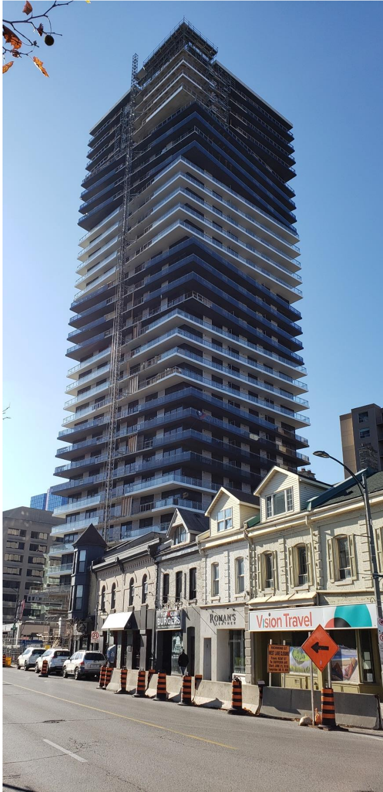
517 Richmond Street a 31-story building nearing construction completion November 14, 2020. This residential building is across the street from the Victoria Park Secondary Plan and it overlooks Victoria Park.
