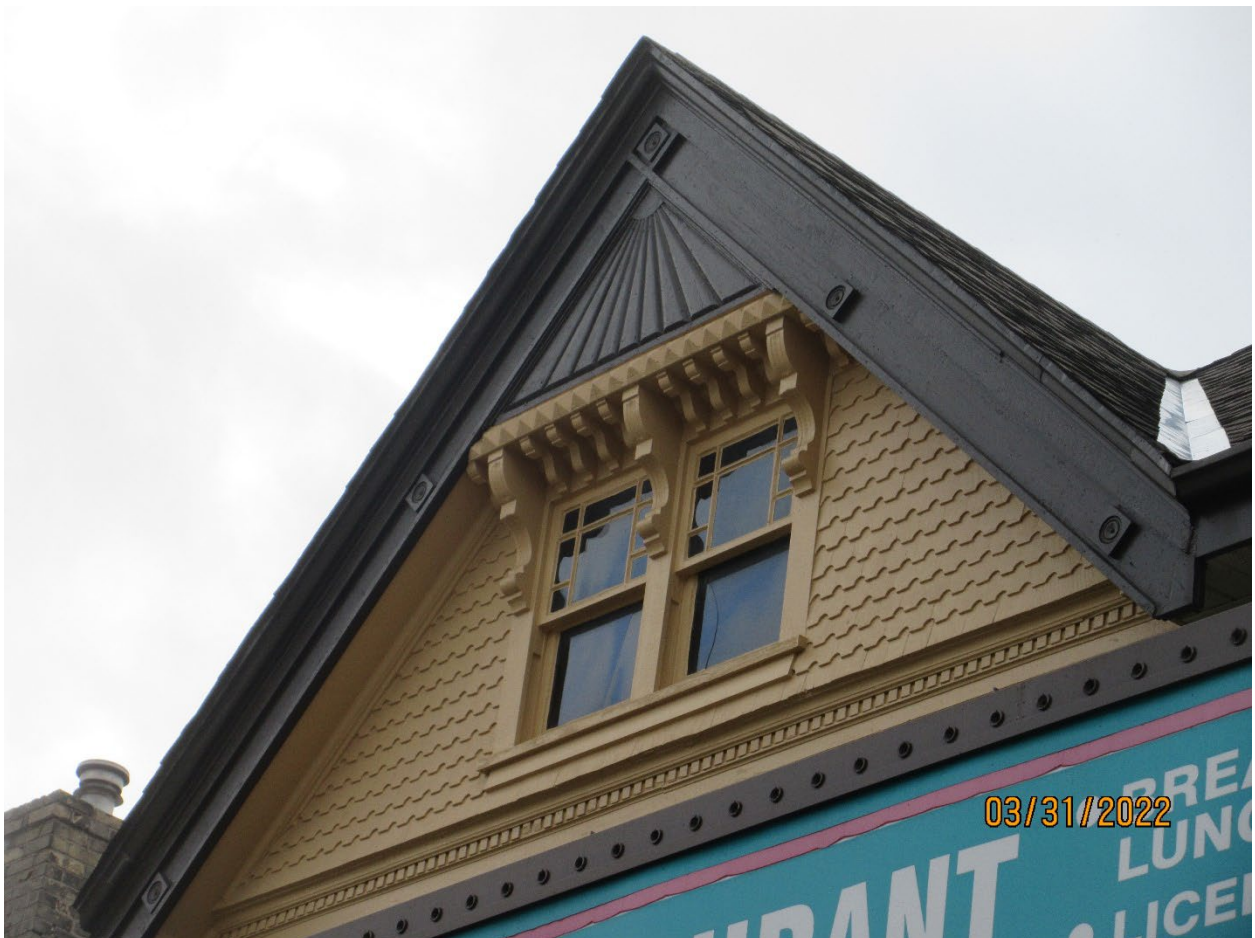
Image 4: Detail of the Queen Anne Revival detailing of the front gable, including the wood shingle imbrication, brackets, bargeboard, dentil moulding, and sunburst motif in the apex. The fenestration of the upper sash of the window is also in the Queen Anne Revival style.
