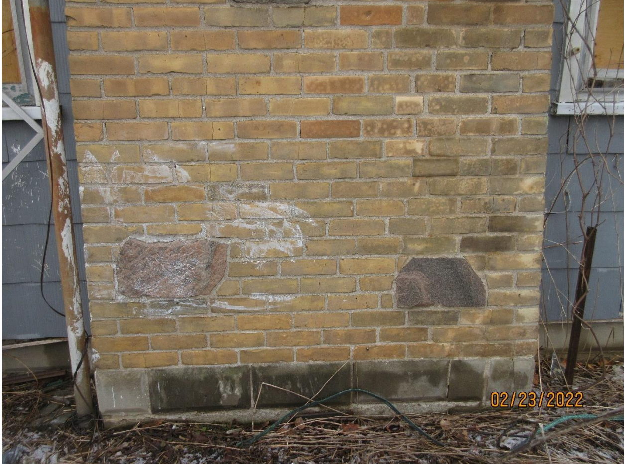
Image 10: Detail of the inset stone detailing in the brick masonry chimney on the south elevation.
