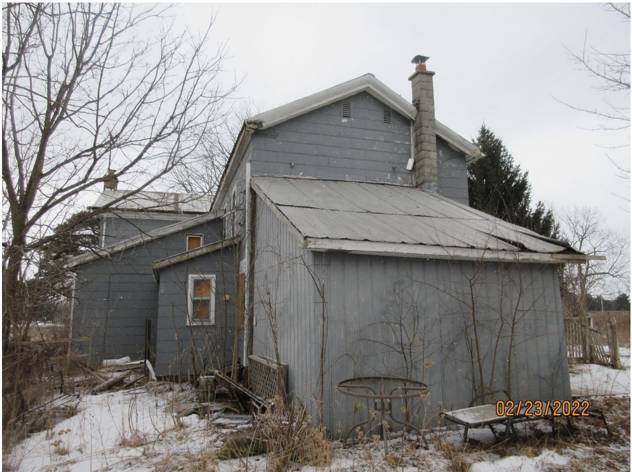
Image 6: View of the east elevation of the farmhouse at 3700 Colonel Talbot Road. Note the additions built onto the structure.
