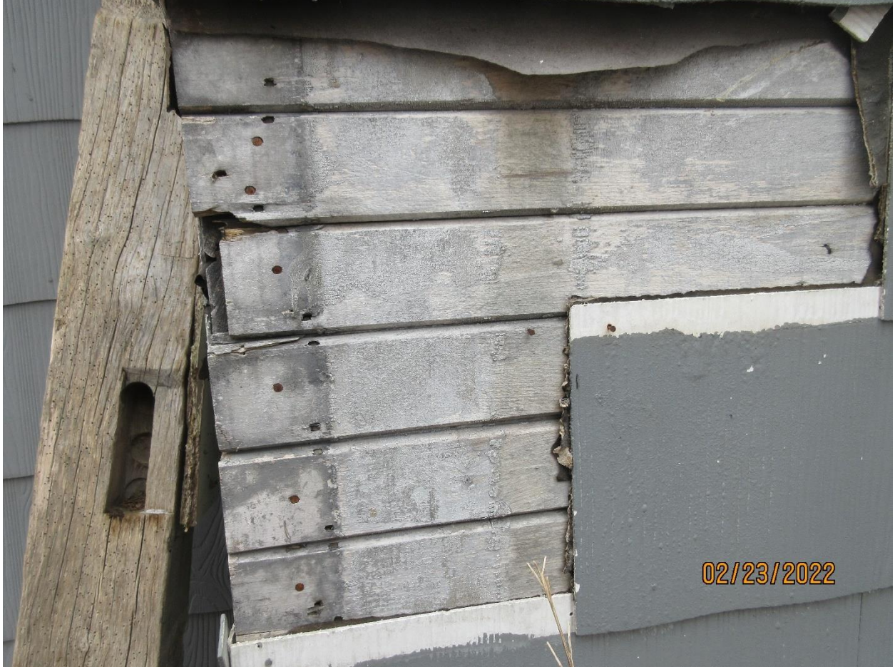
Image 8: Detail of the wood siding under the exterior cladding on the farmhouse at 3700 Colonel Talbot Road. Note the staining from previous paint, suggesting end boards.
