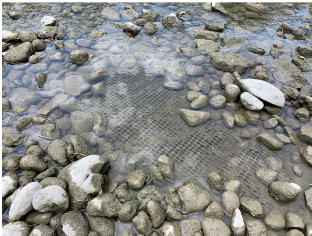
Photo 3: Partially exposed geotextile mat approximately 5 m from the east bank; Date: August 4, 2021.
