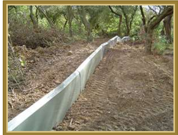
Plate 7. Pre-formed vinyl sheeting fence intended to exclude salamanders for a construction site (photo credit: Herpetosure Ltd.)
