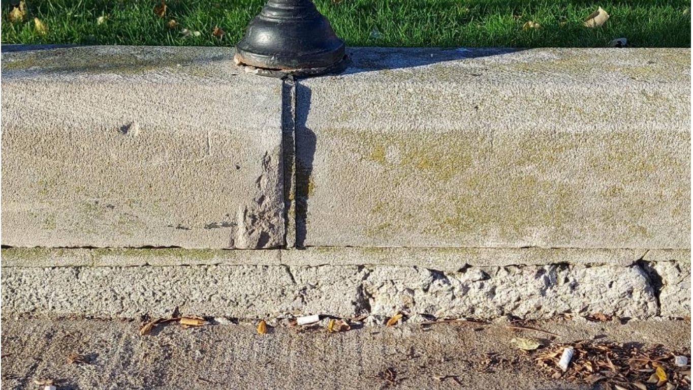
Photograph 24: View of mortar joint between cap stone and concrete foundation and mortar joint at each vertical rail post location (AECOM, November 2021)
