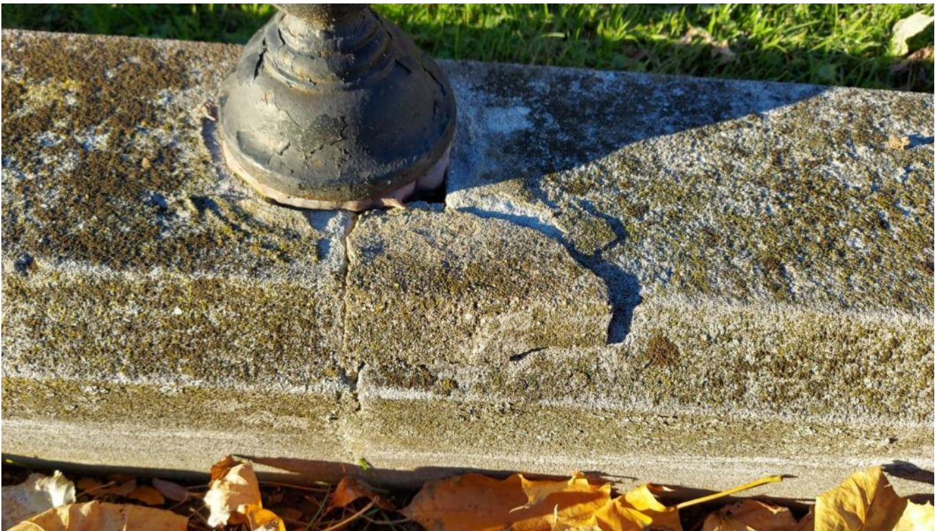
Photograph 23: Capstone cracking and spalling (AECOM, November 2021)
