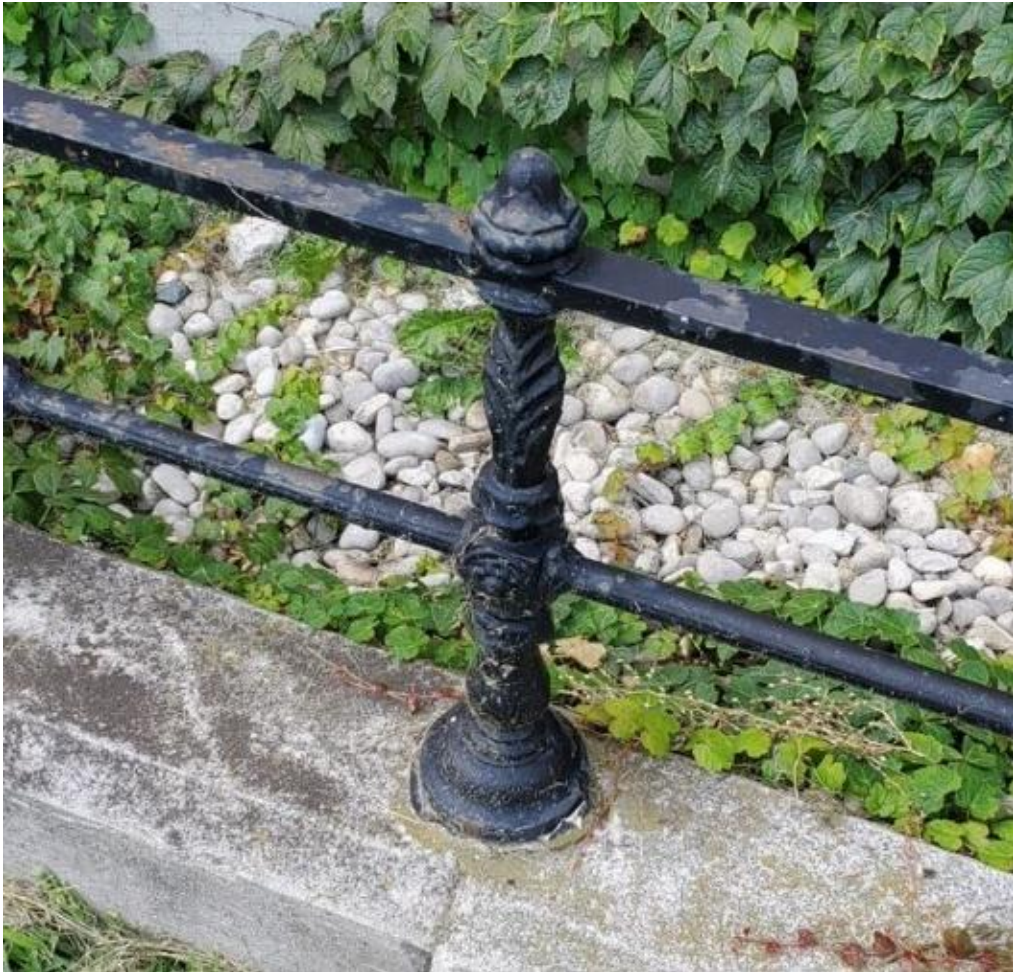
Photograph 37: Example of a vertical rail post with finial with a rounded point (AECOM, July 2021)
