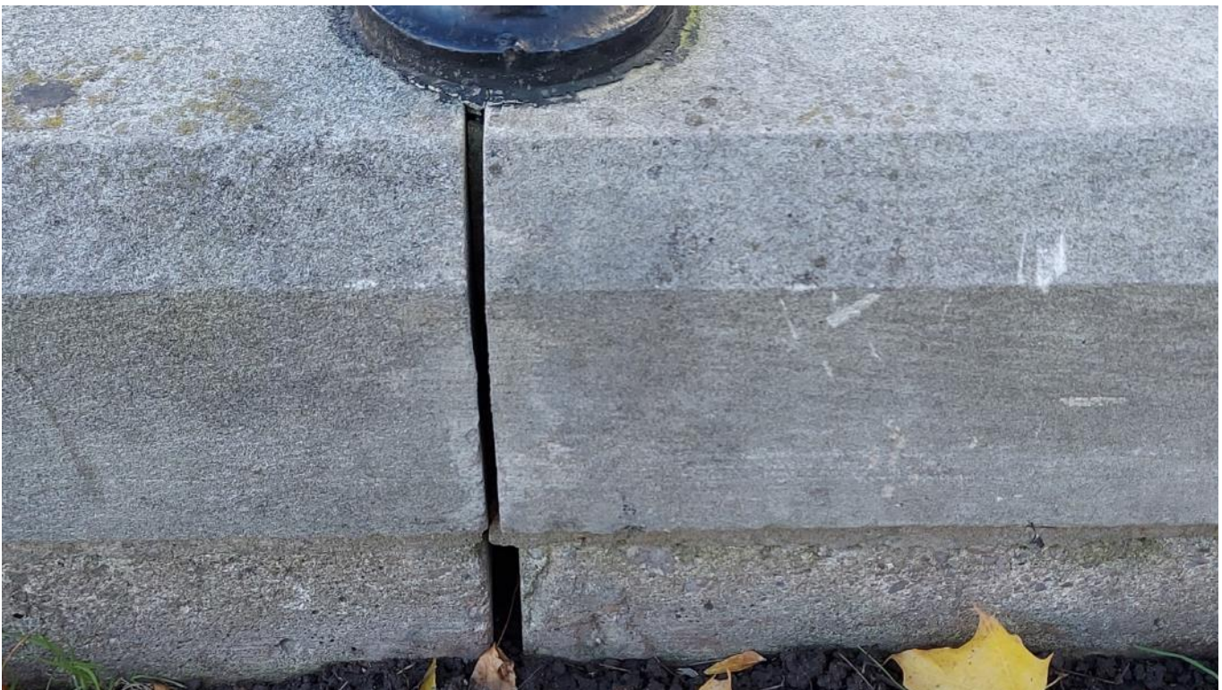
Photograph 25: Example of mortar joint missing and the cap stone cut and notched at each joint to accommodate the post attachment (AECOM, November 2021)
