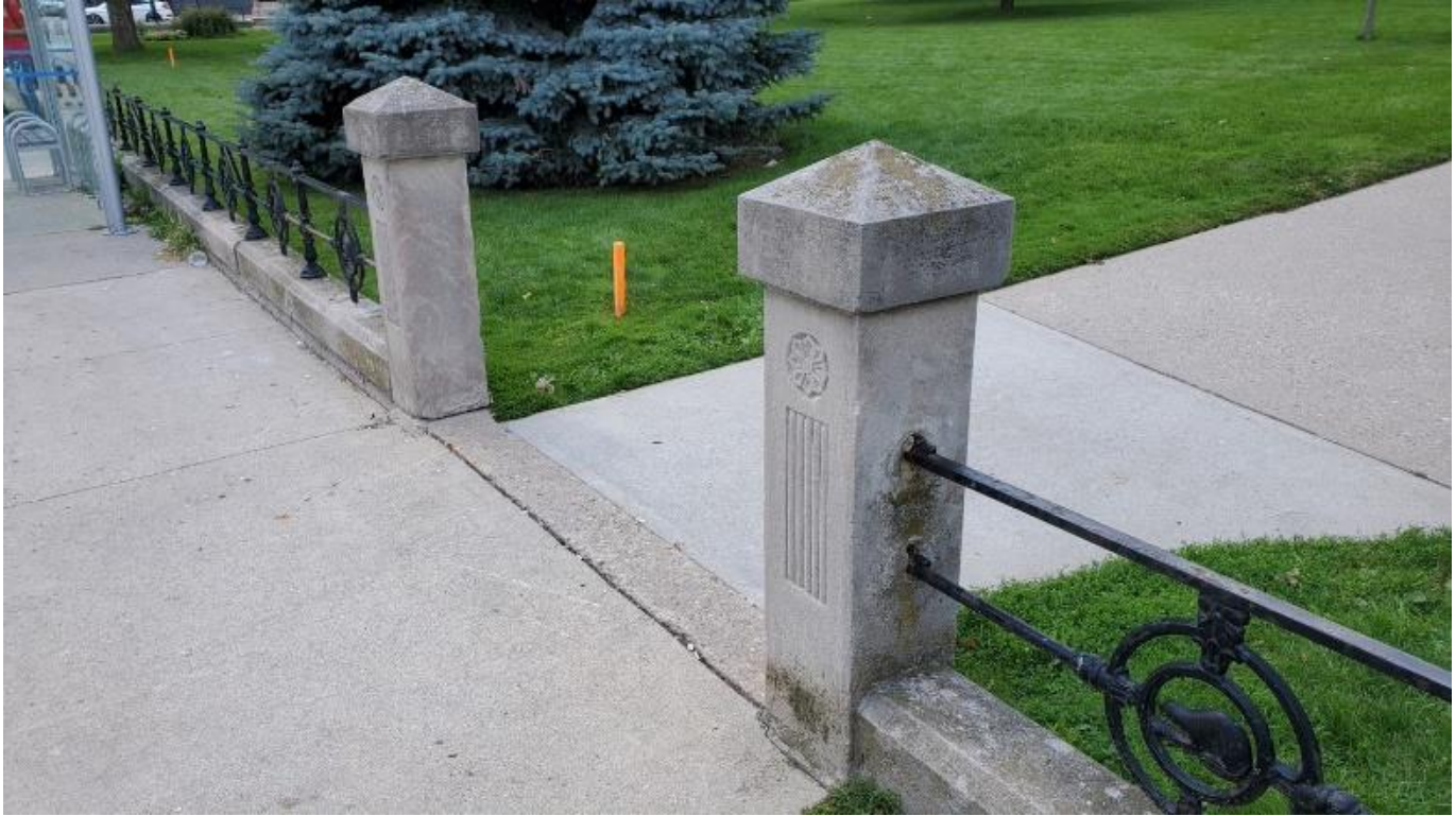
Photograph 14: The most western end posts on Queens Avenue proposed for relocation (AECOM, May 2021)
