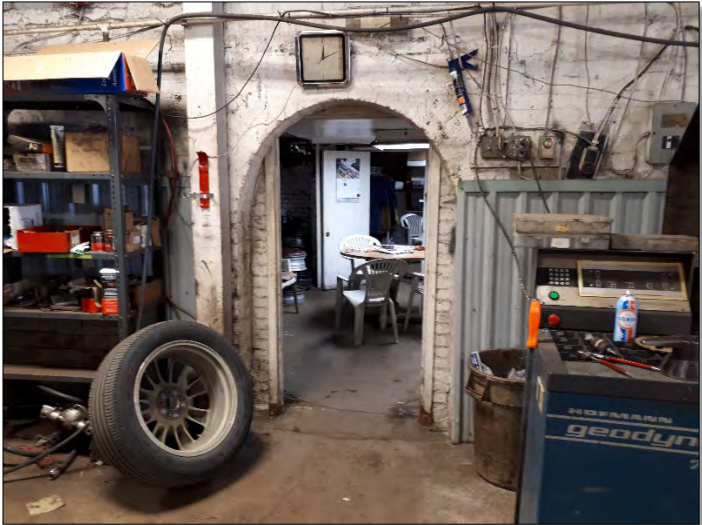
Figures 44 & 45: (above) Former window opening filled in by bricks on eastern elevation on exterior; (below) View of remaining Florentine arch between Building 'B' and Building 'C' (Source: MHBC, 2019).
