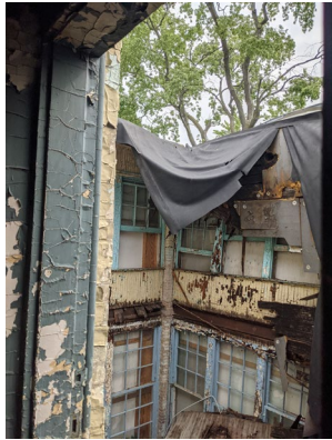
Photo 14: East porch collapse in June 2021
