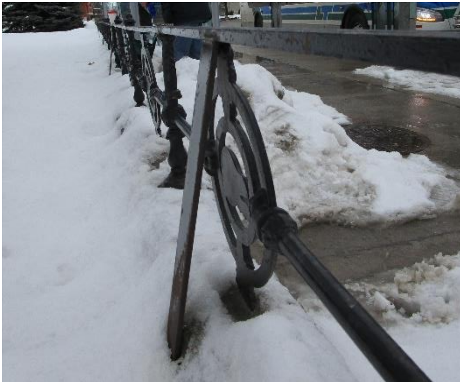
Photograph 40: Example of the back-support brace (AECOM, February 2021)
