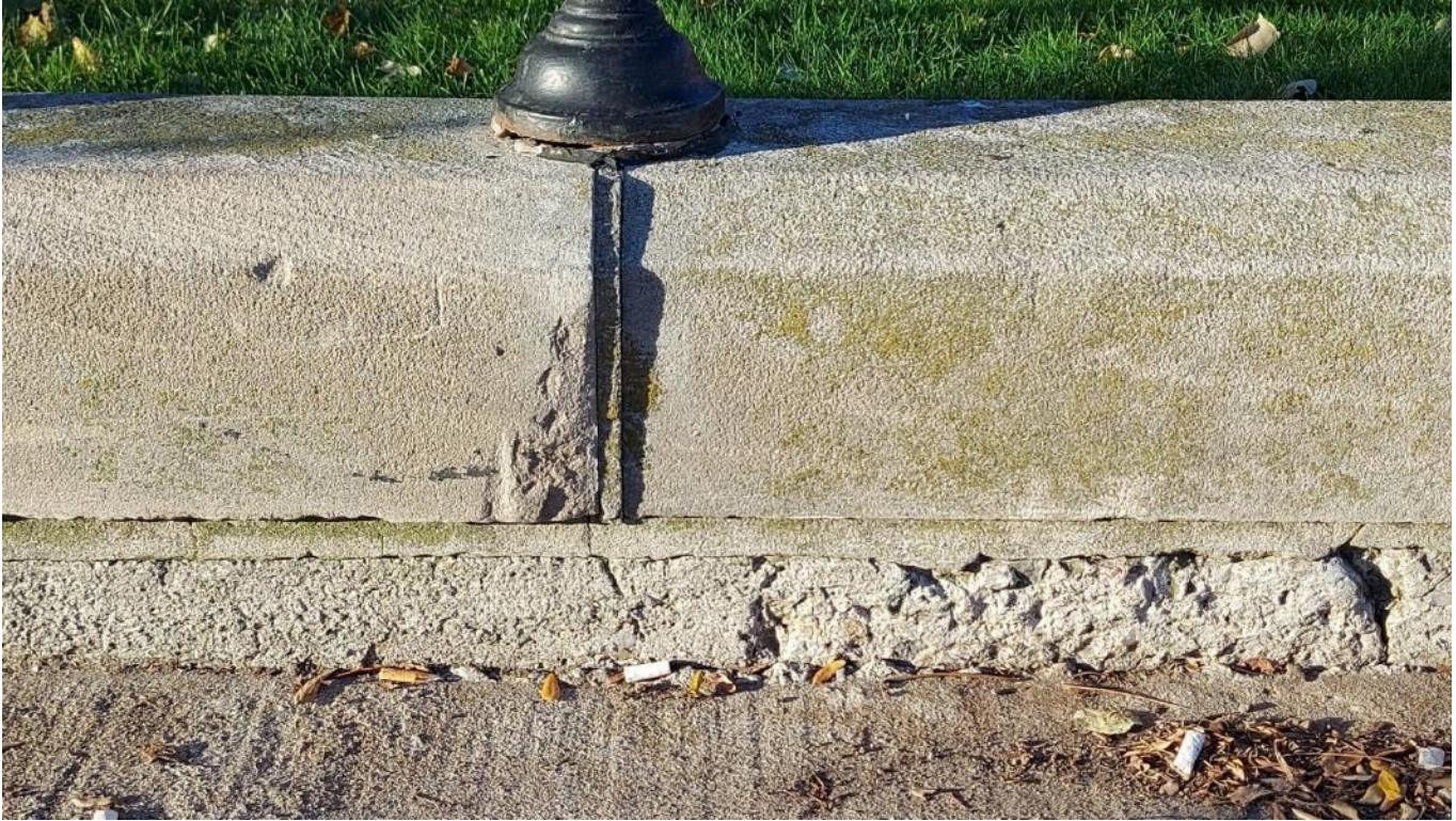
Photograph 24: View of mortar joint between cap stone and concrete foundation and mortar joint at each vertical rail post location (AECOM, November 2021)
