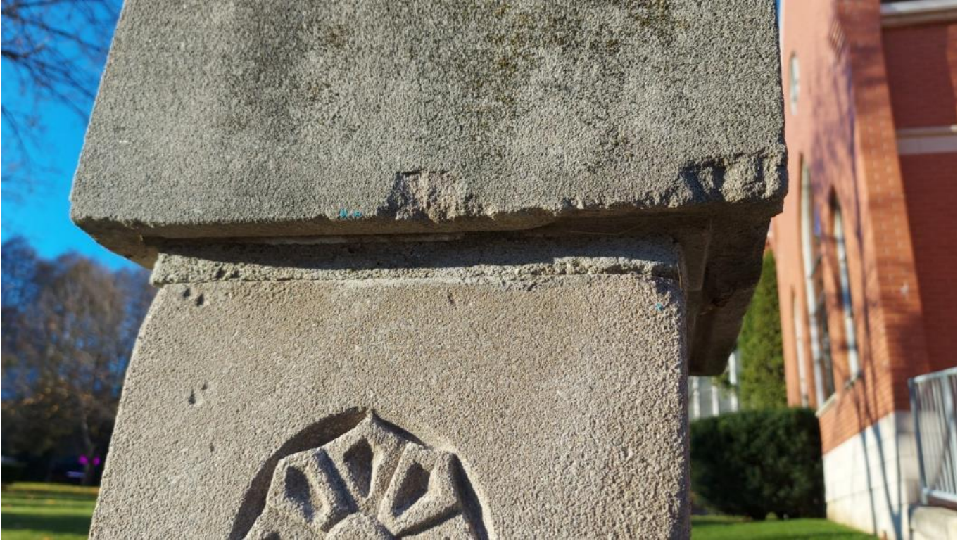
Photograph 16: View of the separate top cap of the end post with mortar layer with the end post (AECOM, November 2021)
