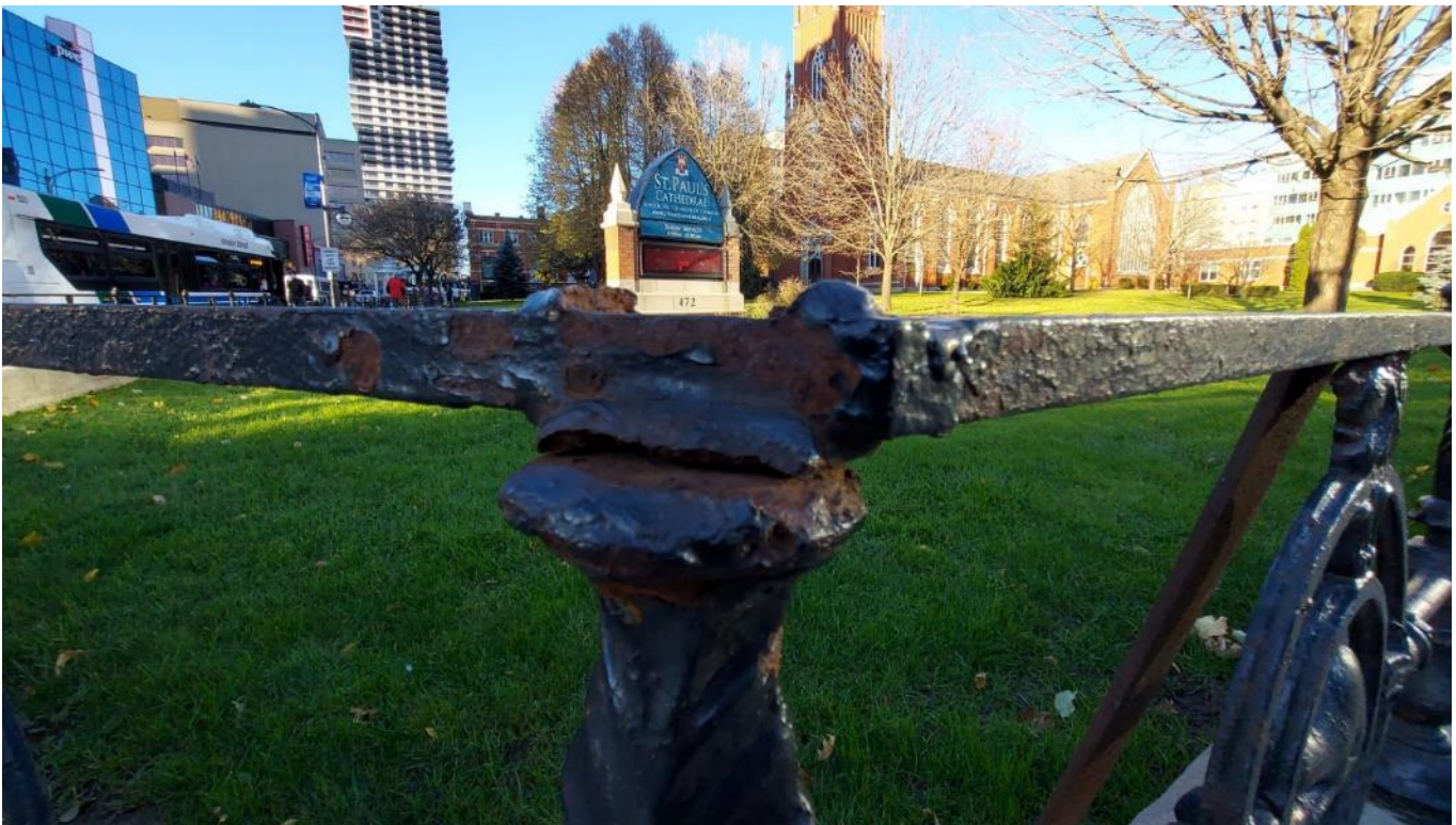
Photograph 34: Welding with cracks, illustrating piece by piece on-site construction of fence (AECOM, November 2021)
