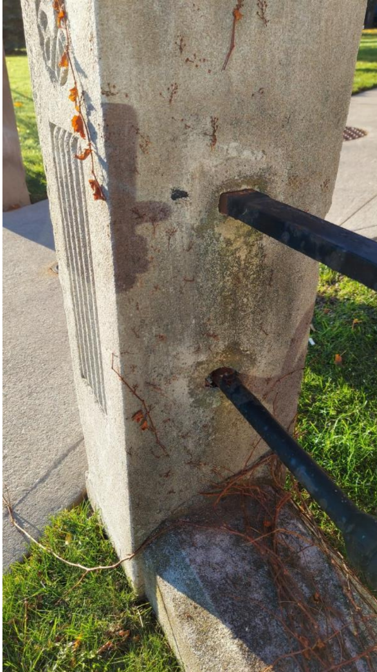
Photograph 19: Modified horizontal rails which place reinforcing steel bars into holes with mortar and welding of reinforcing steel bars to horizontal rails (AECOM, November 2021)
