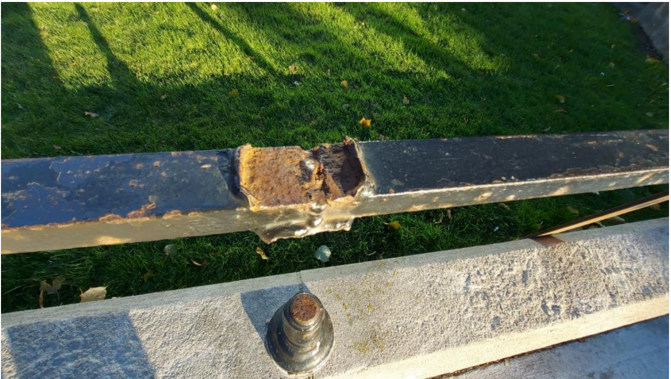
Photograph 32: The flat horizontal bar was placed over the vertical rail post and welded (AECOM, November 2021)
