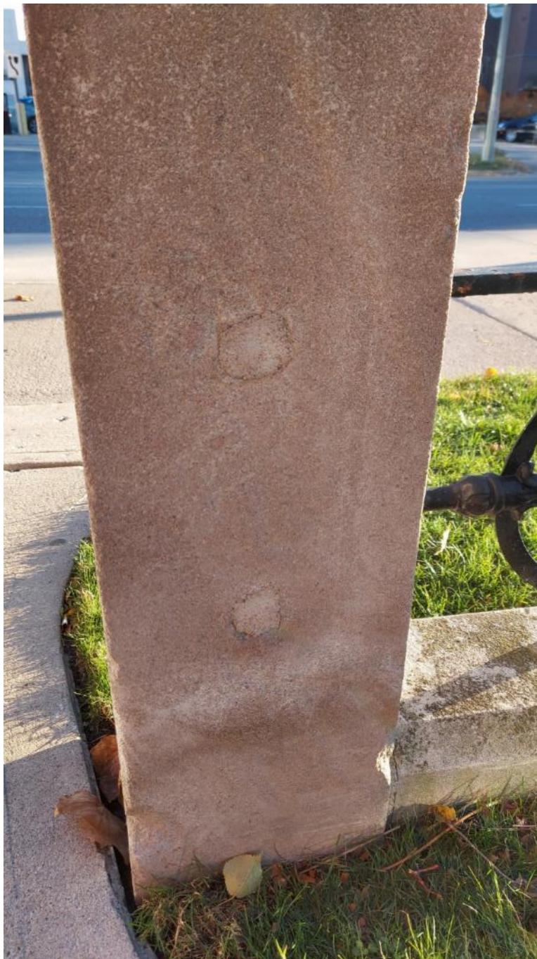
Photograph 20: Former holes in the end posts (for horizontal rail attachment) that were patched up, potentially indicating the end post was turned for repairs (AECOM, November 2021)
