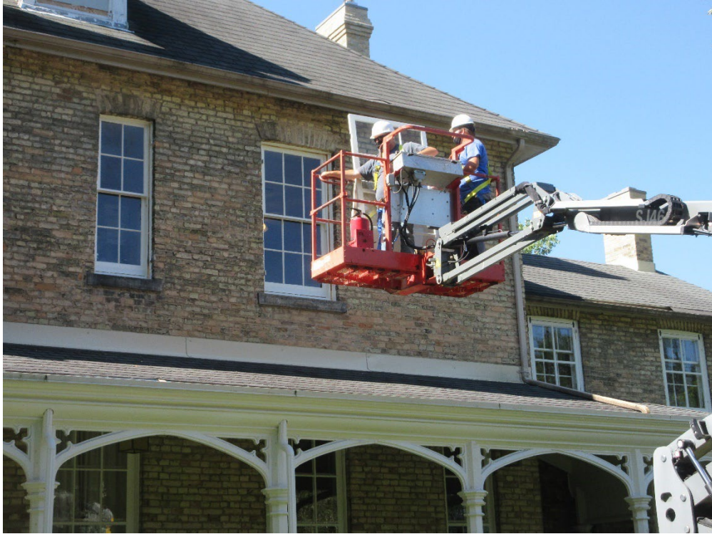
Image 2: Work underway to install the recently restored storm windows at Grosvenor Lodge.
