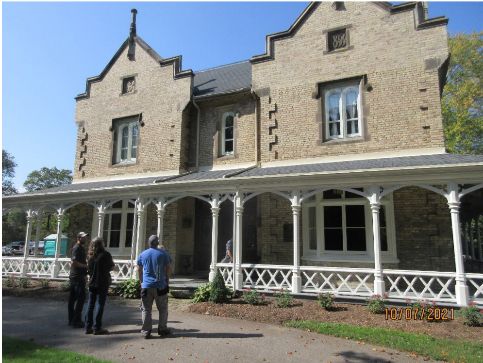
Image 3: Inspecting the new "Cathedral style" storm windows on the upper front windows at Grosvenor Lodge.
