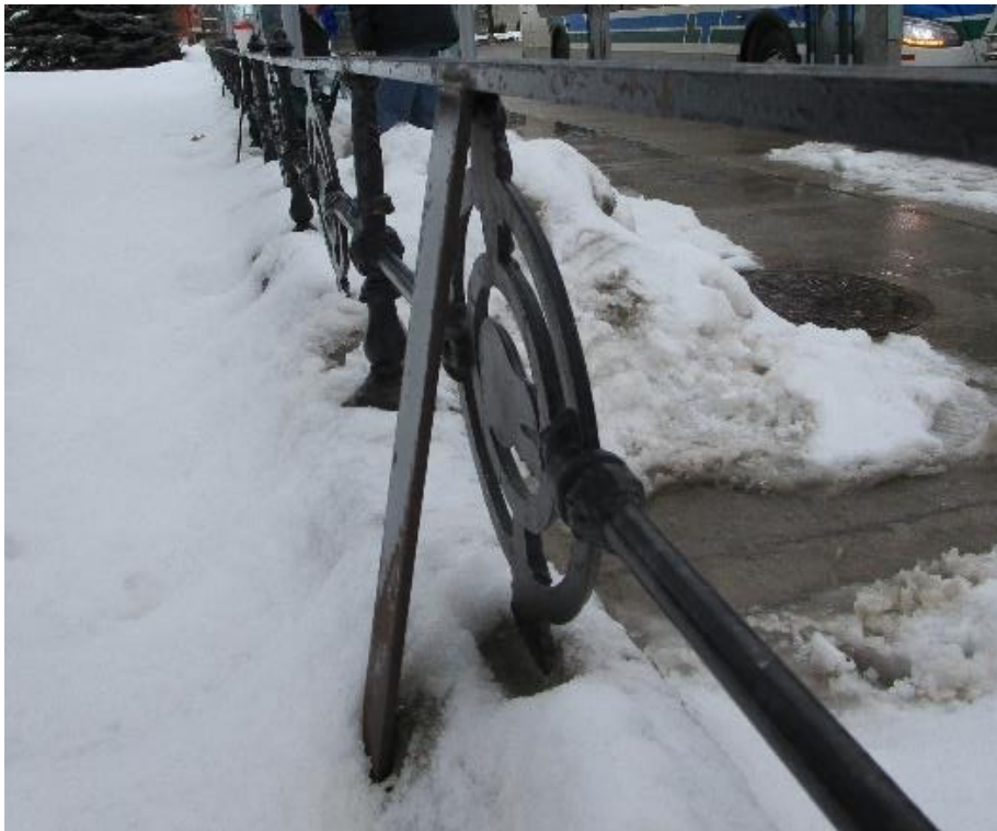
Photograph 40: Example of the back-support brace (AECOM, February 2021)
