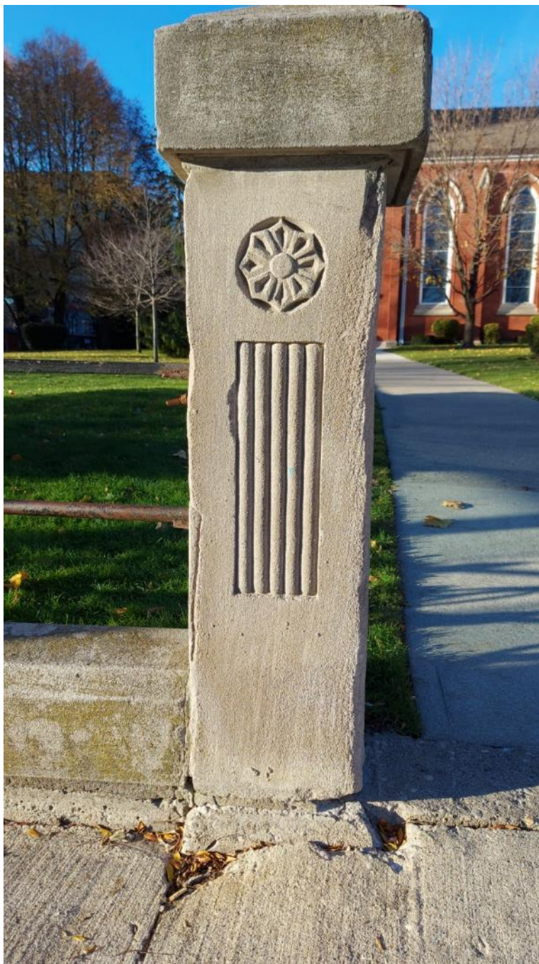
Photograph 15: End post proposed for relocation on Queens Avenue, showing signs of weathering and localized weathering on corners (AECOM, November 2021)
