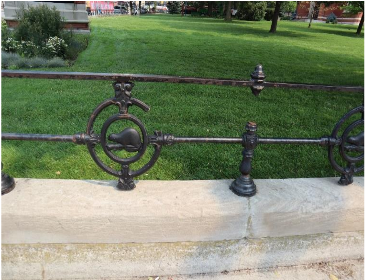
Photograph 30: Damaged section of the beaver fence on Richmond Street (AECOM, May 2021)
