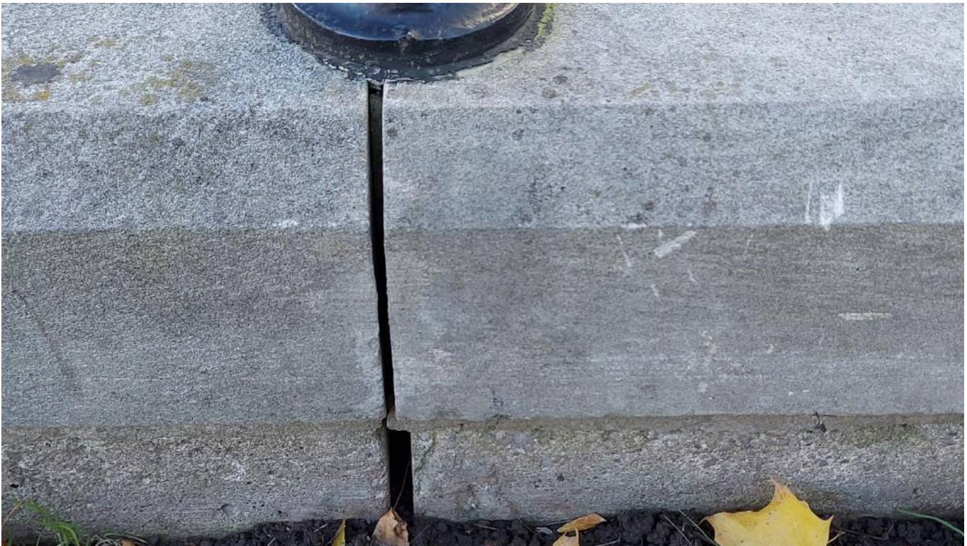
Photograph 25: Example of mortar joint missing and the cap stone cut and notched at each joint to accommodate the post attachment (AECOM, November 2021)
