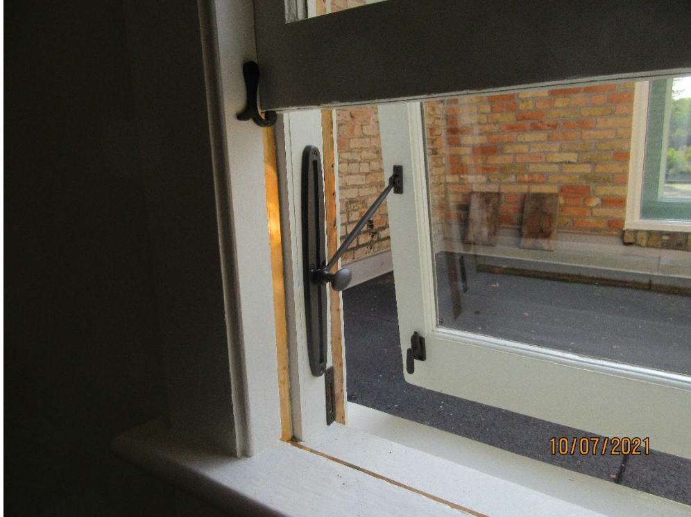
Image 4: Detail of the window opening hardware, security, and spring bronze weather stripping installed on one of the windows at Grosvenor Lodge.
