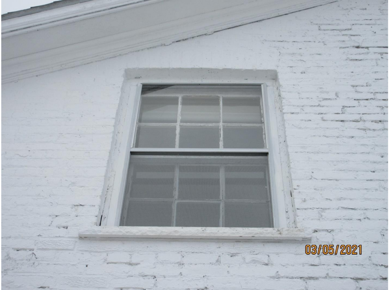
Image 16: Detail of the upper south window on the east elevation of the Clarke House. The sill was previously replaced.
