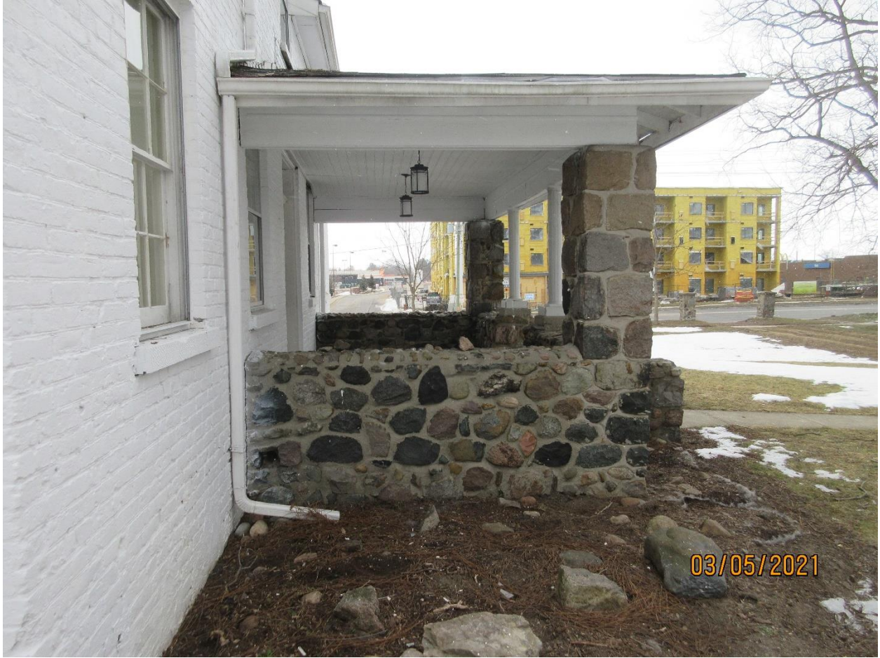
Image 14: Side view of the stone porch, showing the west elevation. Also showing the view towards Clarke Road.
