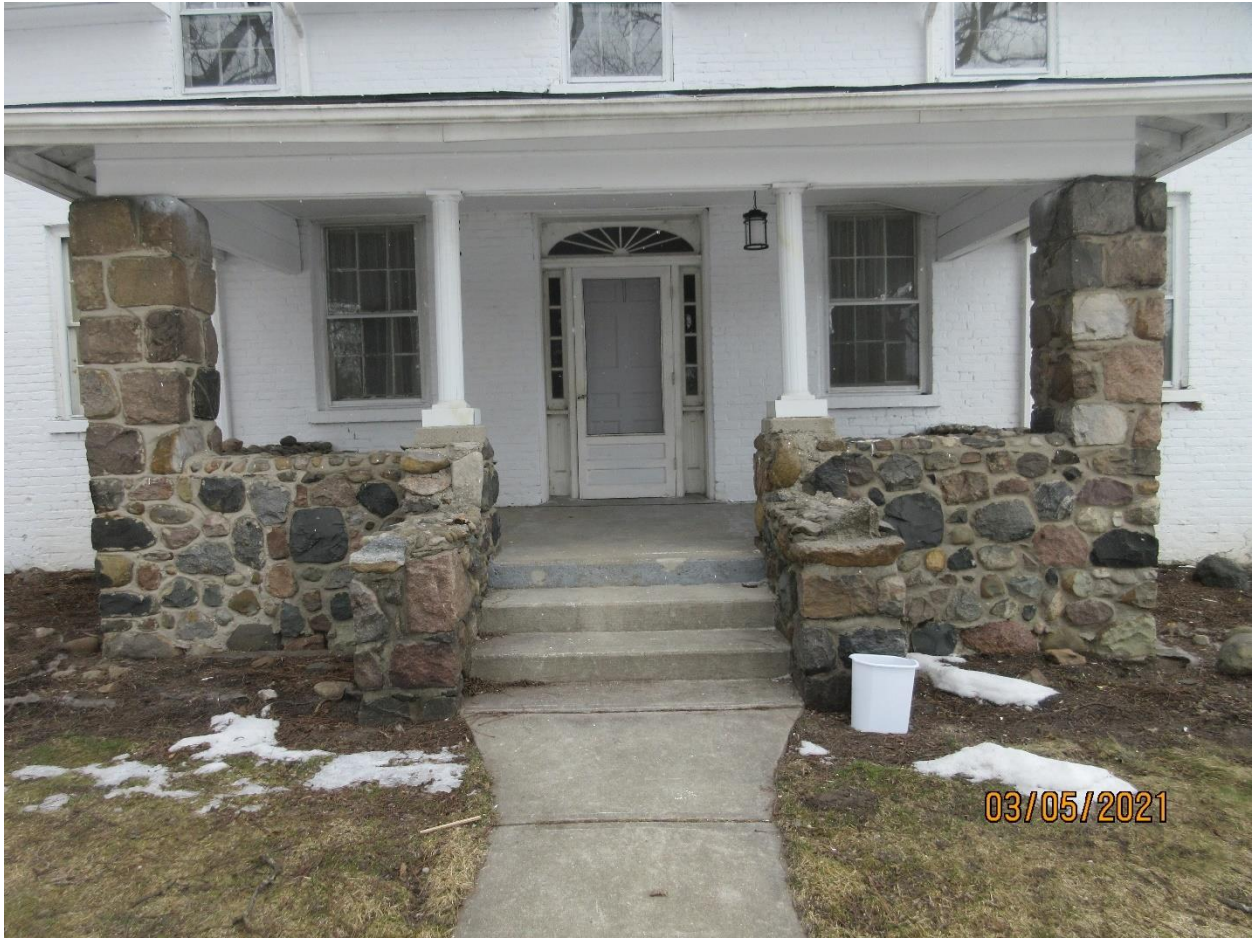
Image 13: Detail of the porch on the main (south) elevation of the Clarke House.
