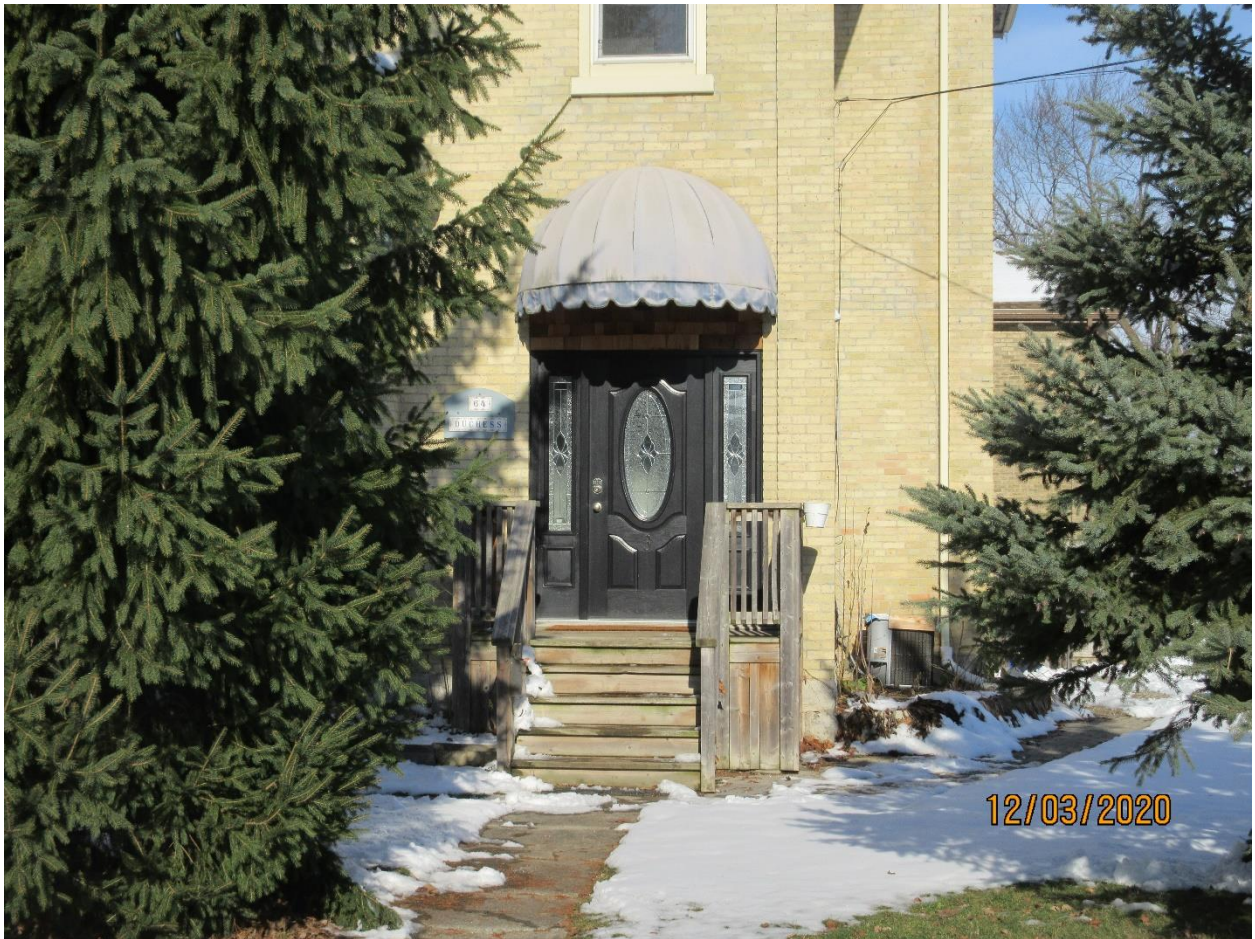
Image 4: Detail photograph showing the doorway that was installed without Heritage Alteration Permit approval.
