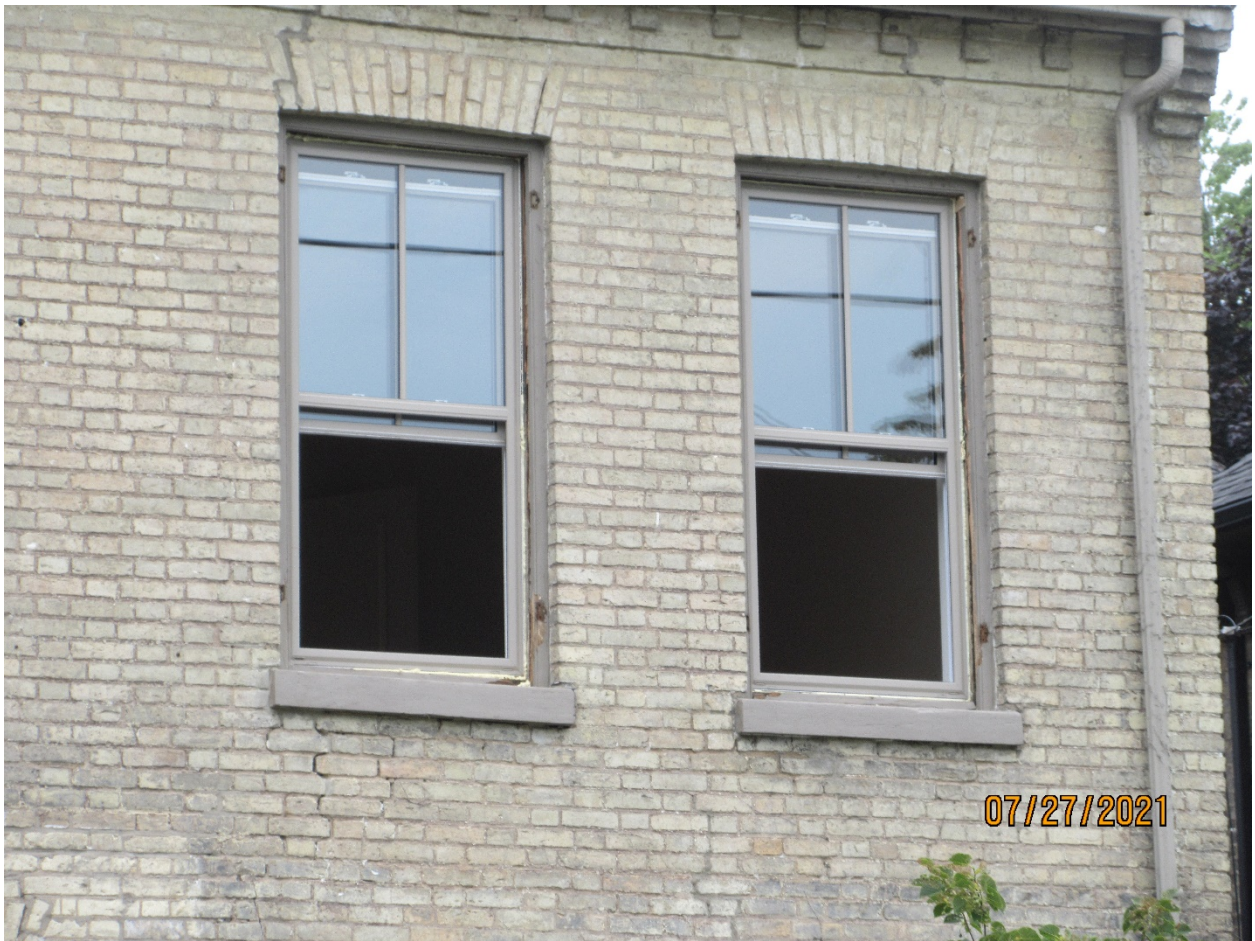
Image 6: Photograph showing the unapproved alterations to the windows at 468 Queens Avenue underway, July 2021.
