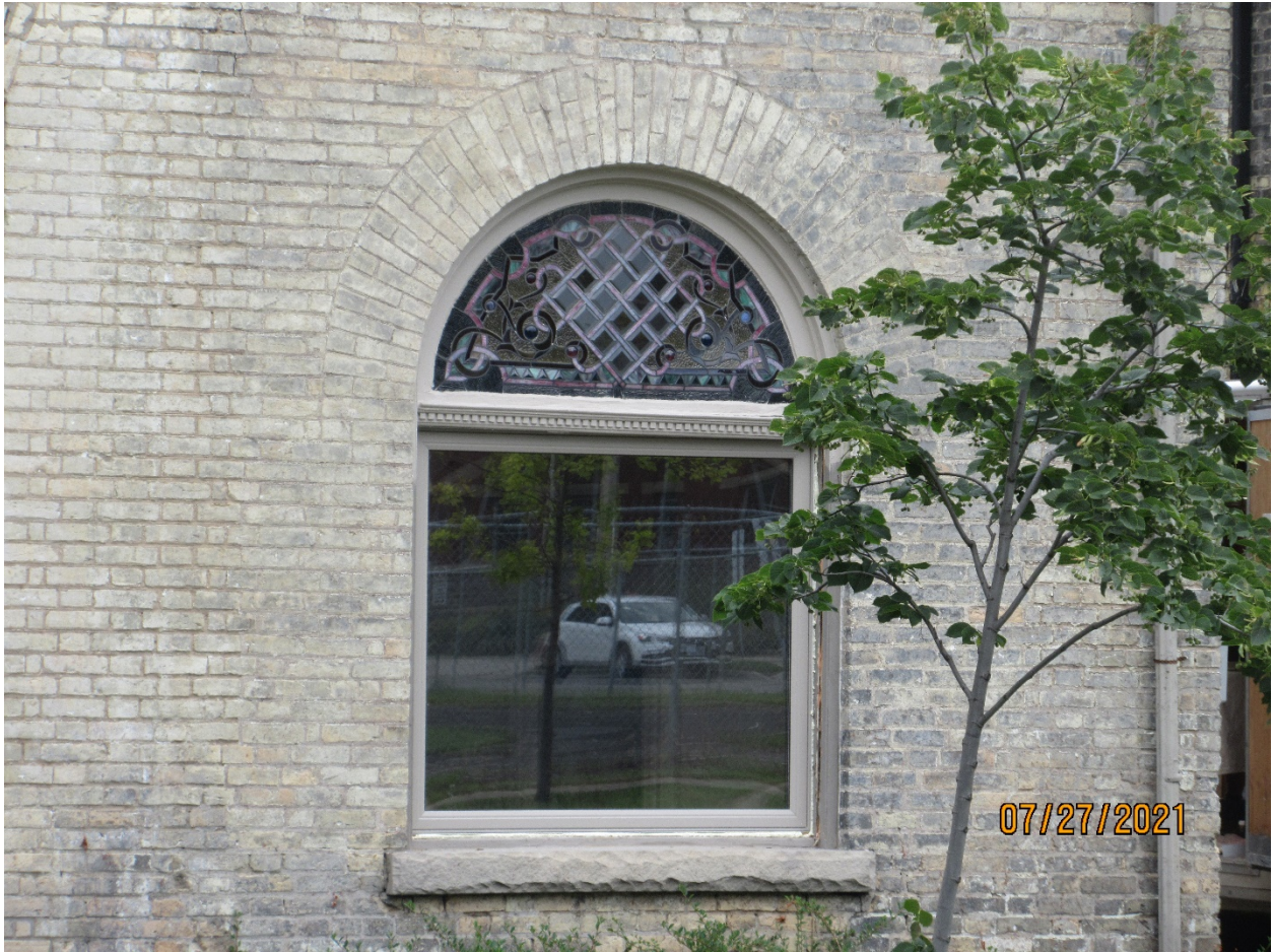
Image 5: Photograph showing the unapproved alterations to the windows at 468 Queens Avenue underway, July 2021.
