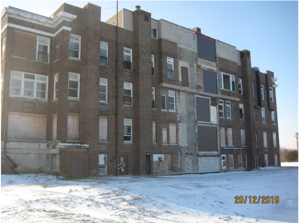
Image 9: Photograph showing the north (rear) facade of the War Memorial Children's Hospital.
