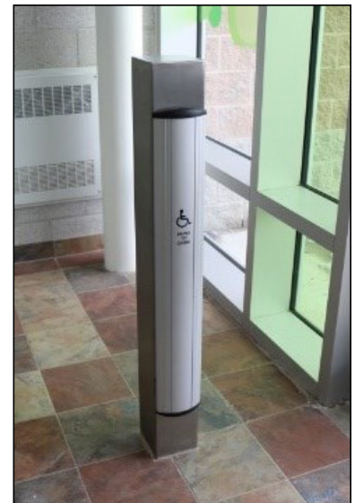
Example of large vertical extended power door operator control.
