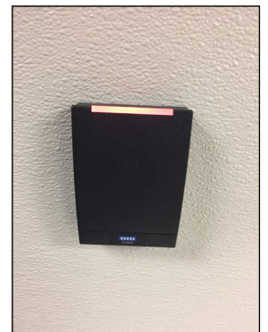
Example of proximity card reader system with visual indicator, City of London.
