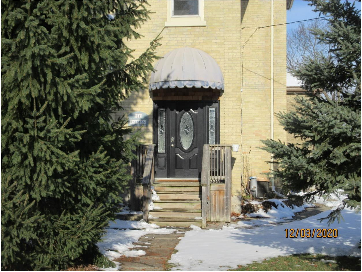
Image 4: Detail photograph showing the doorway that was installed without Heritage Alteration Permit approval.
