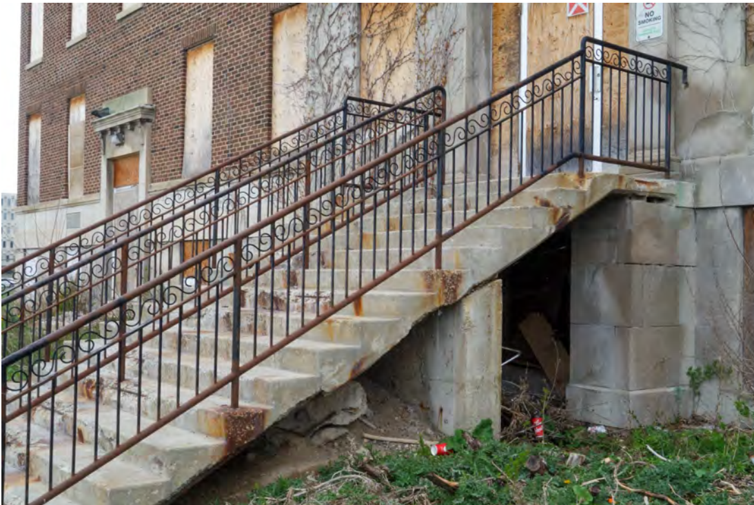
MAIN ELEVATION – STAIRS TO THE FRONT ENTRANCE – the metal railings are in fair condition
