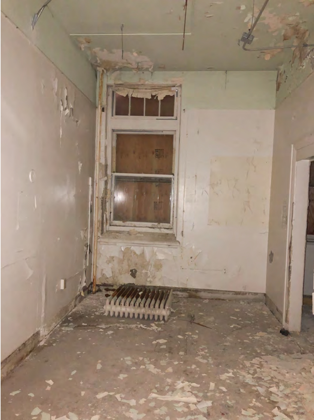
WINDOWS – 1 over 1 wood sash windows with 4-pane transom above are in poor condition
