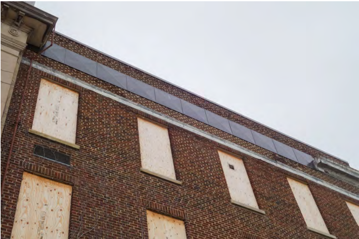
MAIN ELEVATION – missing section of the original cornice
