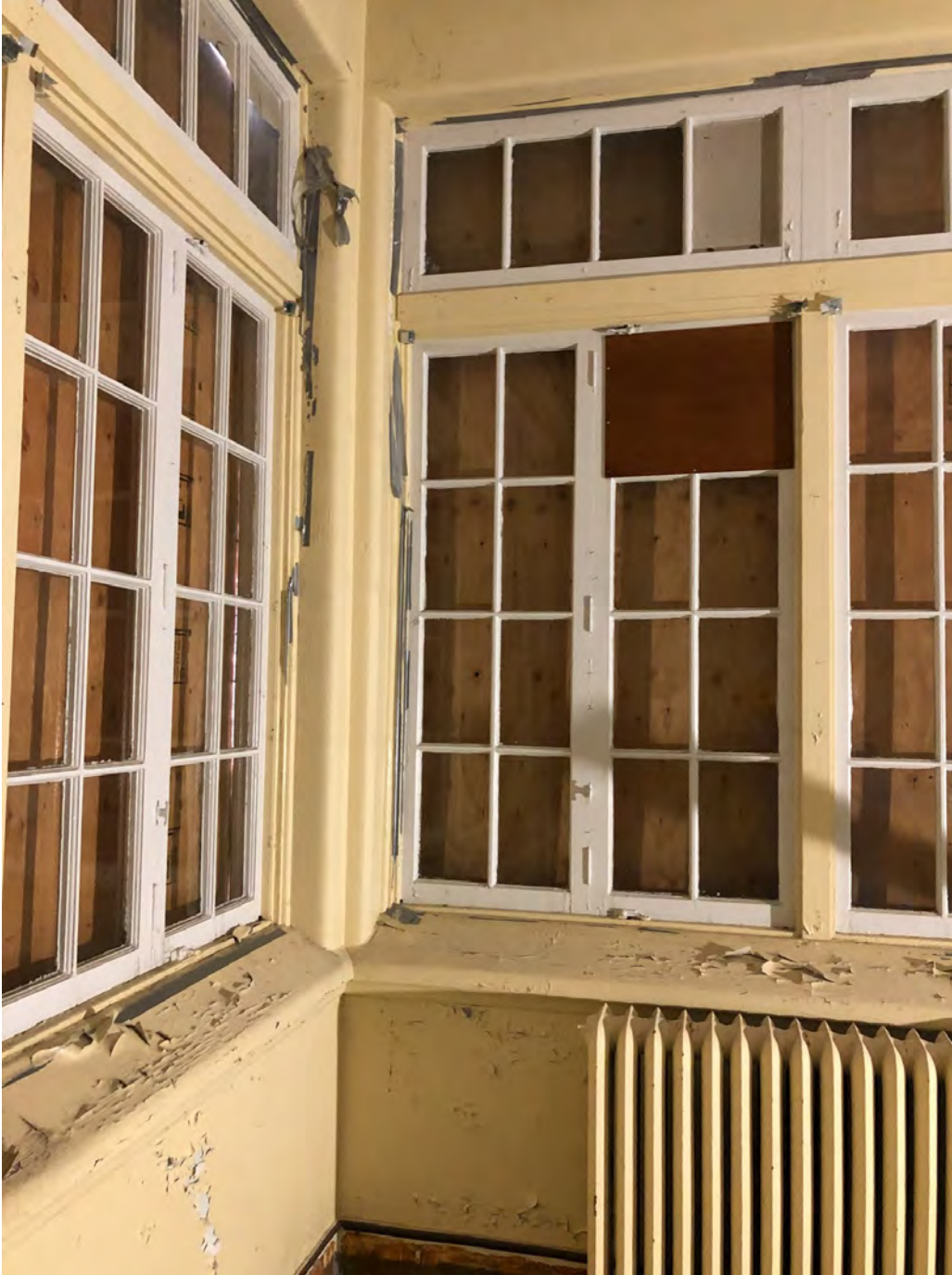
SUNROOM – wood casement windows in the sunrooms are in fair to poor condition
