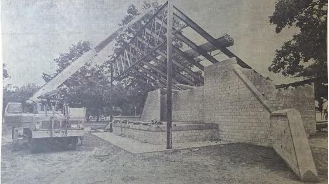
Image 1: Photograph showing the construction of the park stage at Queen's Park, as shown in the London Free Press, September 3, 1971.
