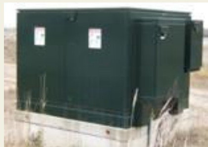
Pad mounted switchgear
