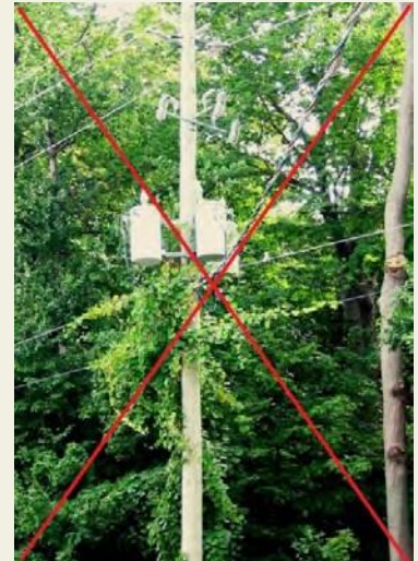
Pole growth contacting electrical equipment & powerlines
