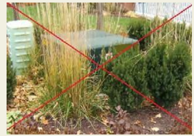
Obstruction around a transformer
