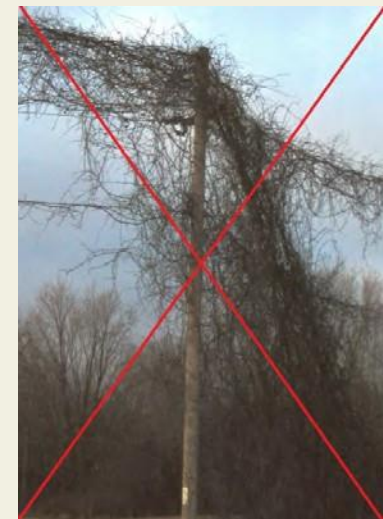
Guy-wire growth contacting electrical equipment & powerlines
