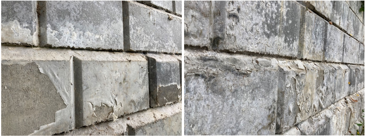
Figure 1: Peeling and degraded anti-graffiti coating from Phase 1 and Phase 2
