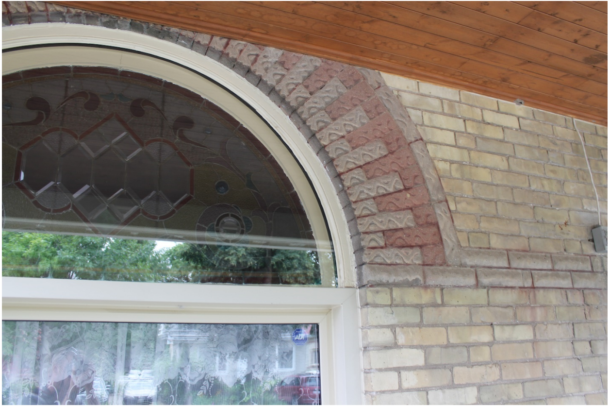
Image 9: Photograph showing detail of the voussoirs, string course, and arched stained glass window.
