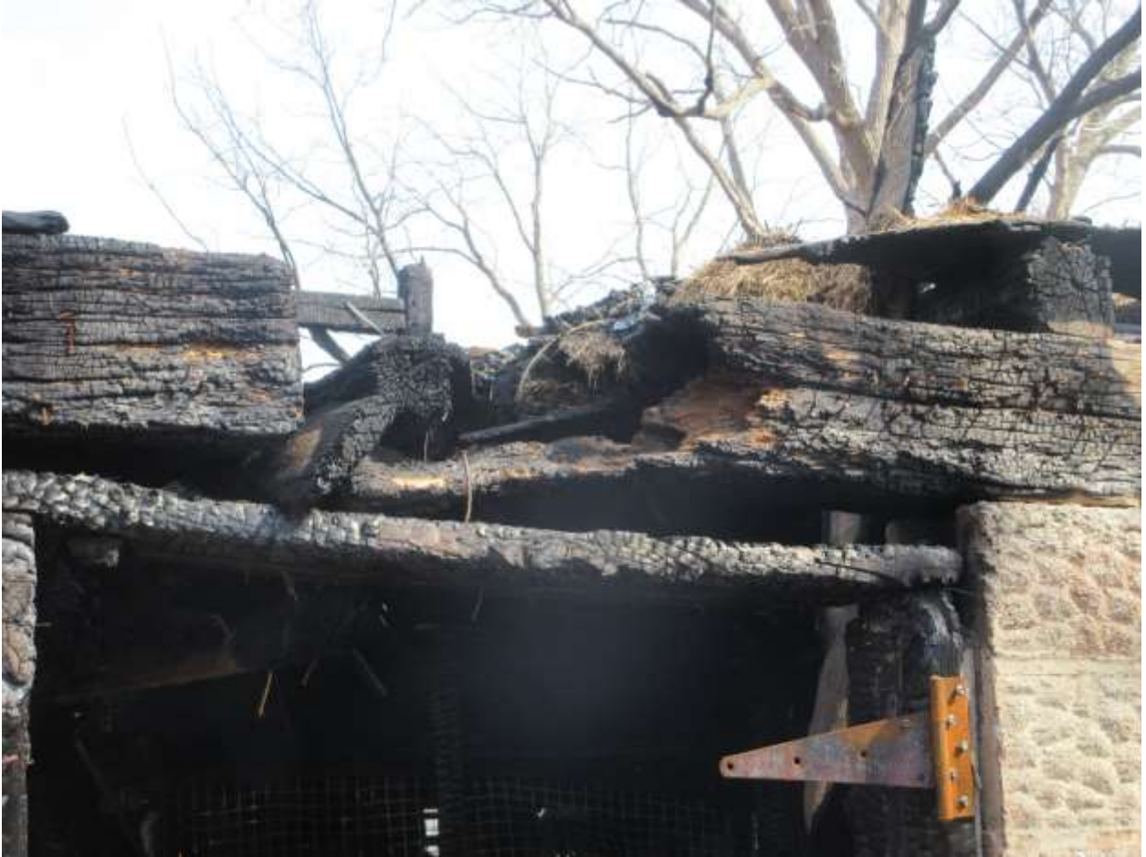
Image 15: Detail of the damage caused by fire on February 16, 2018 to the south barn located at 2154 Richmond Street.
