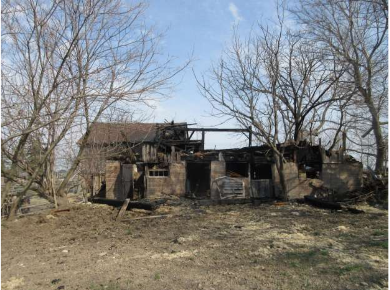
Image 13: View of the south façades of the barns located at 2154 Richmond Street. Note the extent of the damage to the south barn.
