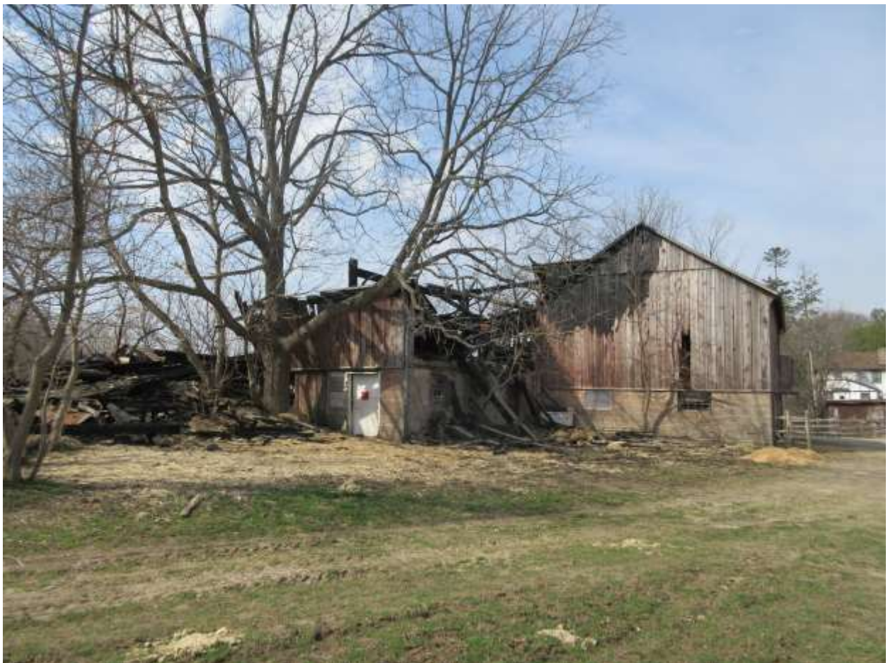
Image 12: View of the east façades of the barns located at 2154 Richmond Street. Note the extent of the damage to the south barn.
