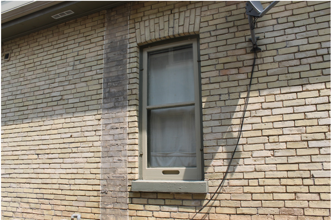
Image 12: Photograph showing double-hung wood window on the west facade of the house, with brick voussoirs and wood sill. Note, the "ghosting" of a former chimney is visible on this wall.
