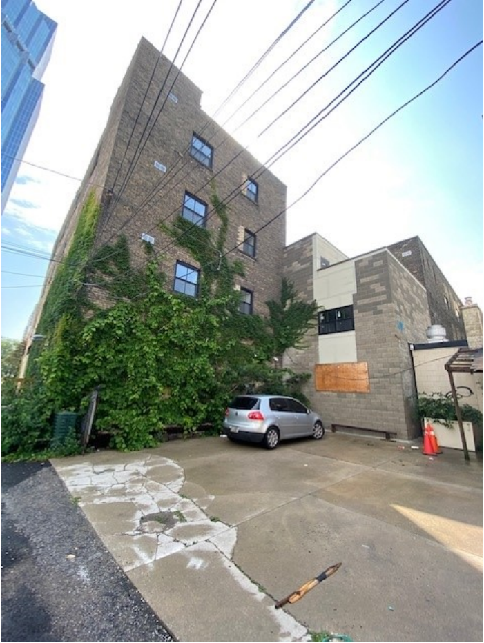
Image 4: View of rear portion of existing building facing parking lot and new addition, seen with unfinished cladding (July 29, 2021)
