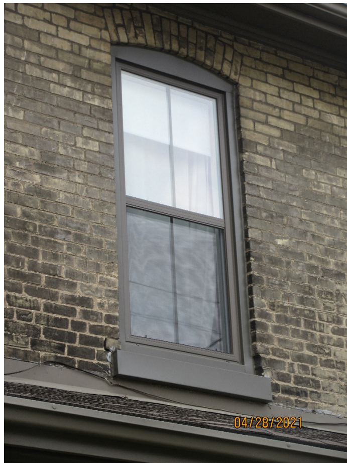
Image 10: Detail photograph of the replacement windows, showing the faux grille (muntin) of the replacement window. The faux grille is only between the glass panes and fails to accurately replicate any historic details.
