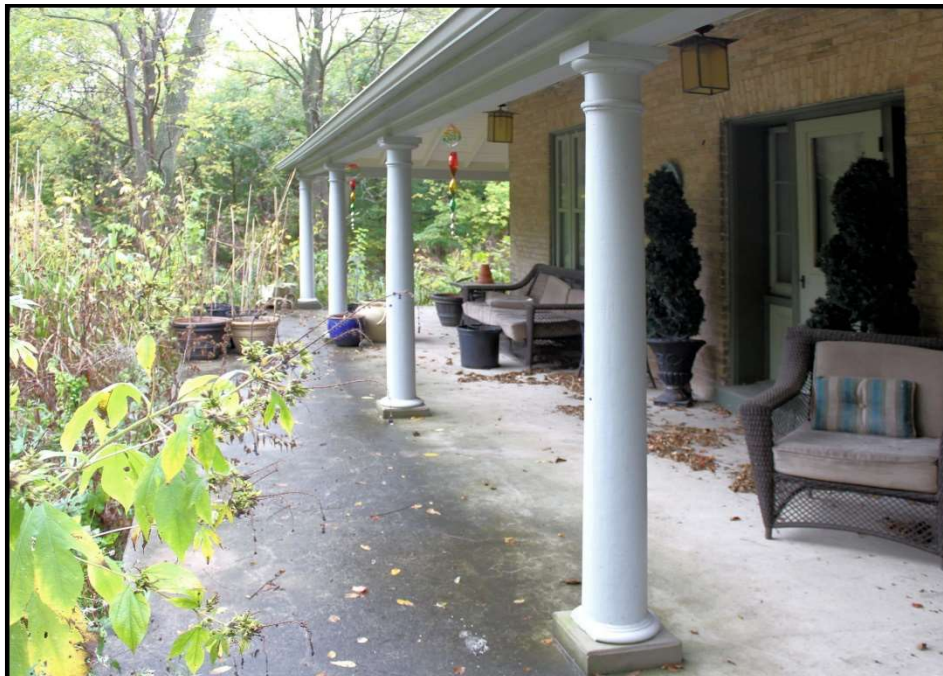
17. View looking northward and into the front cottage verandah. The front entry is to the right.
