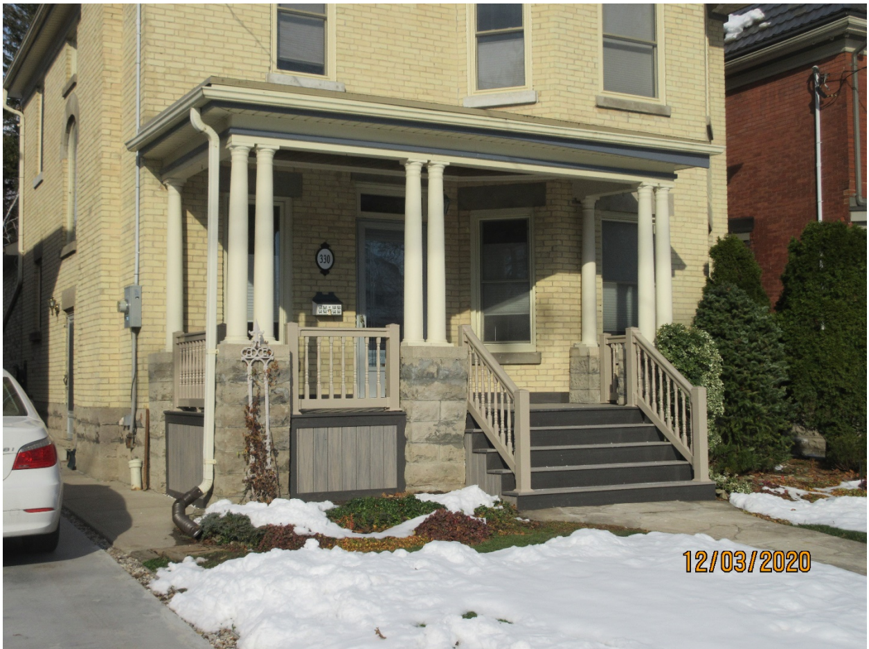
Image 4: Detail photograph of the porch of the property at 330 St. James Street showing the alterations completed to the porch without Heritage Alteration Permit approval.
