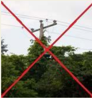
Overgrown vines around electrical equipment
