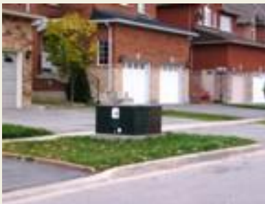
Pad mounted transformer
