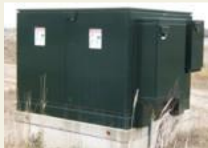
Pad mounted switchgear
