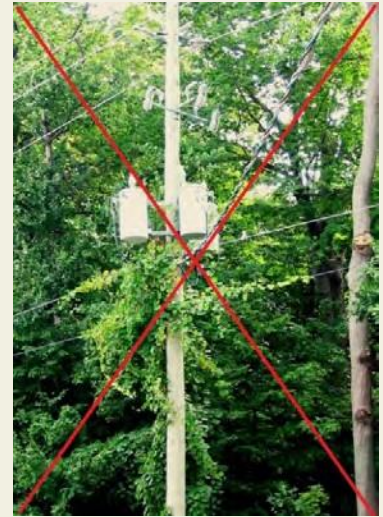
Pole growth contacting electrical equipment & powerlines
