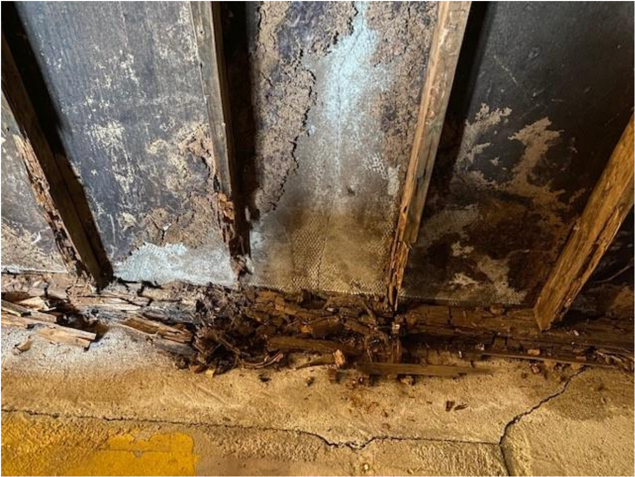
Image 5: Interior view of detached garage showing degradation of wood sill and wall studs (April 22, 2021)
