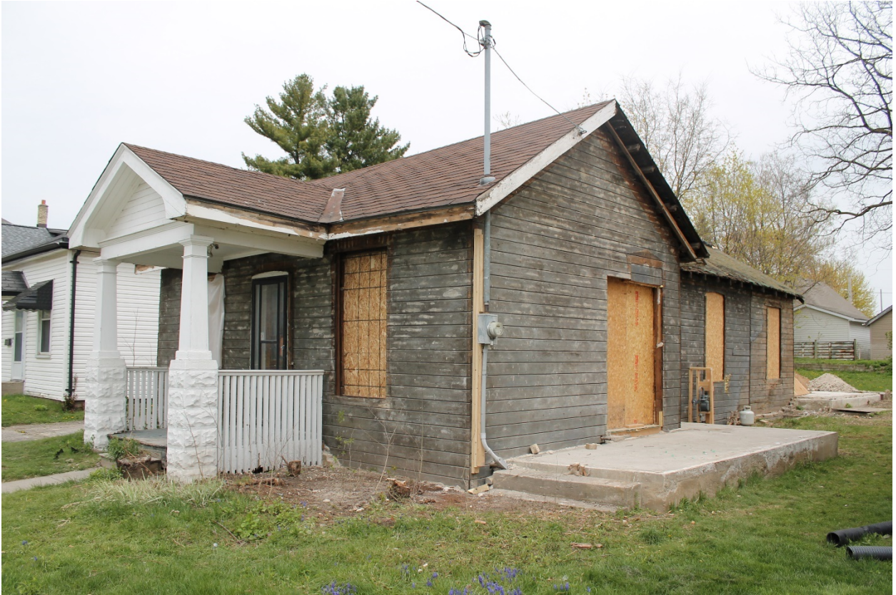
Image 8: Photograph showing the west (front) façade and the south façade of the dwelling. The rear addition is visible, 2021.
