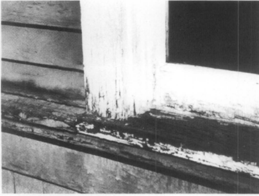
Figure 3. Deterioration of poorly maintained windows usually begins on horizontal surfaces and at joints where water can collect and saturate the wood. The problem areas are clearly indicated by paint failure due to moisture. Photo: Baird M. Smith, AIA
