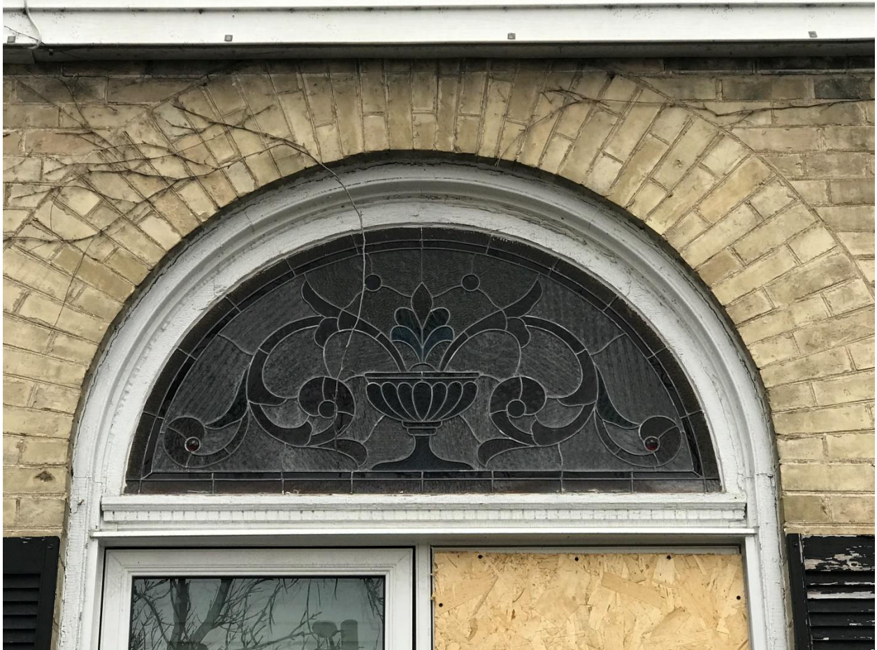
Image 3: Detail photograph of the arched transom over the front window with stained glass (April 5, 2021). The stained glass has an urn and floral motif, typical of the period of construction for the subject property. Salvage of this window in advance of demolish is strongly encouraged.
