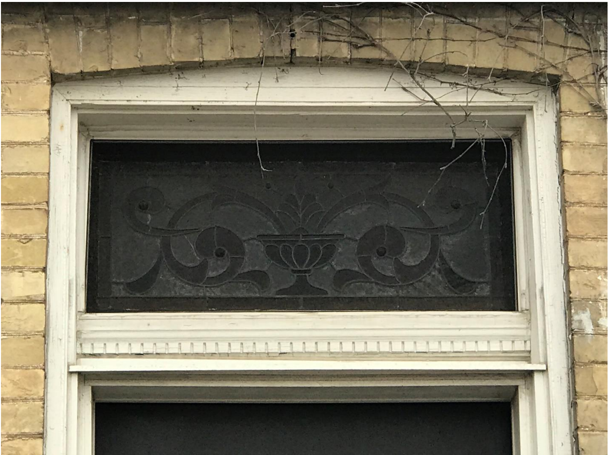
Image 4: Detail photograph of the rectangular transom over the front doorway with stained glass (April 5, 2021). The stained glass has an urn and floral motif, typical of the period of construction for the subject property. Salvage of this window in advance of demolish is strongly encouraged.
