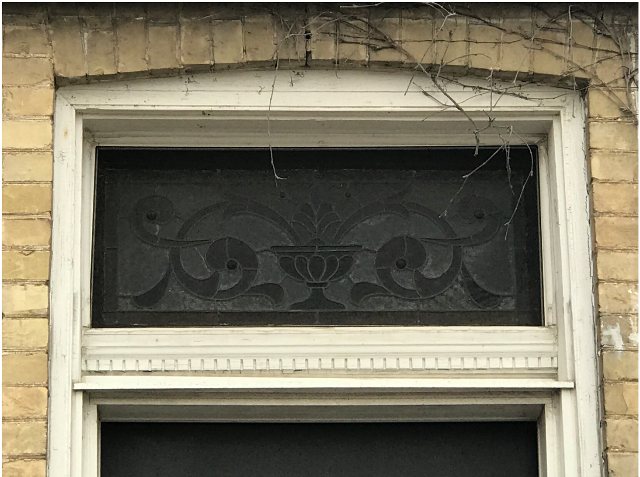
Image 4: Detail photograph of the rectangular transom over the front doorway with stained glass (April 5, 2021). The stained glass has an urn and floral motif, typical of the period of construction for the subject property. Salvage of this window in advance of demolish is strongly encouraged.
