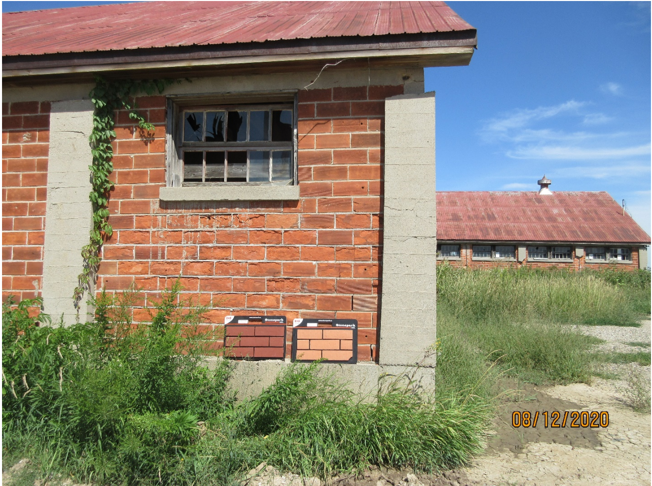
Image 2: Photograph showing two samples of a proposed veneer cladding, seeking a suitable colour match. The sample on the left has been selected as the preferred veneer cladding.
