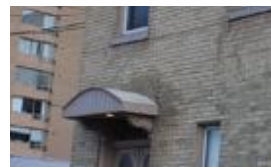
18. The porch roof of the doorway is altered but appears to adhere to the line of a previous porch and is still supported by original brackets
