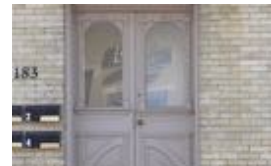
15. The principal doorway on the front façade has an original double-leafed door, which is carved, pierced and well decorated
