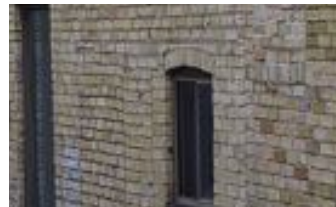
12. Door and window openings on the west and east side have been bricked over as the building's function changed
