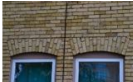
10. The fenestration is symmetrical within the irregular profile; with most of the principal windows being segmental-arched topped with brick voussoirs
