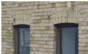
10. Most of the original windows are segmental arch openings topped with brick voussoirs
