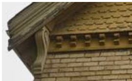
14. The brackets and modillions adhere to a single character throughout the whole structure
