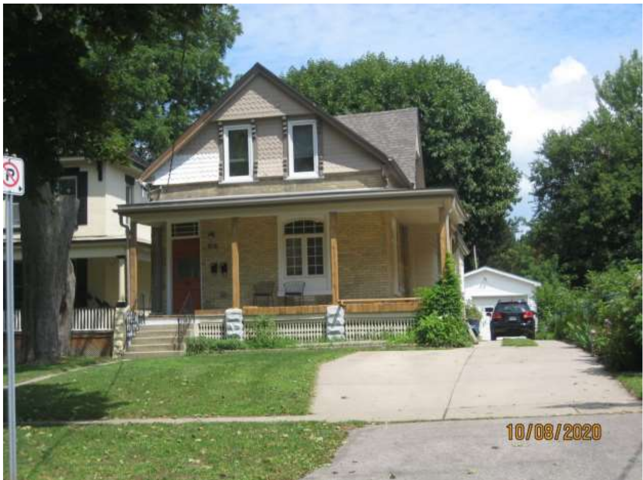
Image 4: Photograph showing unapproved alterations underway at 562 Maitland Street in August 2020. Note, the porch floor has been installed, and six 6" x 6" structural posts have been installed to support the porch roof.
