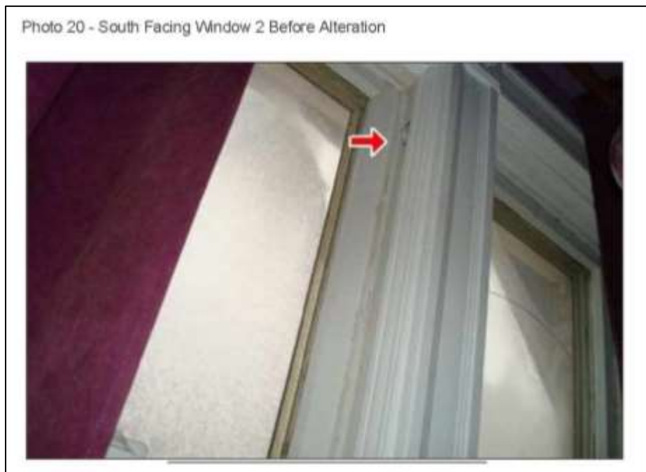
Image 12: Image of the south facing window 2 before alteration (interior), submitted as part of the Heritage Alteration Permit application. Arrow on image identifying missing sash cord.
