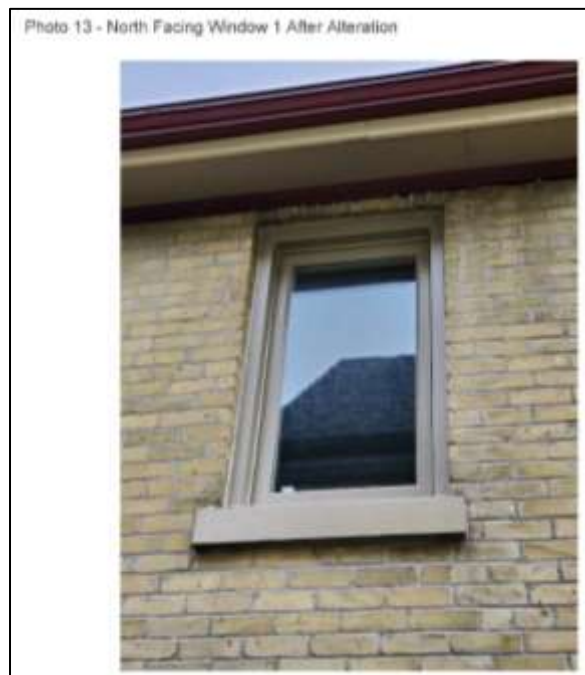
Image 9: Image of the north facing window 1 after alteration (exterior), submitted as part of the Heritage Alteration Permit application.
