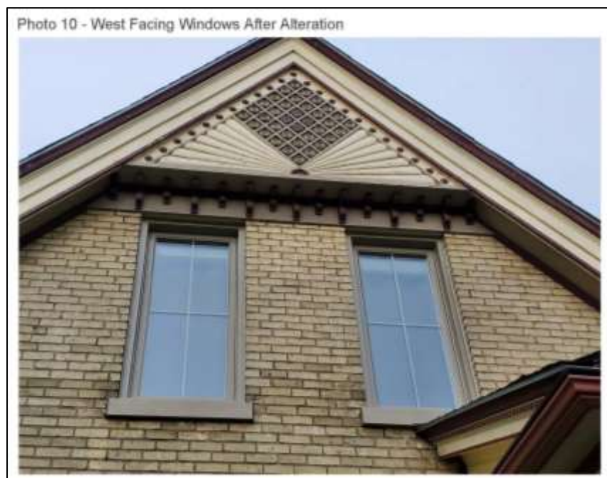
Image 7: Detail image of the upper windows on the west façade after their replacement, submitted as part of the Heritage Alteration Permit application.
