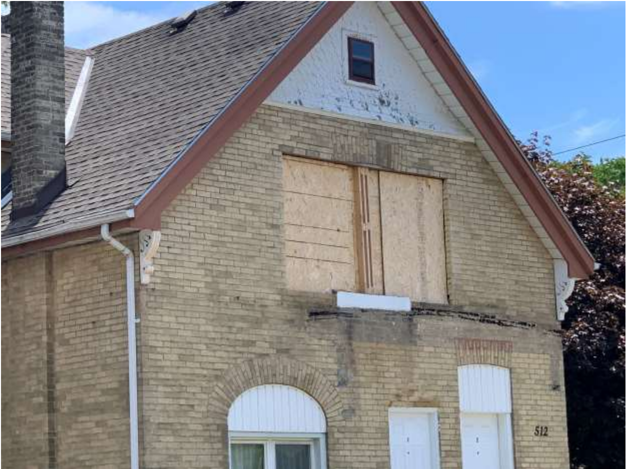
Image 5: Photograph submitted as a part of the Heritage Alteration Permit application showing unapproved alterations underway.
