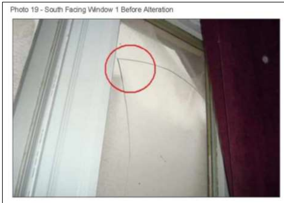
Image 11: Image of the south facing window 1 before alteration (interior), submitted as part of the Heritage Alteration Permit application. Circle on image identifying crack in the glass pane.
