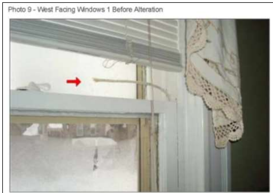
Image 6: Image, submitted as part of the Heritage Alteration Permit application, showing a cut or broken sash cord.
