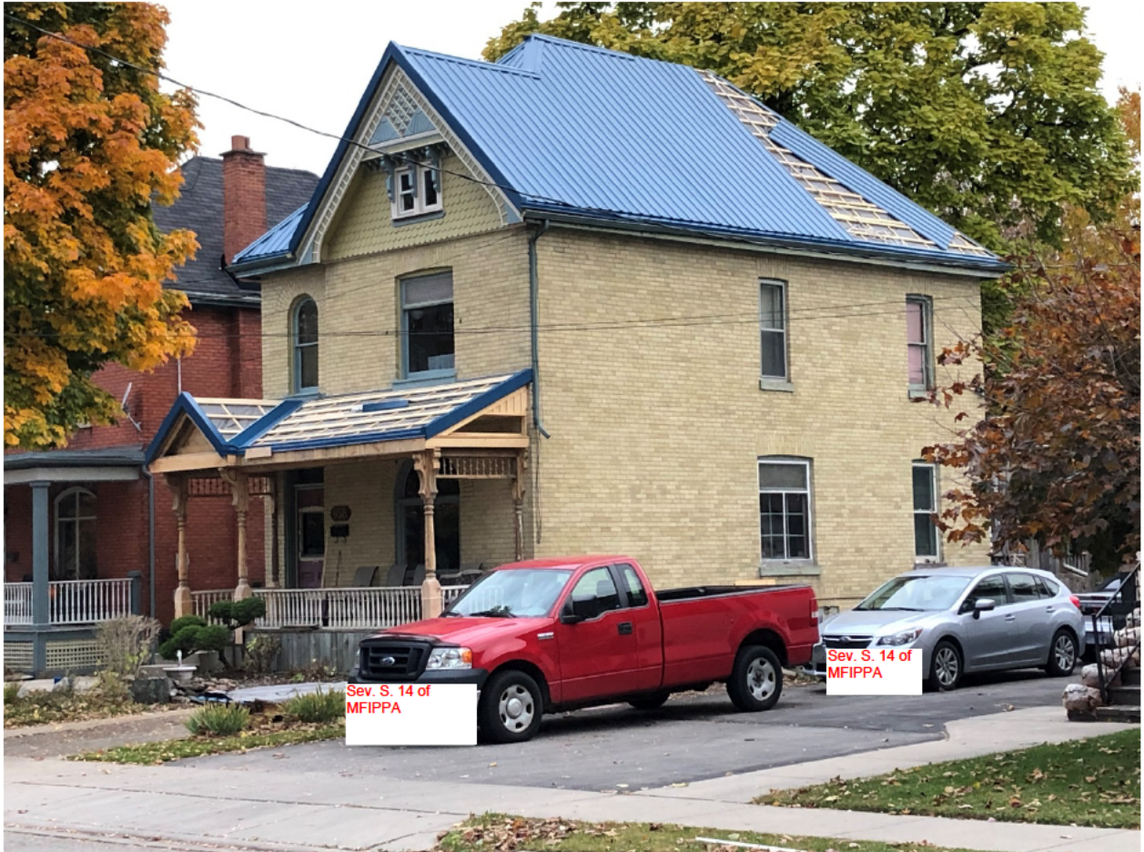
Image 3: Photograph showing unapproved roof material alterations being undertaken in October 2019
