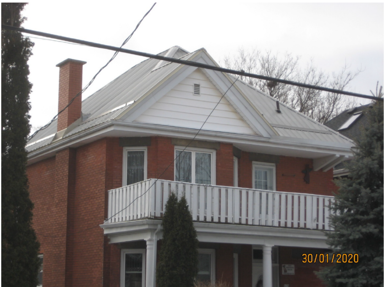
Image 14: Photograph showing unapproved sheet metal roofing material alteration at 825 Lorne Avenue in January 2020
