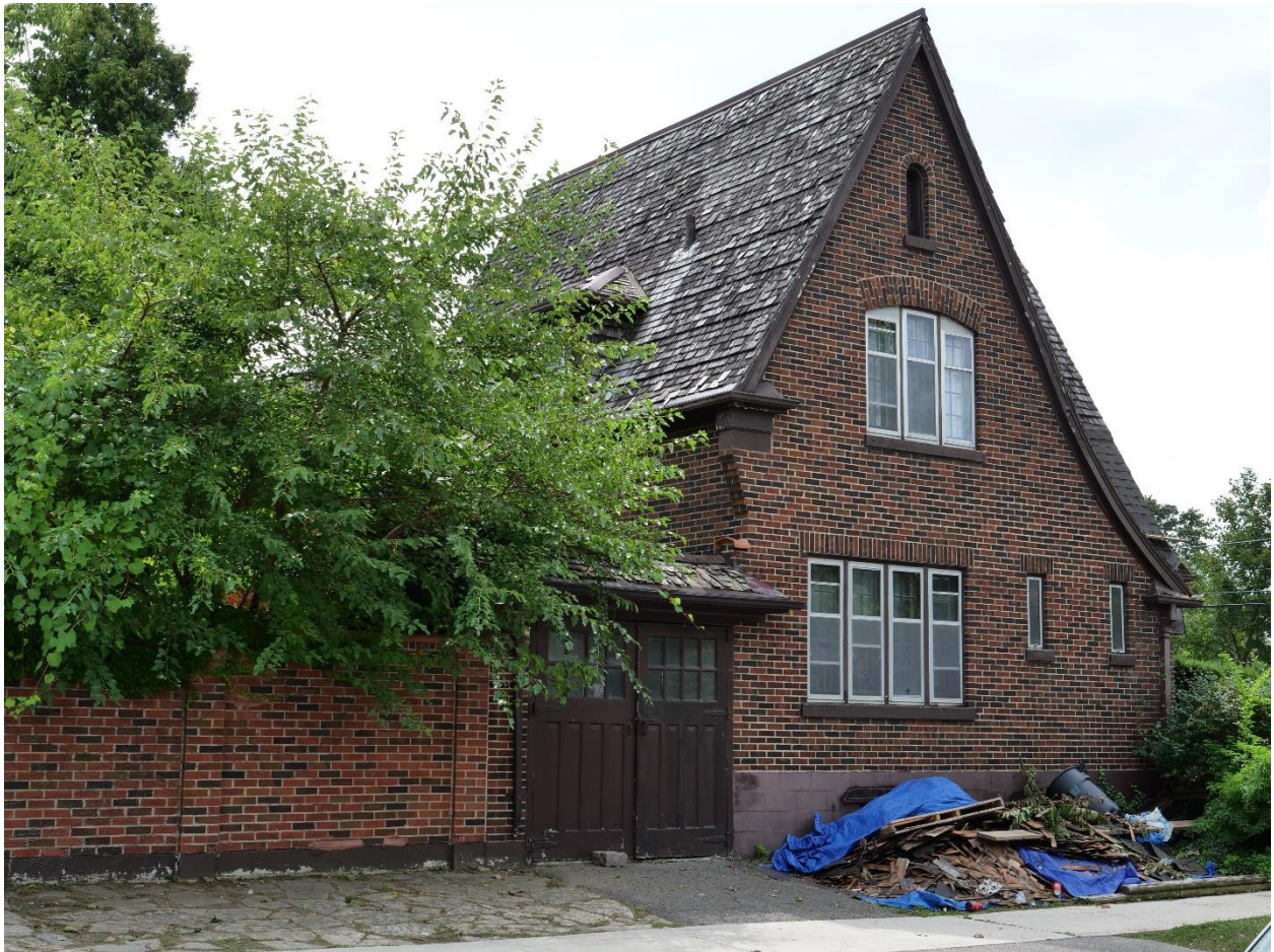
Image 7: Photograph of the property (east and north elevations) at 1058 Richmond Street on August 26, 2019 showing work underway to remove the wood shingle roof and replace it with asphalt shingles.
