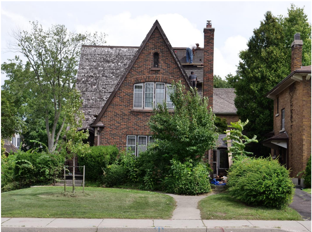
Image 4: Photograph of the property (front/west elevation) at 1058 Richmond Street on August 26, 2019 showing work underway to remove the wood shingle roof and replace it with asphalt shingles.
