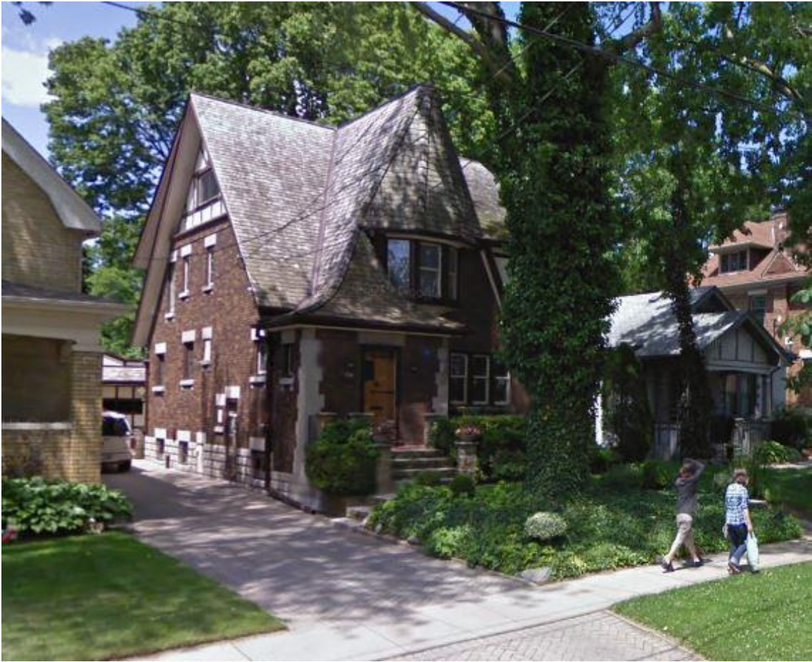
Image 18: Photograph of the property at 516 Grosvenor Street in April 2016, showing the cedar shingle roof (courtesy Google).
