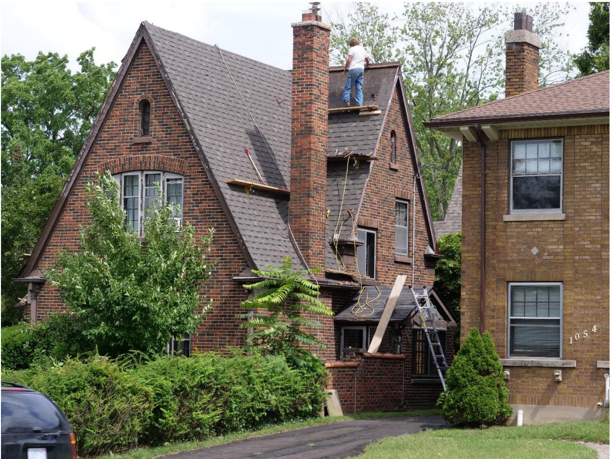
Image 5: Photograph of the property (front/west and south elevations) at 1058 Richmond Street on August 26, 2019 showing work underway to remove the wood shingle roof and replace it with asphalt shingles.
