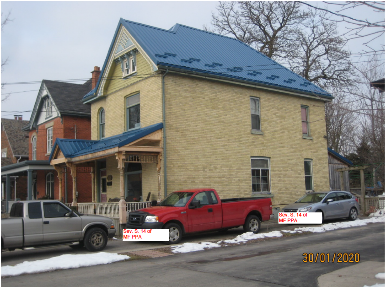
Image 11: Photograph showing the unapproved roof materials alterations completed, and existing status of porch in January 2020
