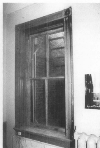
Figure 4f. Following the relatively simple repairs, the window is weathertight, like new in appearance, and serviceable for many years to come. Both the historic material and the detailing and craftsmanship of this original window have been preserved. Photo: John H. Myers
