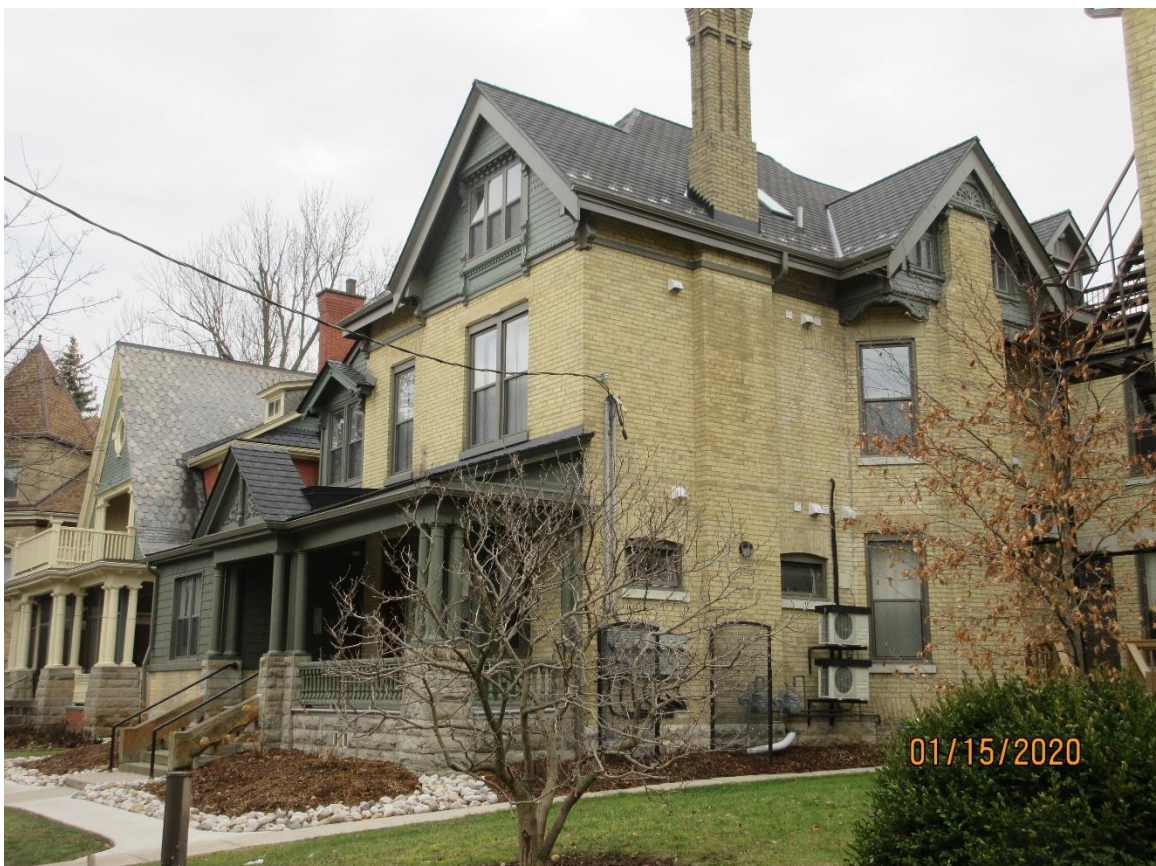
Image 15: Photograph of the property at 309-311 Wolfe Street following roofing replacement with a rubber composite product on January 15, 2020.
