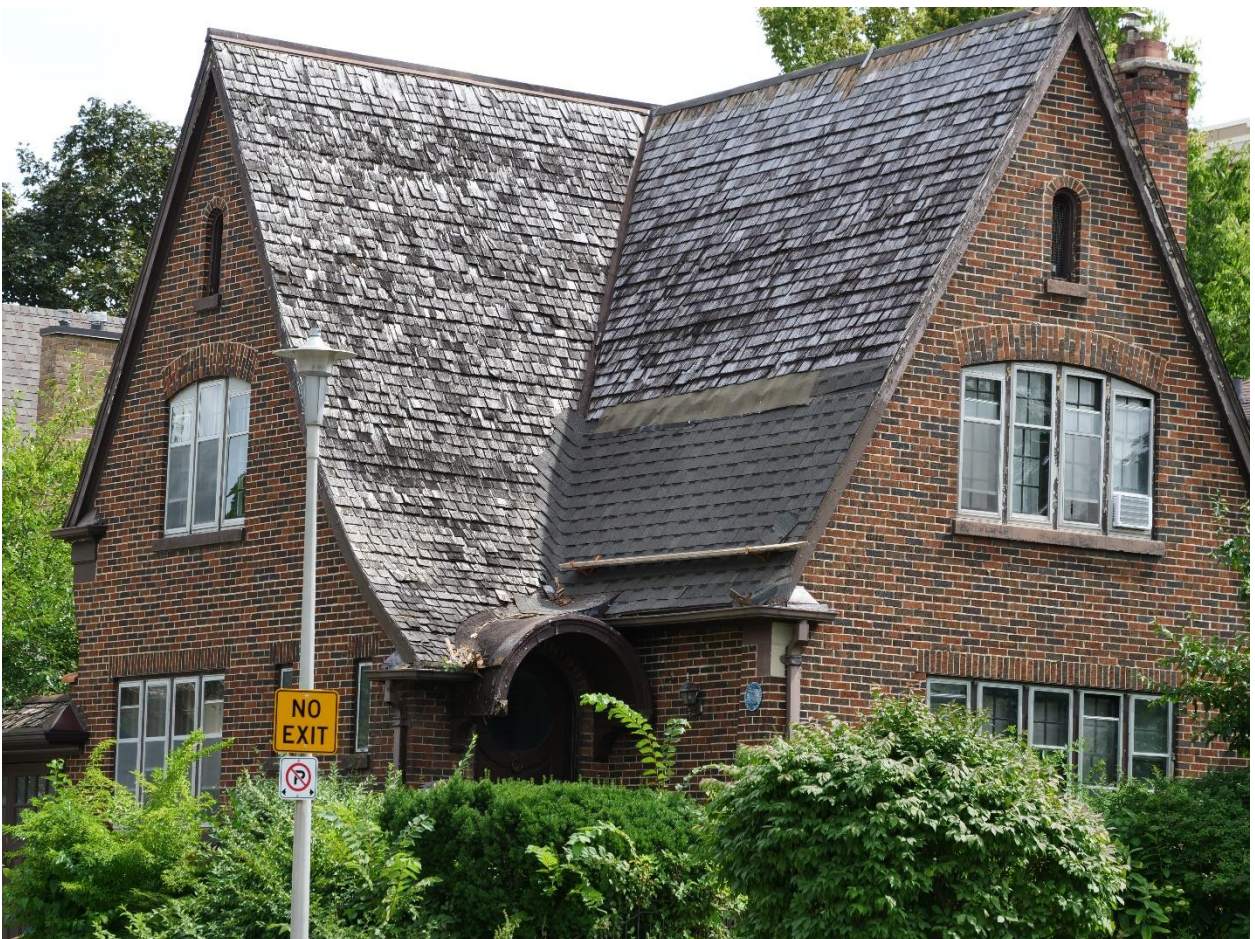
Image 6: Photograph of the property (north and front/west elevations) at 1058 Richmond Street on August 26, 2019 showing work underway to remove the wood shingle roof and replace it with asphalt shingles.
