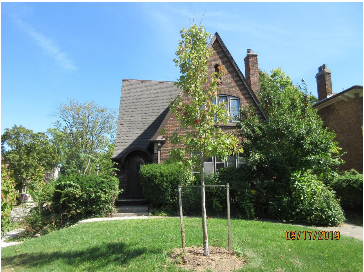
Image 10: Photograph showing the completed roofing replacement with asphalt shingles on the property at 1058 Richmond Street (west/front elevation) on September 17, 2019.
