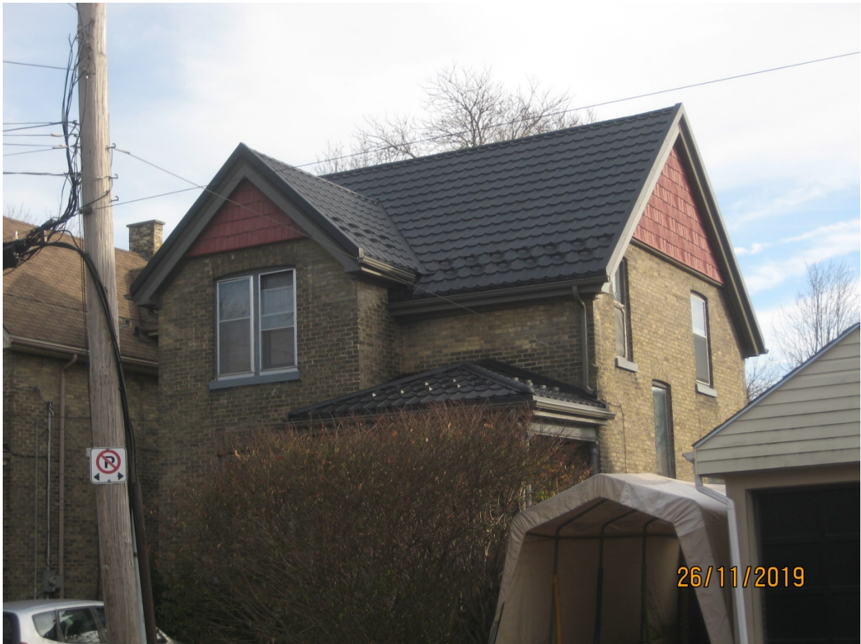
Image 15: Photograph showing unapproved roofing material alteration at 753 Lorne Avenue in November 2019
