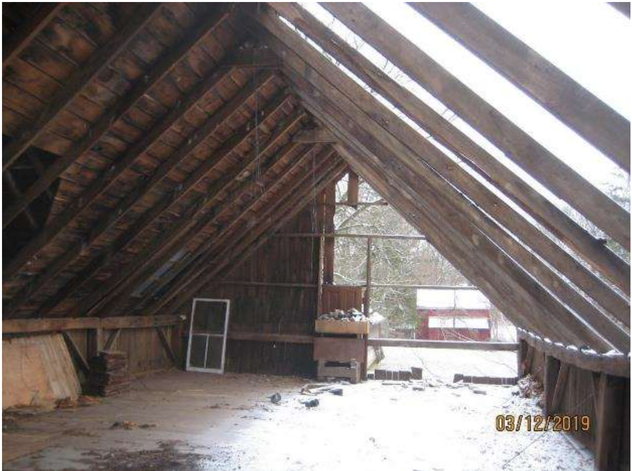
Image 26: Interior view of the loft in the accessory building, approximately one week prior to its collapse, December 3, 2019.
