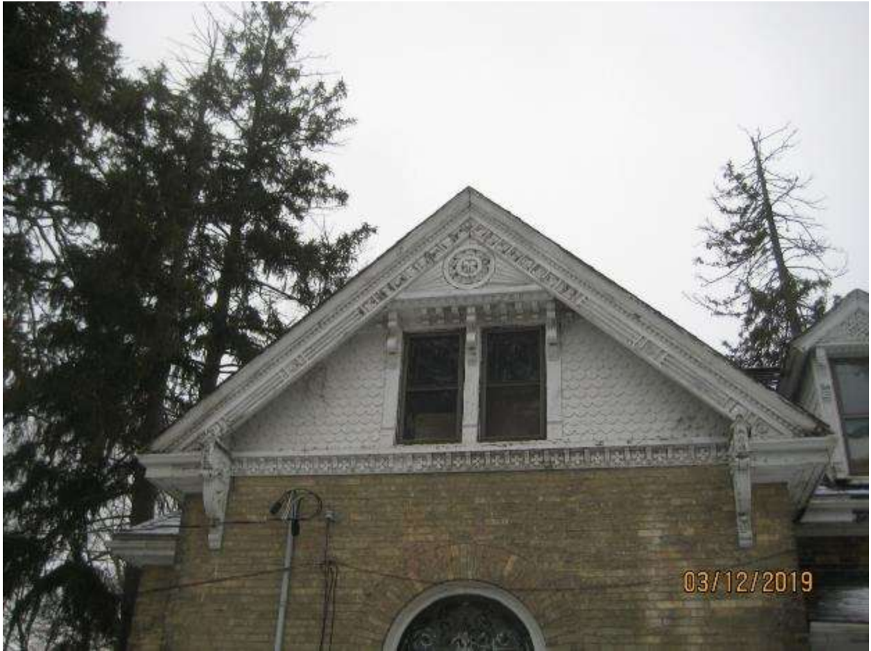
Image 15: Detail showing decorative woodwork in gable on the east elevation of the dwelling, December 2019.
