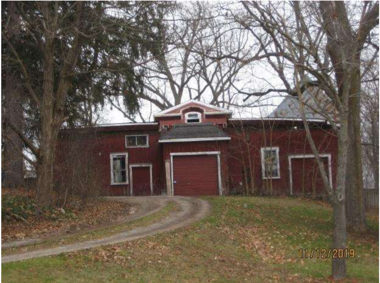
Image 31: Photograph showing the east side of the accessory building as viewed from Halls Mill Road, showing the collapse of the roof framing, December 11, 2019
