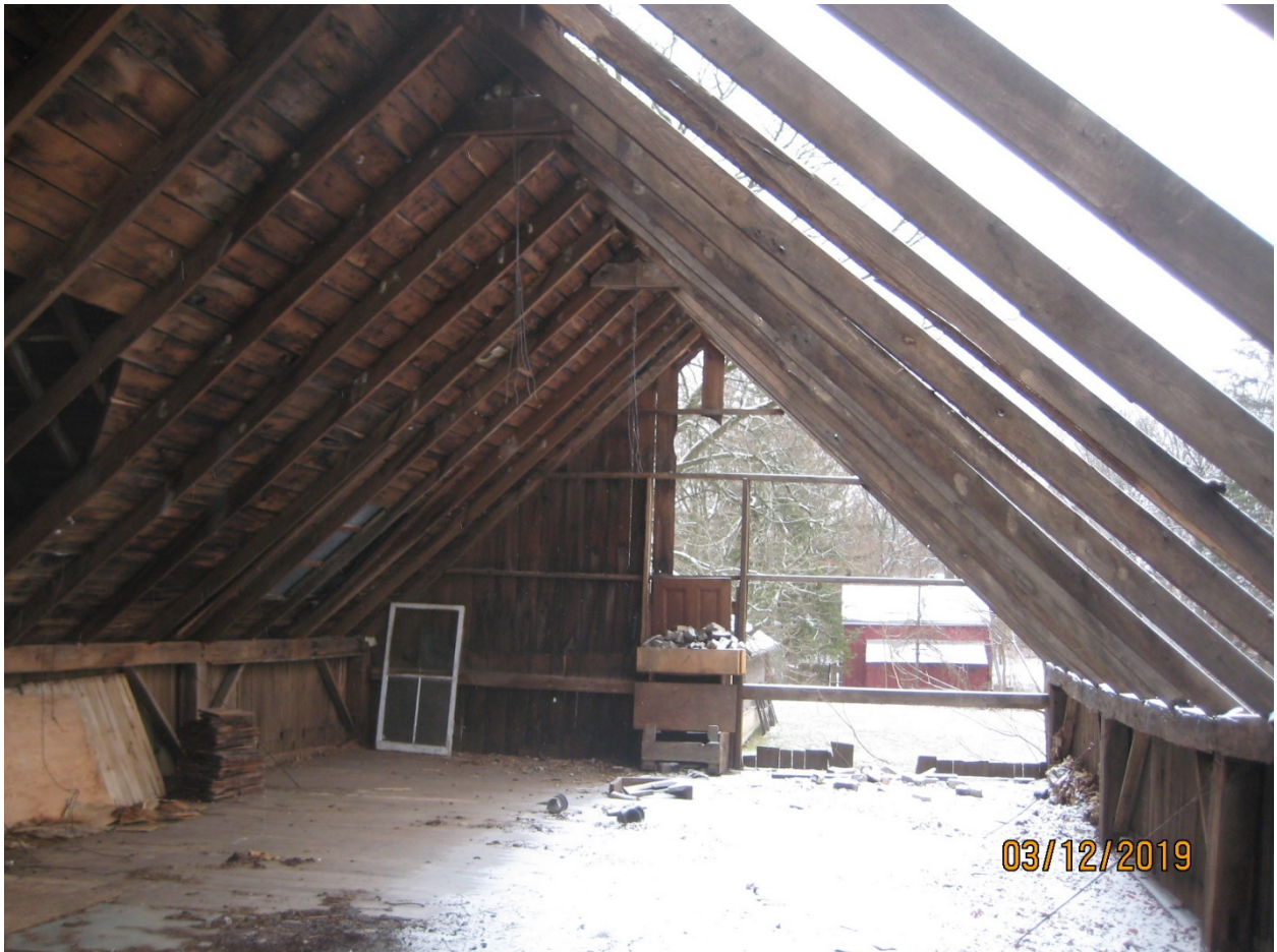
Image 26: Interior view of the loft in the accessory building, approximately one week prior to its collapse, December 3, 2019.
