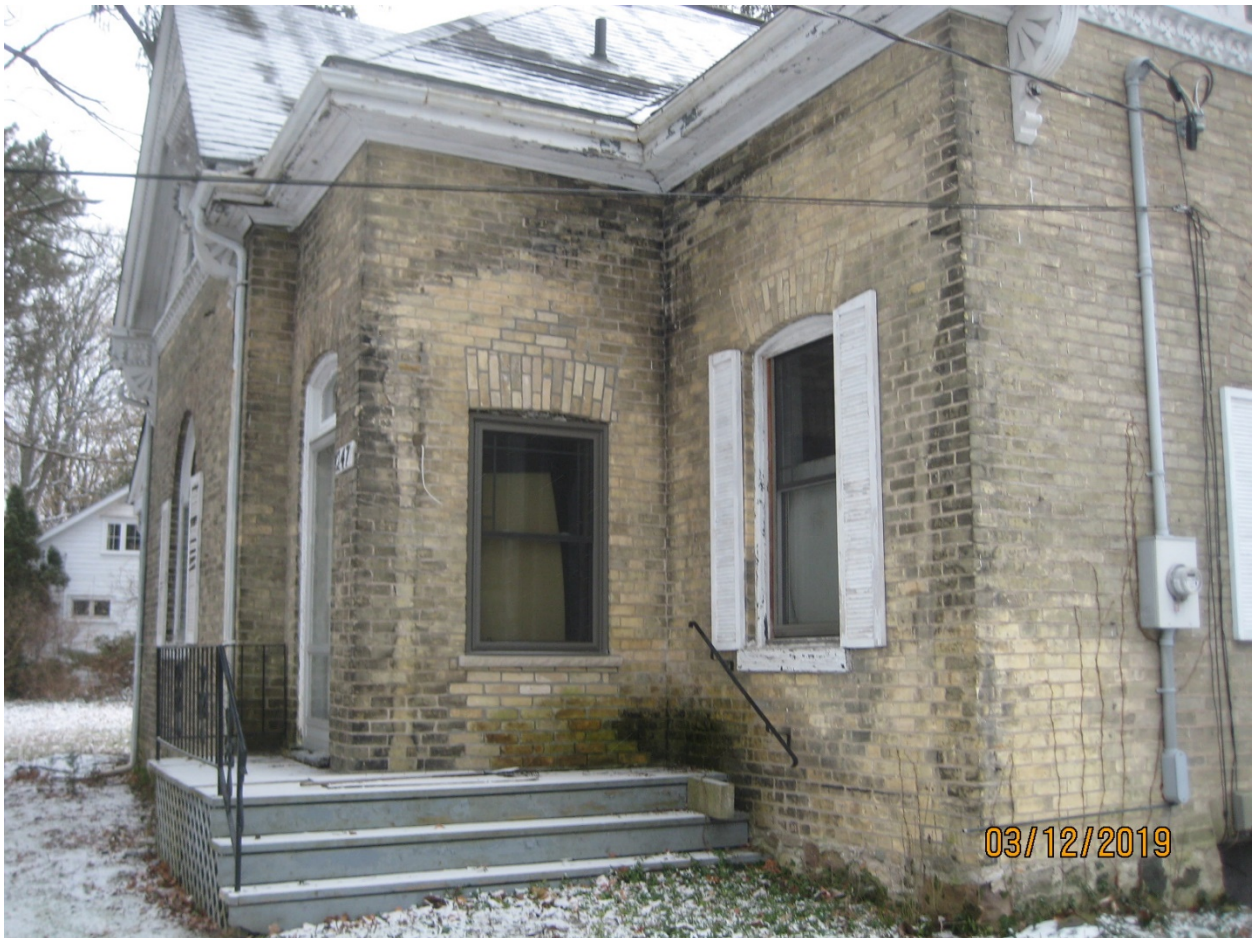
Image 16: Detail showing window/doorway alterations on the east elevation to 247 Halls Mill Road, December 2019.
