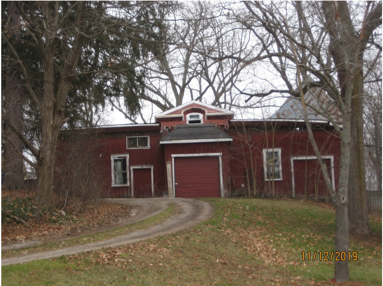
Image 31: Photograph showing the east side of the accessory building as viewed from Halls Mill Road, showing the collapse of the roof framing, December 11, 2019
