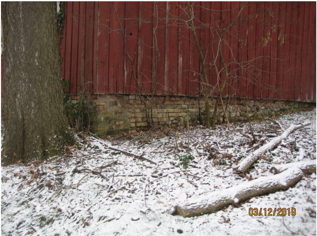
Image 24: Photograph of the foundation on the west side of the accessory building showing a mix of buff brick and field stone materials, December 3, 2019.
