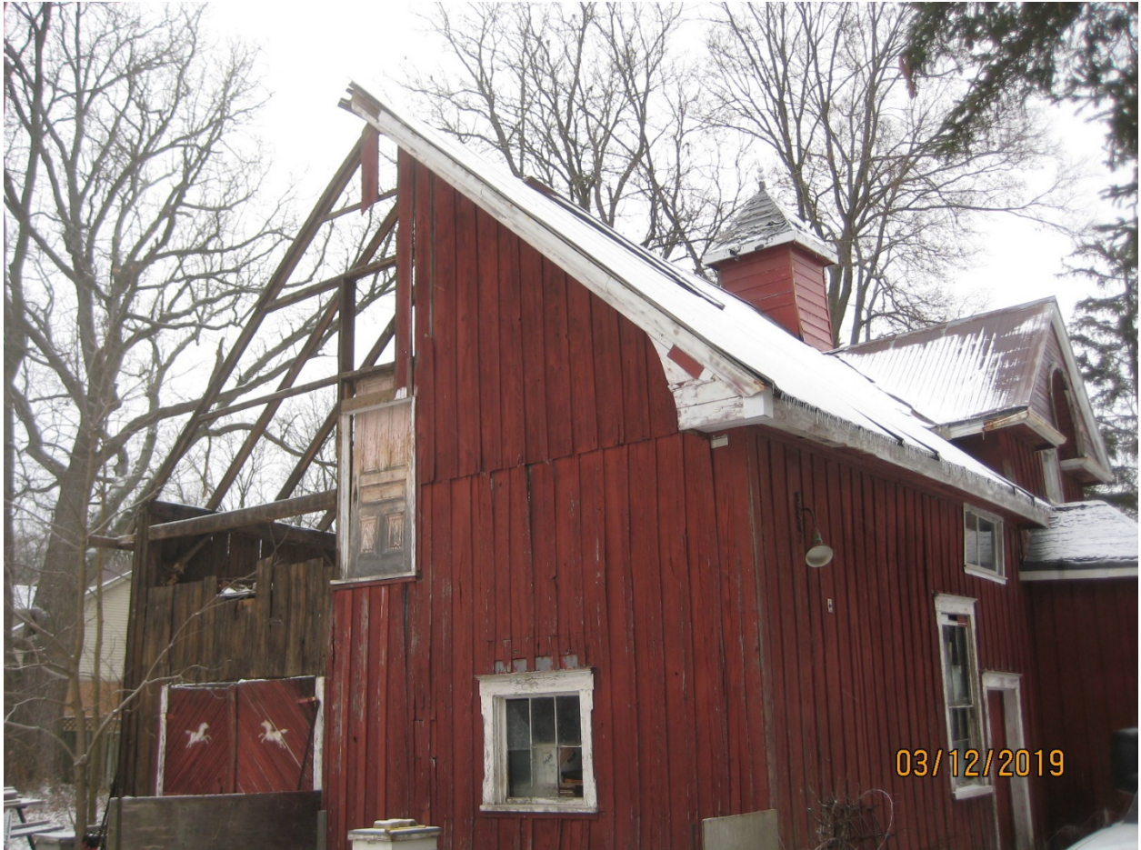
Image 22: Photograph of the south side of the accessory building. Note the portions of the exterior cladding and roof had been removed by the property owner the in the fall of 2019, December 3, 2019.
