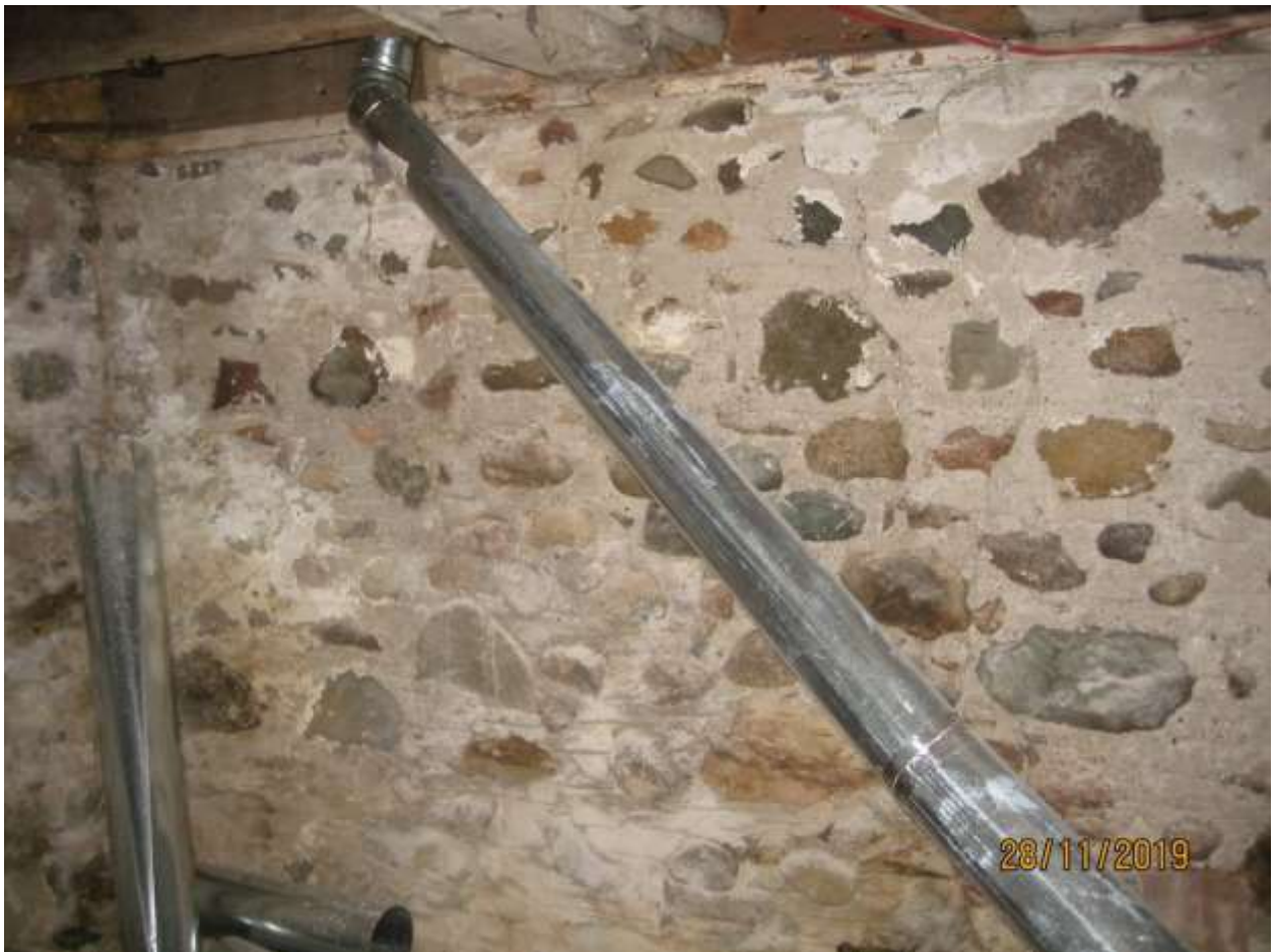
Image 14: Interior detail, showing the field stone foundation walls of the dwelling at 2325 Sunningdale Road East.
