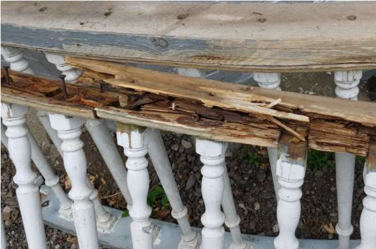
Image 3: Detail of the top and bottom rails on the porch at 906 Lorne Avenue submitted as a part of the Heritage Alteration Permit application, showing the deteriorated wooden elements (October 2019).
