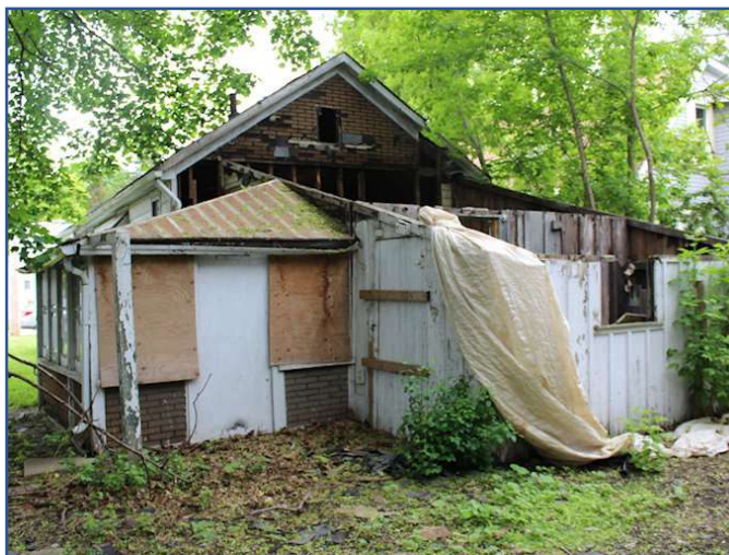
32. The above photograph shows the rear portions of the house in June 2019. These were removed as directed due to concern for public safety.
