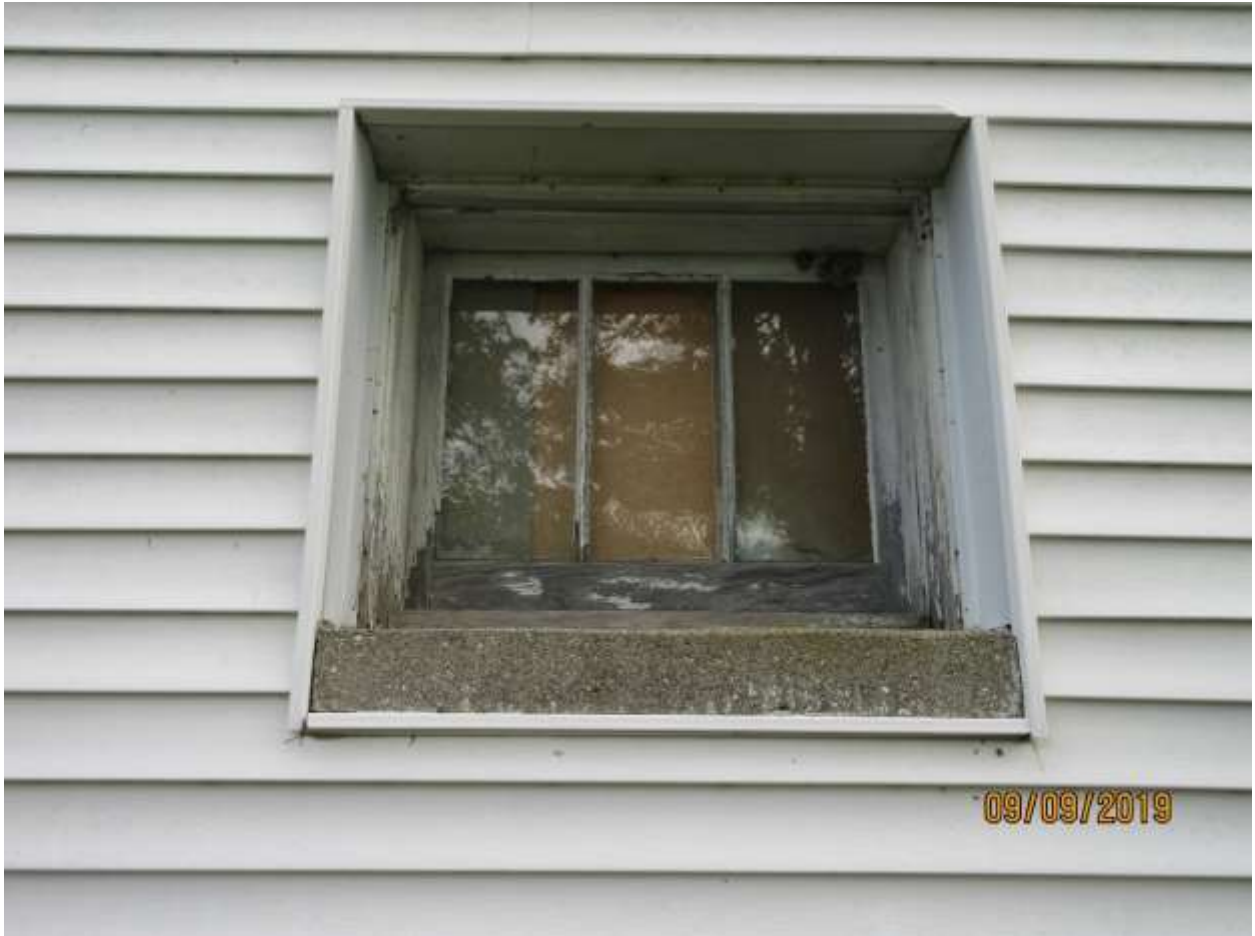
Image 7: The above pictured window on the south façade of the dwelling at 6100 White Oak Road is the only main storey window that is not secured from the exterior (it is boarded from the interior). Also note the concrete window sill.
