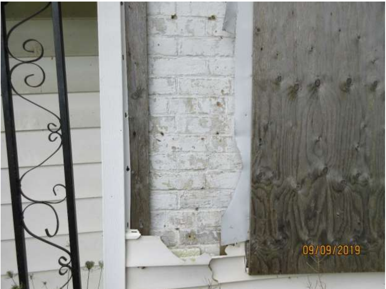
Image 6: Detail of the brickwork, underneath the existing vinyl siding. The brick work appears to be buff brick, with several layers of paint applied. The brickwork appears to be laid in a common bond pattern. The brickwork appears to extend to the ground level, however board cladding prevented the confirmation of this detail.
