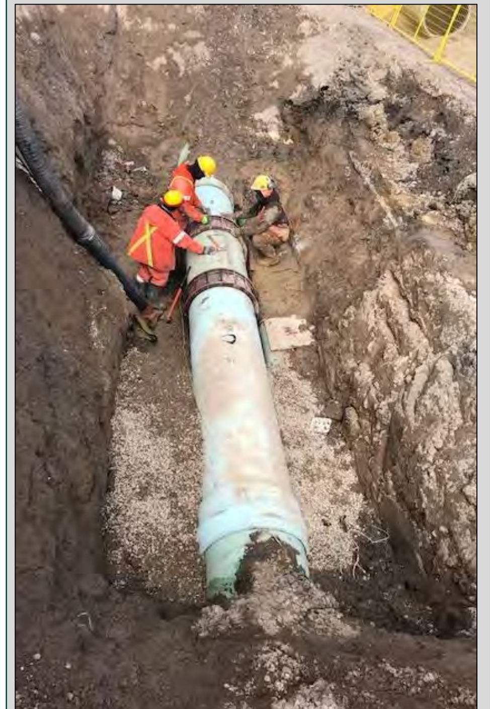
Stormwater Sewer pipes – Conveyance System
