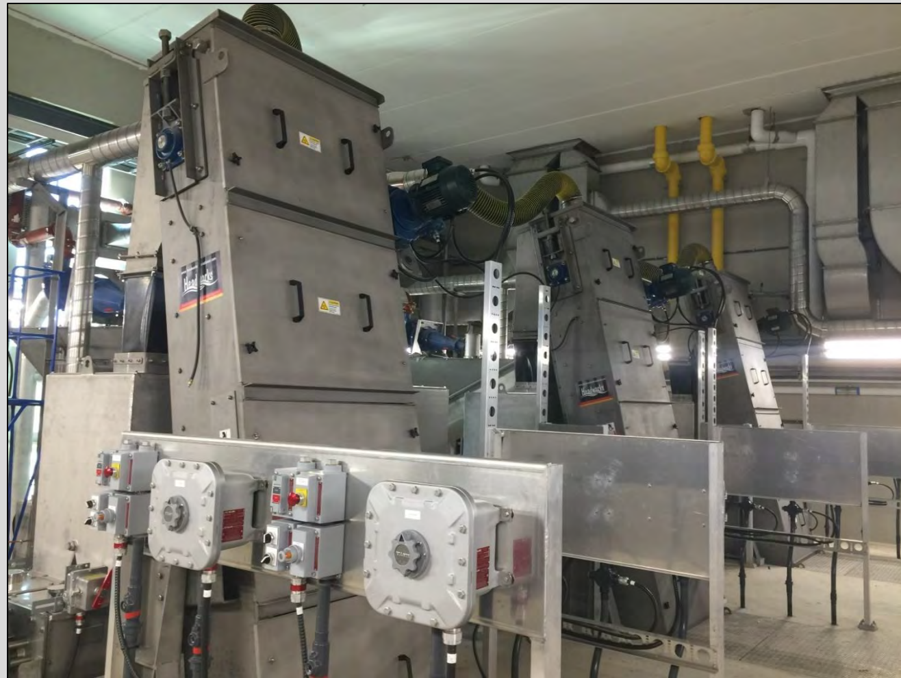
Headworks screens Primary wastewater Treatment – Greenway Wastewater Treatment Plant
