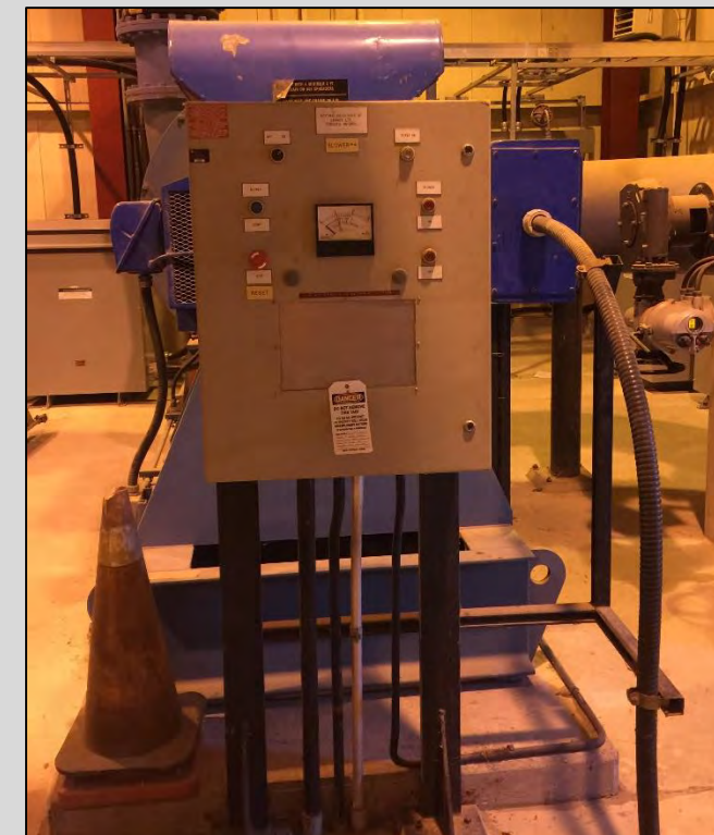
Turbo Blower control unit - Greenway WWTP
