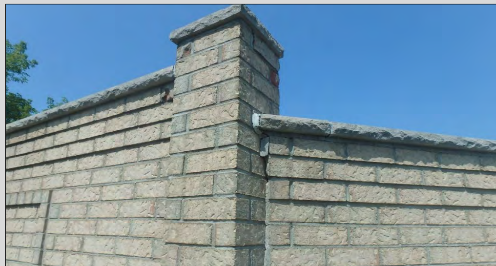
Mason Joints Loss - Noisewall
