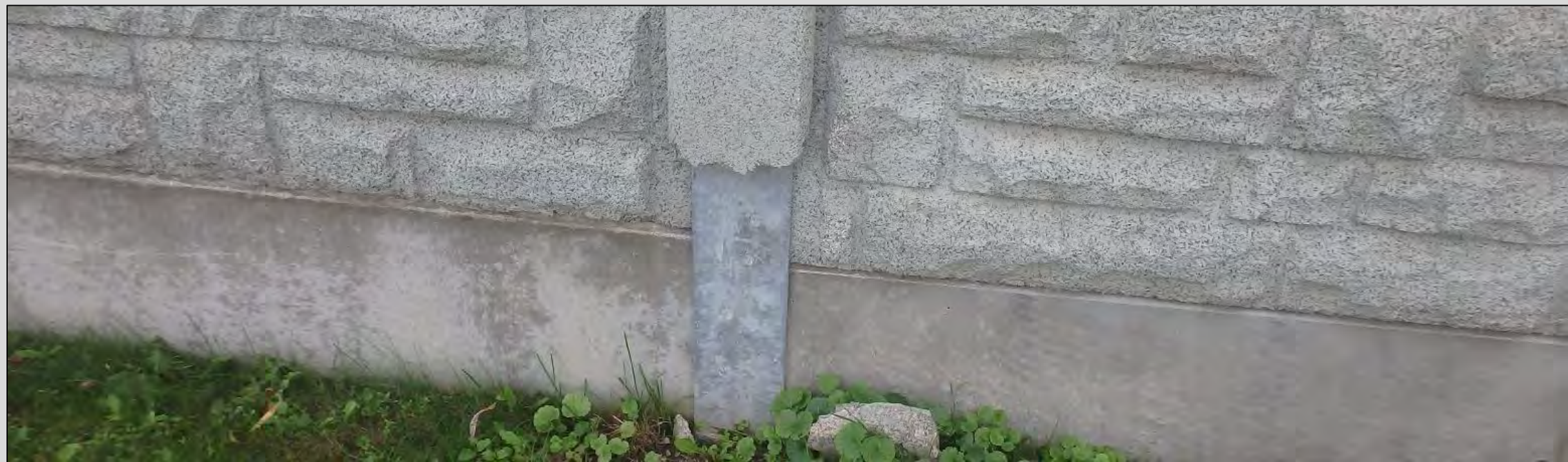
Broken Copping - Noisewall
