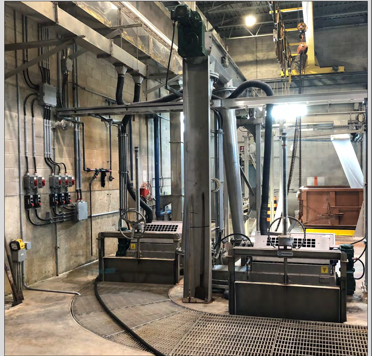
Inlet Screen – Pottersburg Wastewater Treatment Plant
