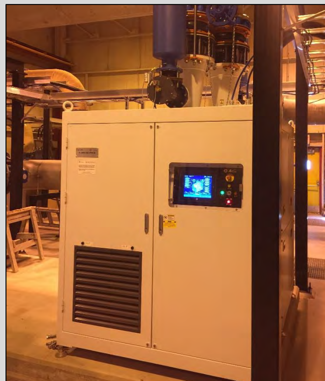
Turbo Blower - Greenway WWTP
