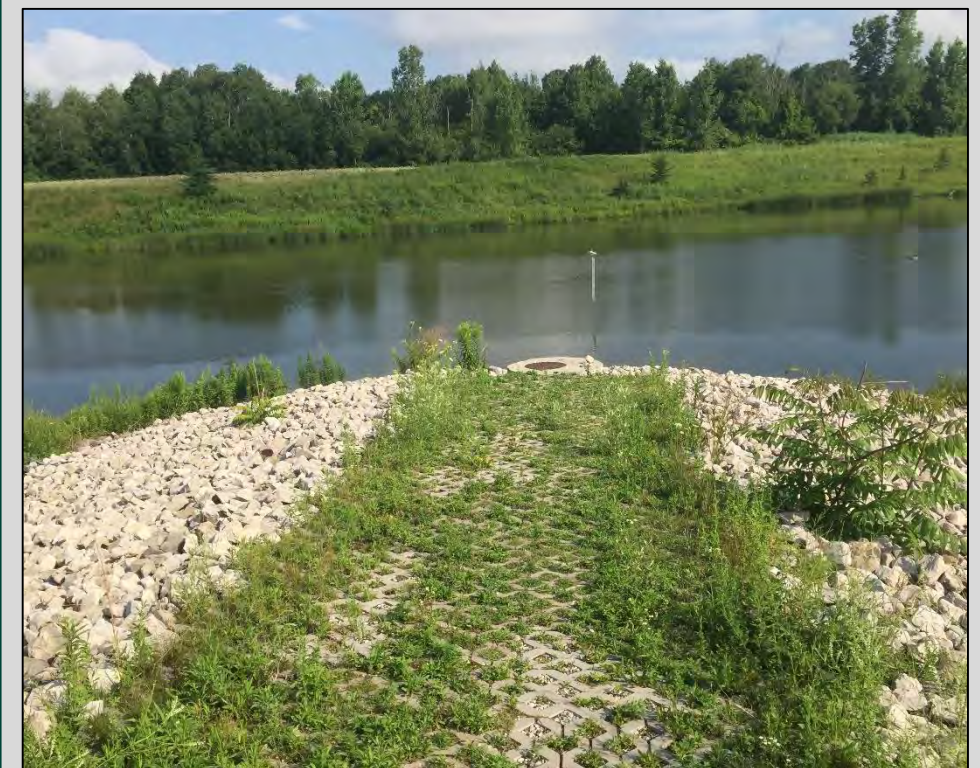
Stormwater Management Facility
