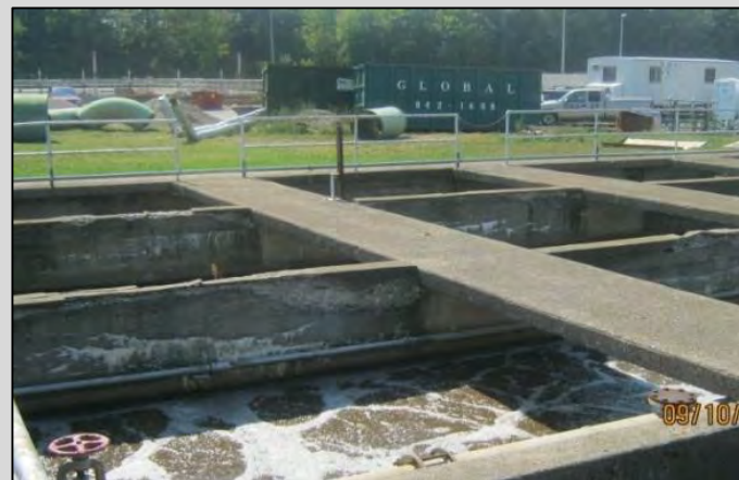
Greenway Section 1 – Crumbling Concrete
