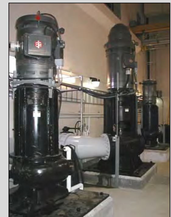
Wastewater Treatment Pumps - Adelaide
