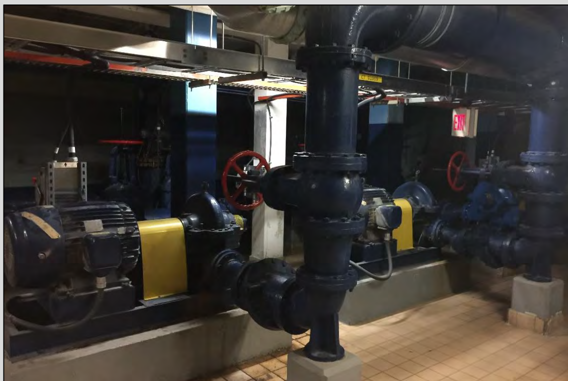
Pumps - Greenway WWTP
