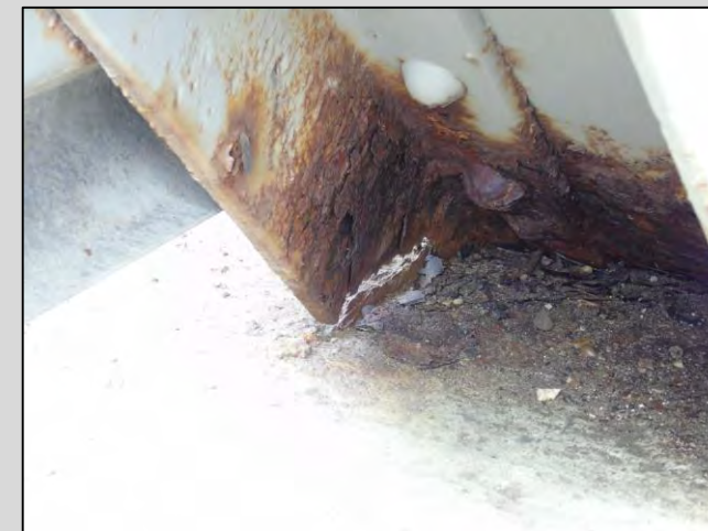
Victoria Bridge – Deterioration and Perforation of S-E Diagonal Truss Member above Sidewalk
