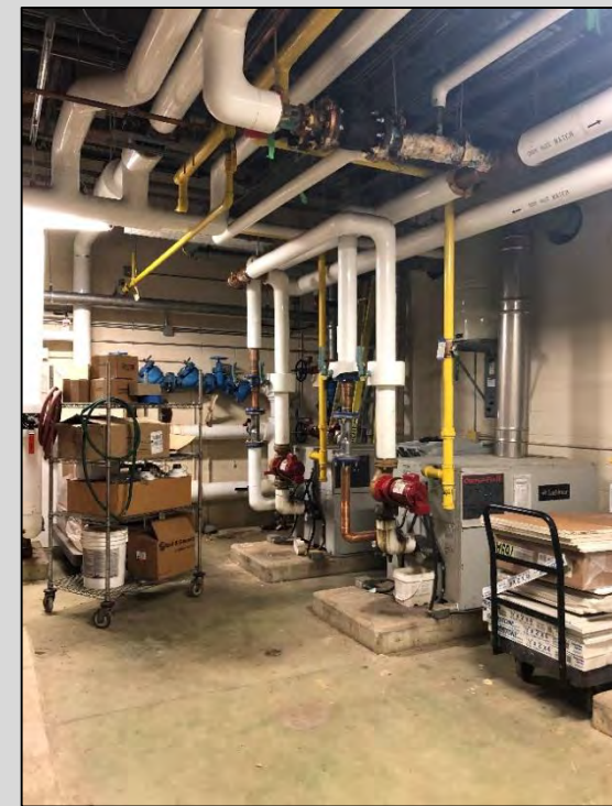
Dearness Home – Boiler and Pump Room
