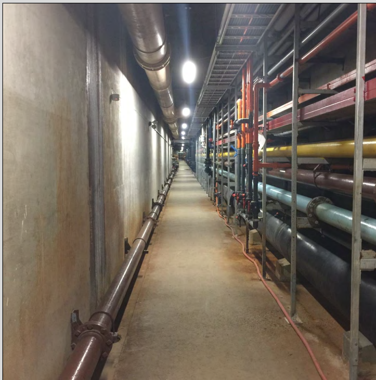
Piping - Greenway Wastewater Treatment Plant
