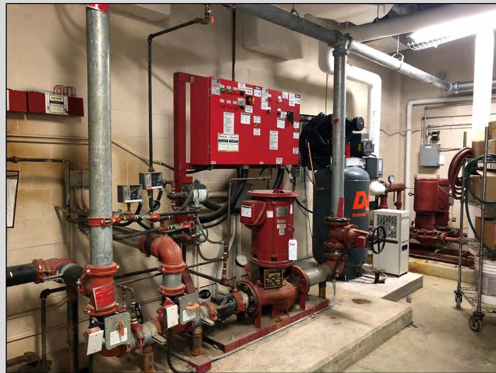
Dearness Home – Boiler and Pump Room
