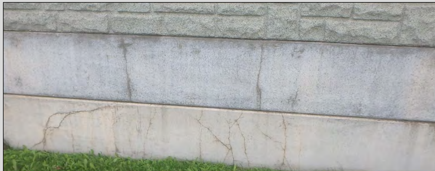
Cracking Retaining Wall
