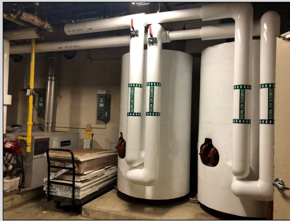
Dearness Home – Boiler and Pump Room
