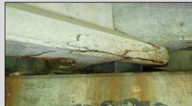
Riverside Bridge over CN Rail – Girder End Delamination
