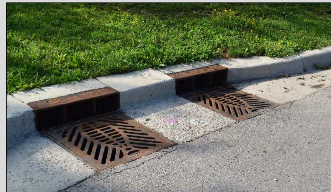
Stormwater Curb Inlet Catch Basins
