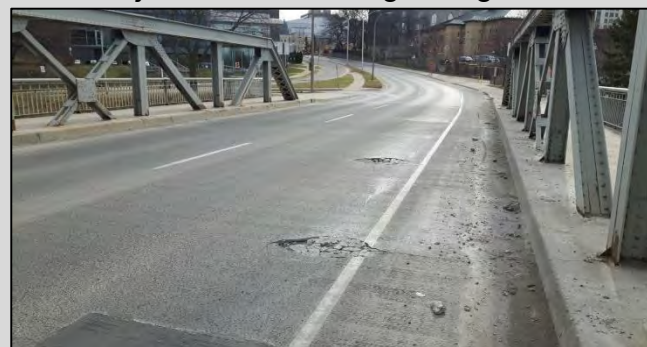
Kensington Bridge – Deck Delaminations
