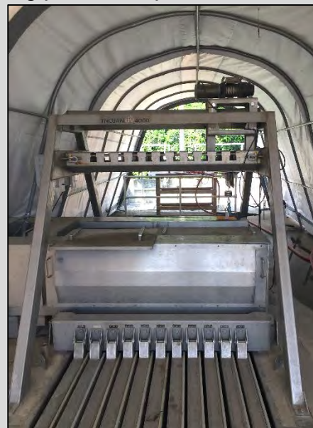
Wastewater Ultra Violet Disinfection Systems Greenway WWTP
