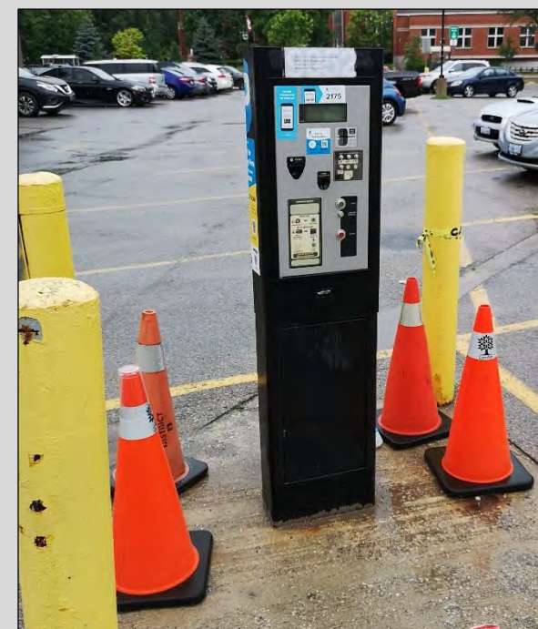
Parking Meter in Deteriorating Condition
