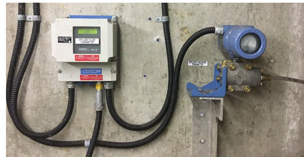
Southwinds Pumping Station Instrumentation
