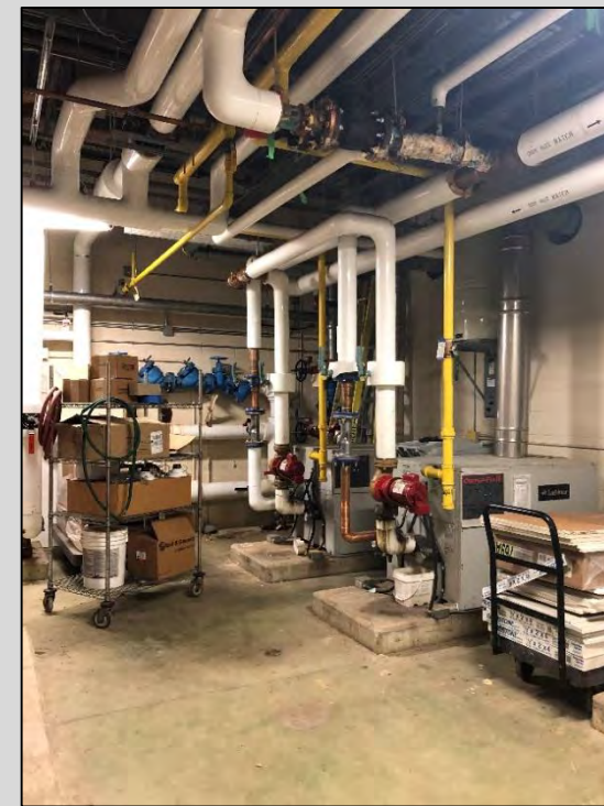
Dearness Home – Boiler and Pump Room
