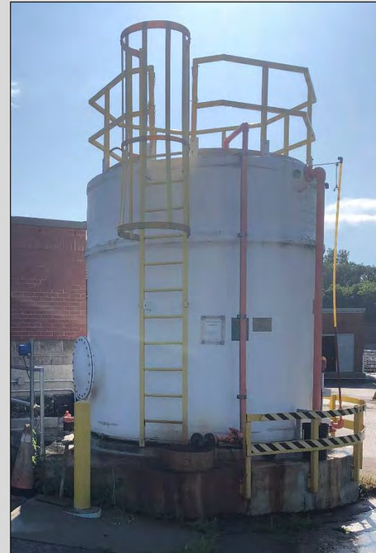
New Ferric Tank at Pottersburg Wastewater Treatment Plant
