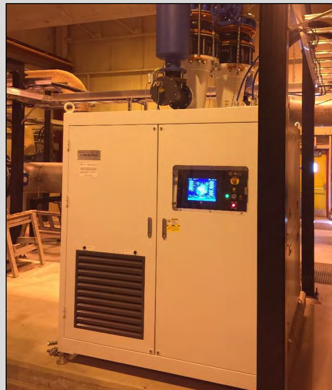
Turbo Blower - Greenway WWTP
