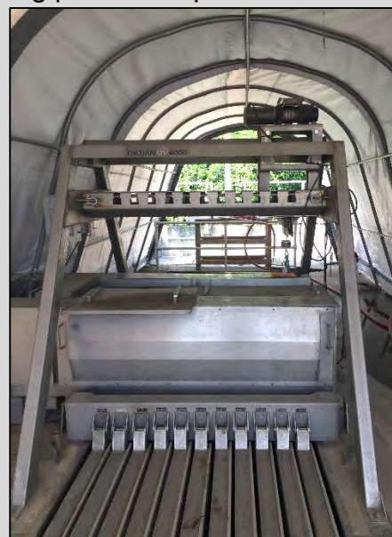
Wastewater Ultra Violet Disinfection Systems Greenway WWTP
