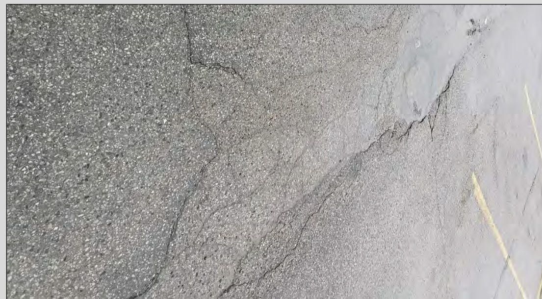
Example of Cracked Surface Lot
