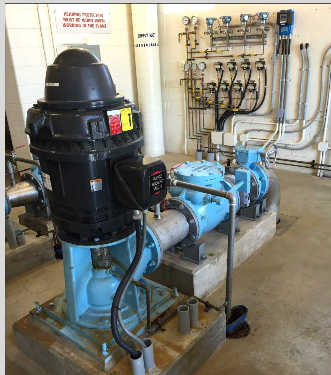
Water pump - South East Reservoir
