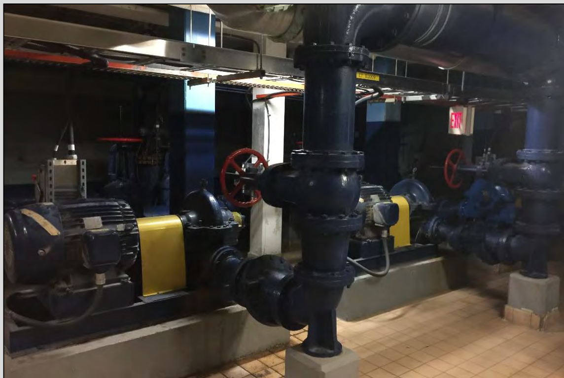
Pumps - Greenway WWTP
