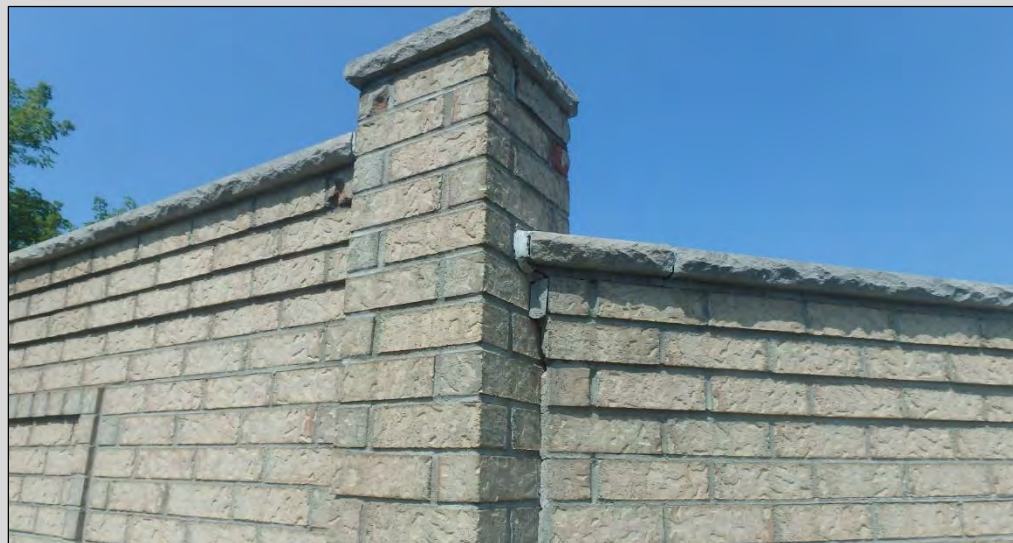
Mason Joints Loss - Noisewall
