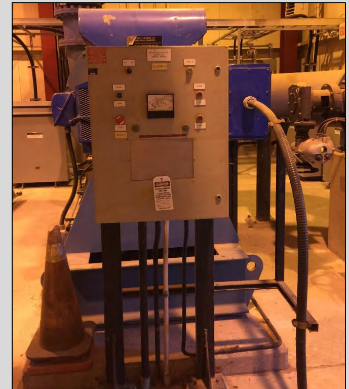
Turbo Blower control unit - Greenway WWTP
