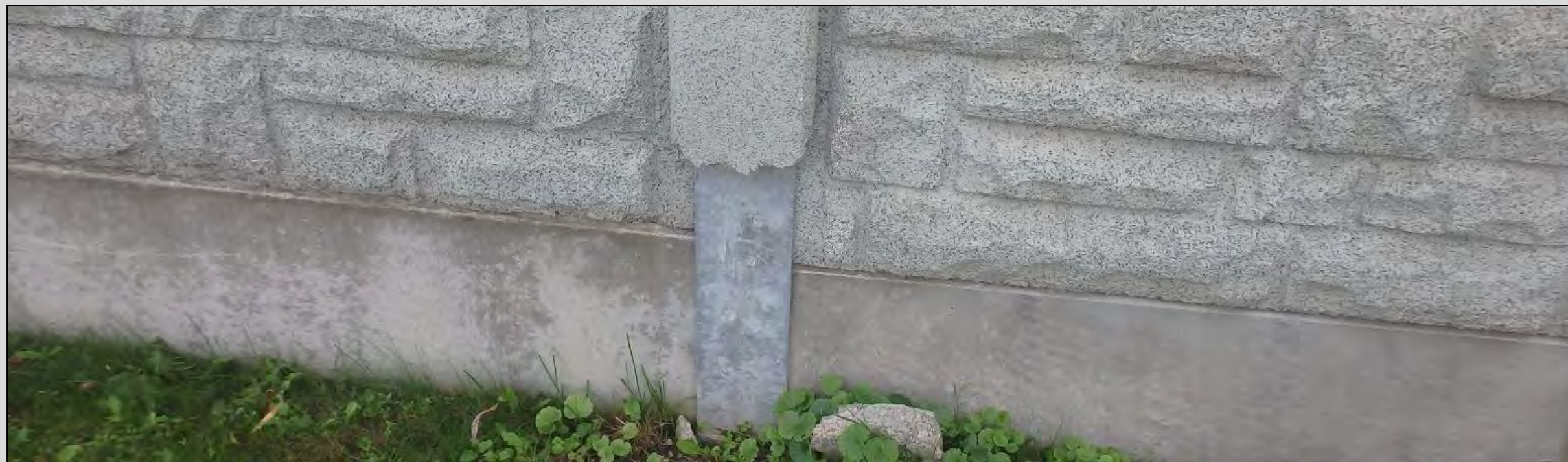
Broken Copping - Noisewall
