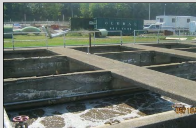
Greenway Section 1 – Crumbling Concrete
