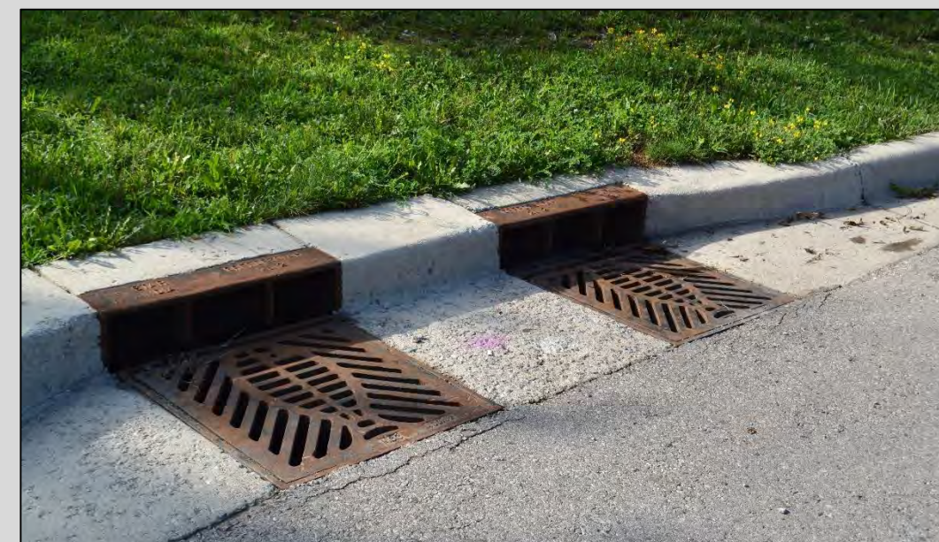
Stormwater Curb Inlet Catch Basins
