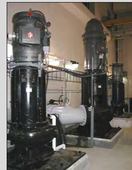
Wastewater Treatment Pumps - Adelaide
