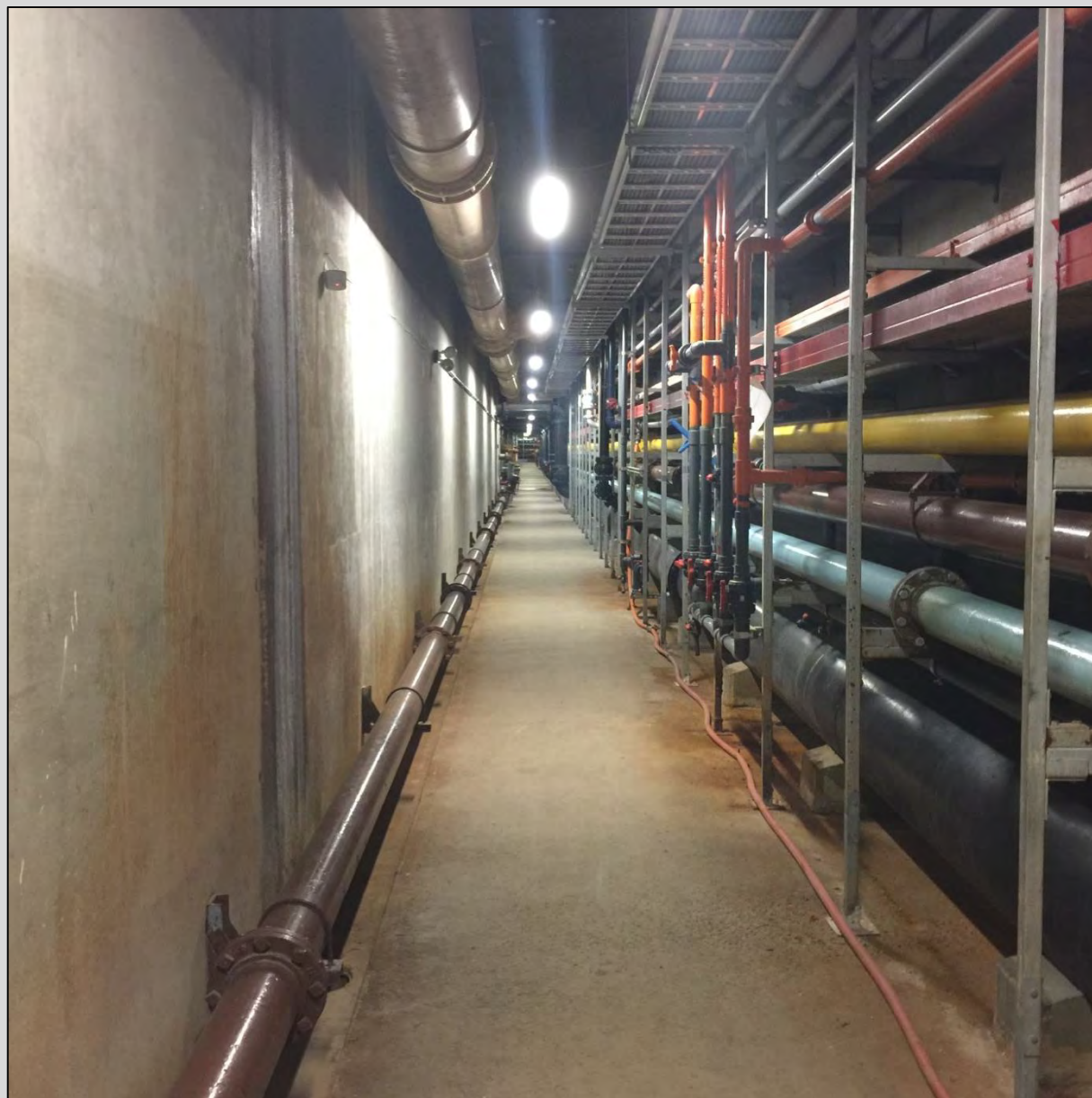
Piping - Greenway Wastewater Treatment Plant
