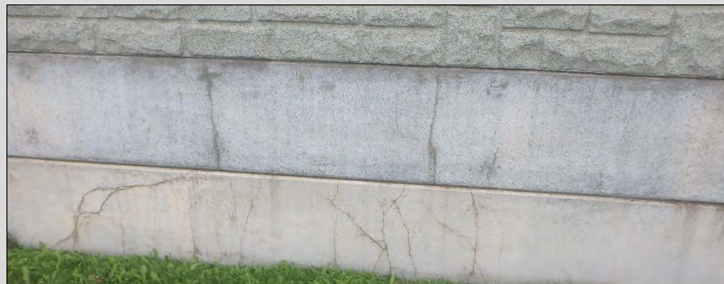
Cracking Retaining Wall
