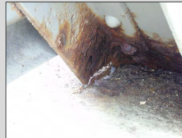
Victoria Bridge – Deterioration and Perforation of S-E Diagonal Truss Member above Sidewalk
