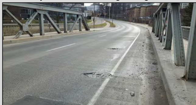
Kensington Bridge – Deck Delaminations
