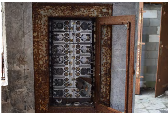
Plate 75: Fuse box, looking west
