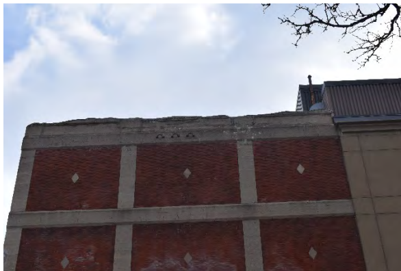
Plate 20: Second and third storey concrete banding and concrete diamonds topped by a concrete parapet, looking south
