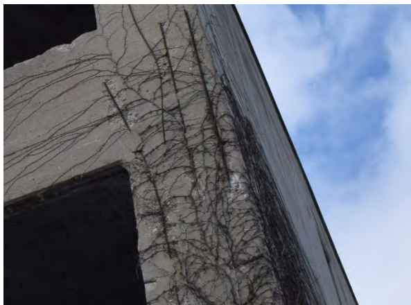
Plate 31: Exposed rebar, looking north
