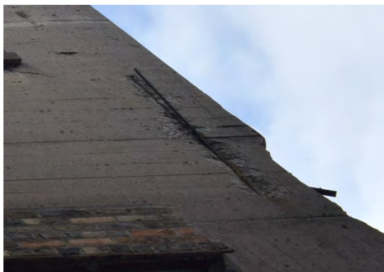
Plate 35: Exposed rebar on west façade, looking east
