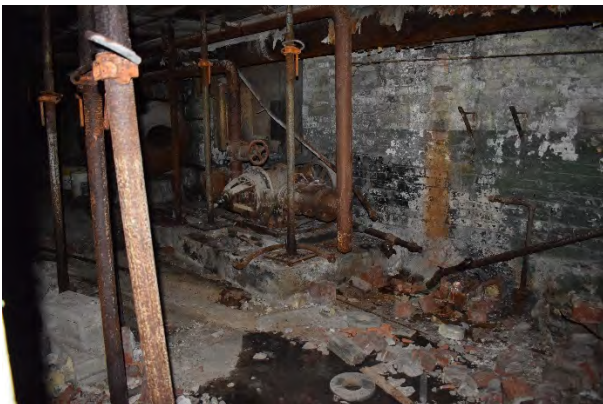
Plate 86: Southwest room with machinery, looking west
