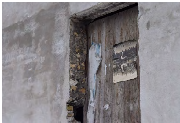
Plate 30: Eroded window opening, showing buff brick exterior, looking west
