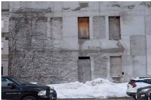
Plate 27: Blind and boarded window and door of south half of first storey on east façade, looking west
