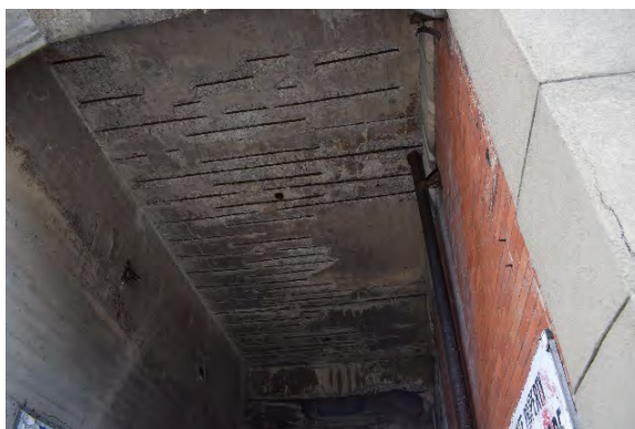
Plate 45: Exposed rebar, looking south
