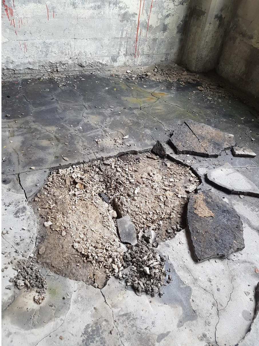
Photograph No. 2 – Asphalt Layer Overlying the Poor Concrete Floor Slab
