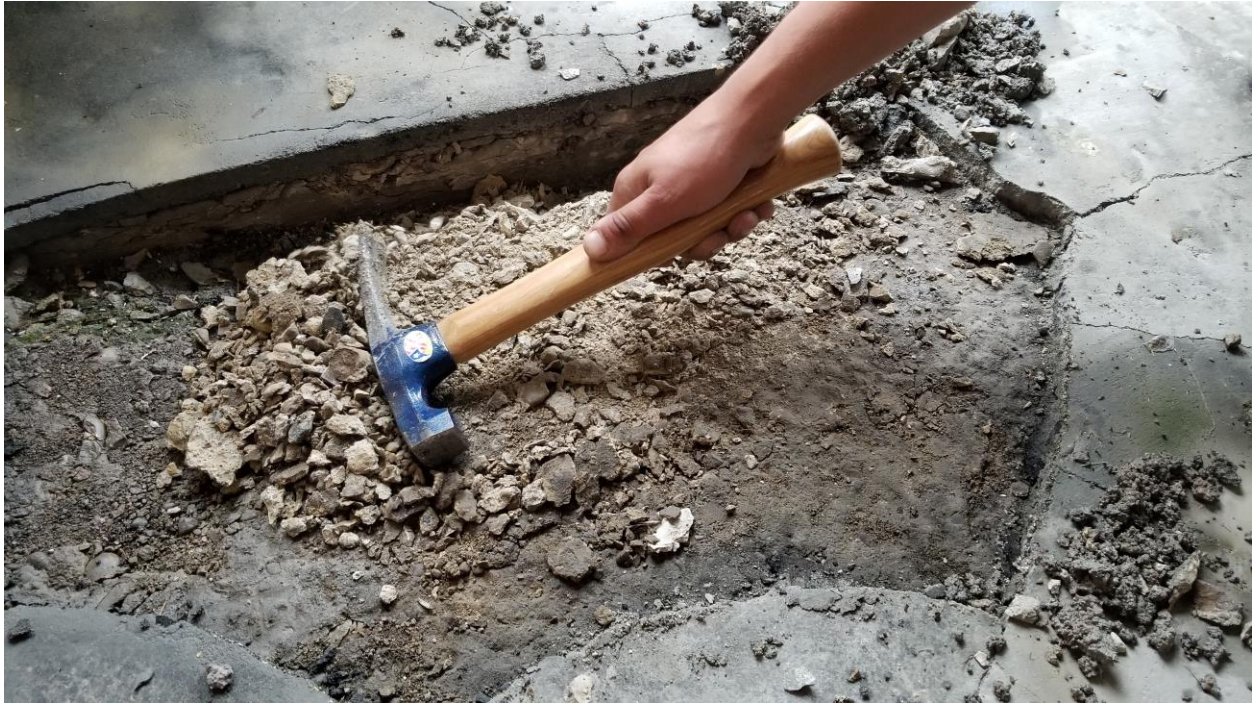
Photograph No. 4 – Broken Pieces/Crumble of Concrete Floor Showing Unsuitable Coring Conditions
