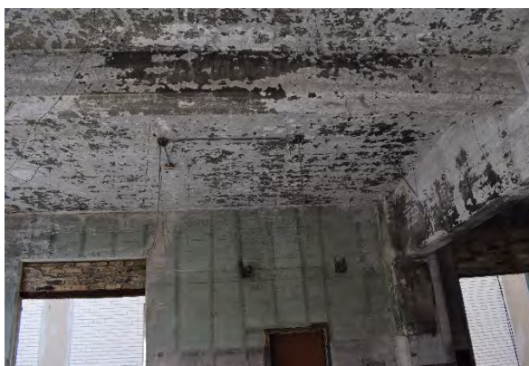
Plate 69: Wiring for light fixtures
