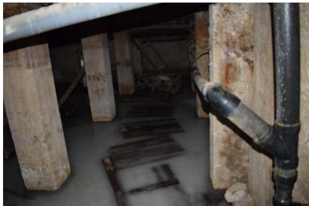
Plate 87: Flooded southwest room, looking south
