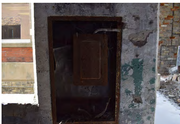
Plate 67: Electrical box, looking west
