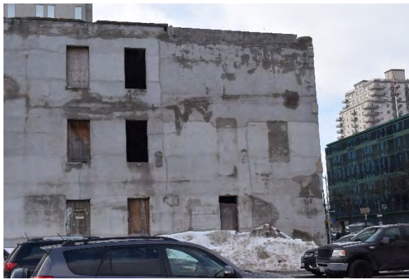
Plate 28: Blind and boarded windows on north half of east façade, looking west
