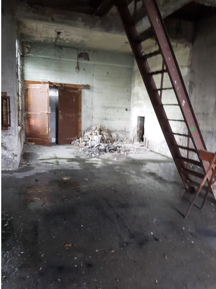
Photograph No. 3 – Overall Picture Showing Poor Concrete Floor and Wall Conditions
