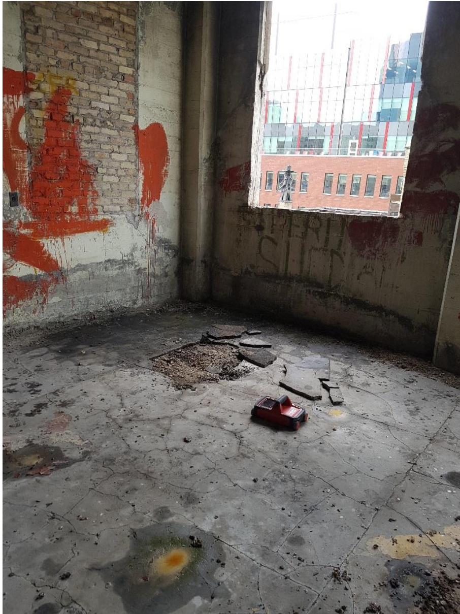
Photograph No. 1 – Severe Concrete Floor and Wall Cracks
