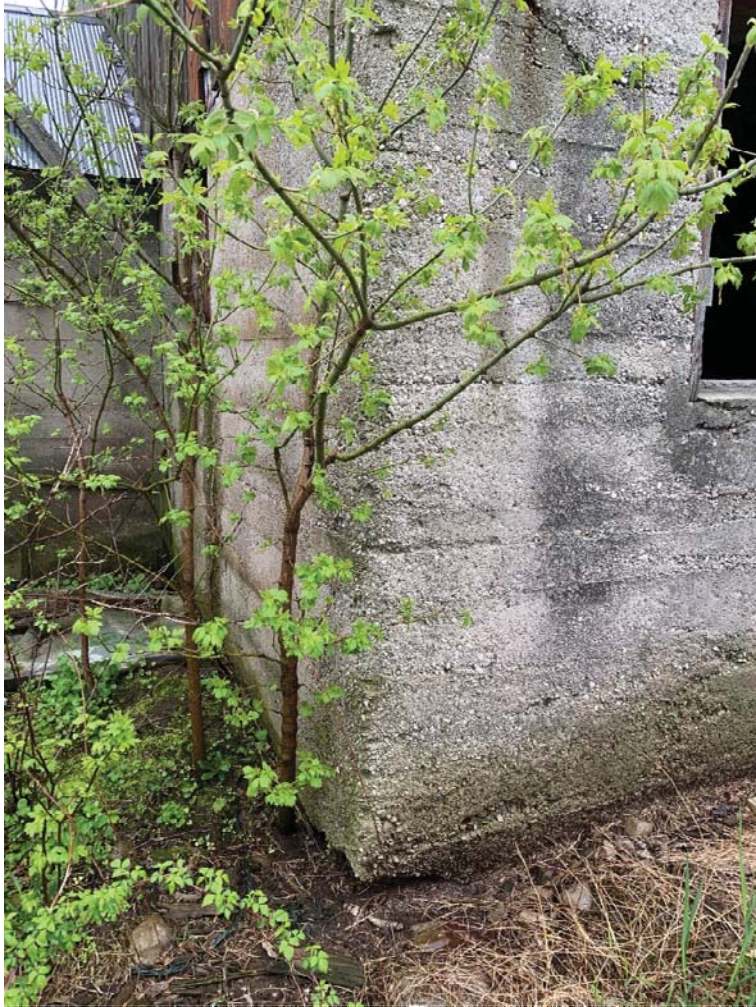
Figure 8.0 - Photo of Pitting/Deterioration and Undermining of Existing Foundation Wall
