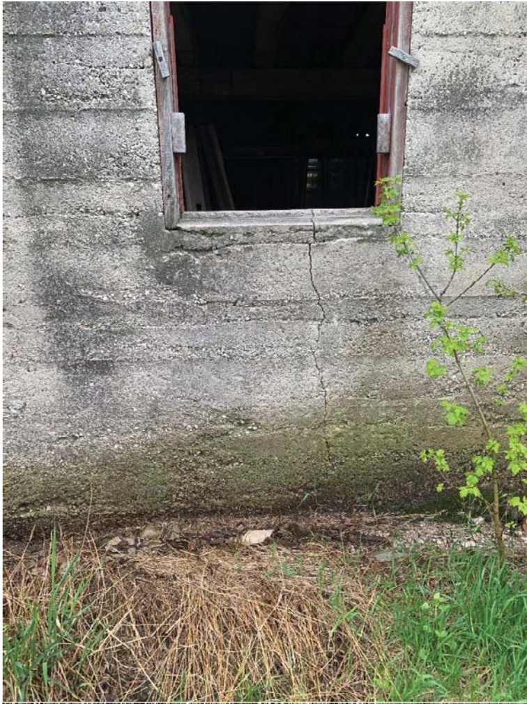
Figure 9.0 - Photo of Cracked Existing Foundation Wall
