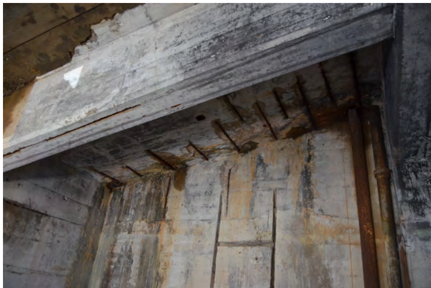
Photo No 11: Interior Suspended Slab (Delaminated Concrete)
