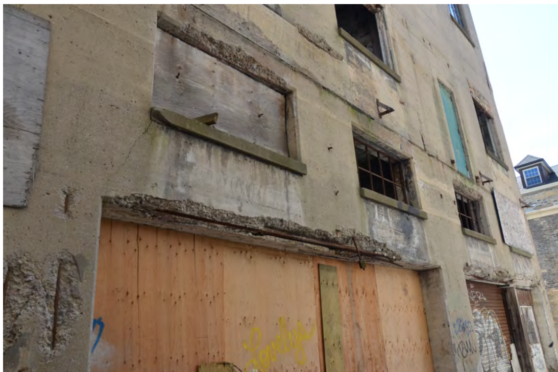
Photo No 04: Delaminated Concrete Beams
