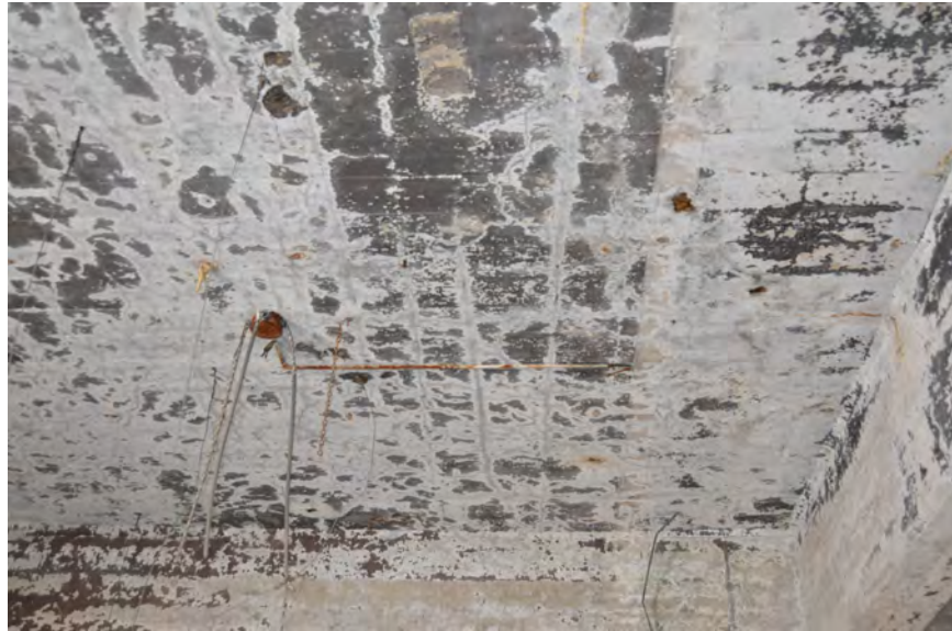
Photo No 10: Interior Suspended Slab (cracked along rebar)
