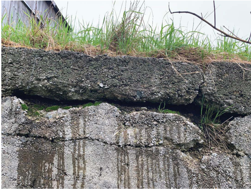
Figure 3.0 - Photo of Existing Ramp Structure with Severe Delamination/Spalling
