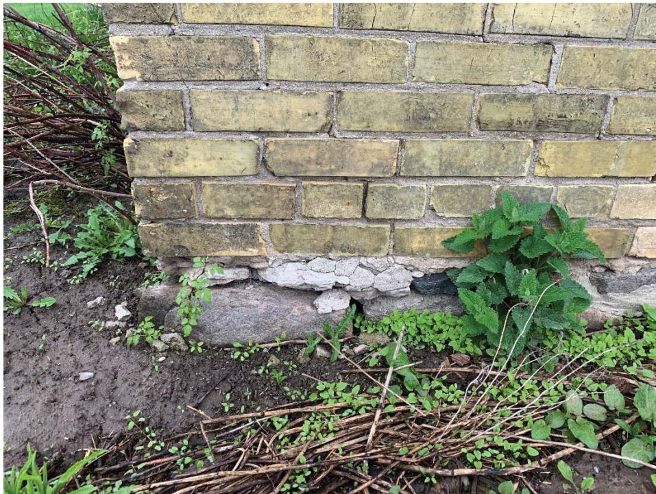
Figure 2.0 – Photo of Existing Foundation Wall Structure with Deteriorated Mortar Joints
