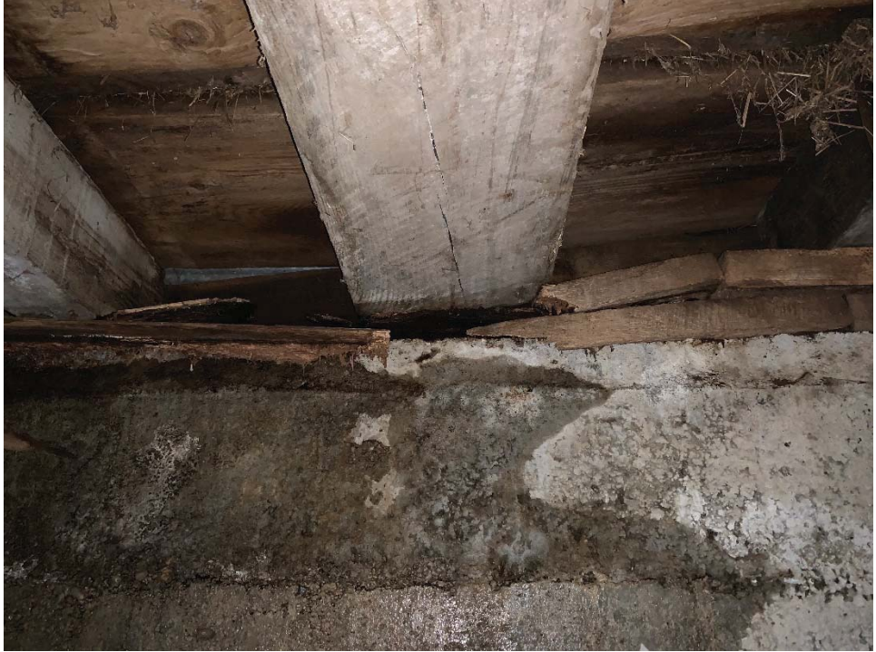
Figure 7.0 - Photo of Damaged Perimeter Sill-plate
