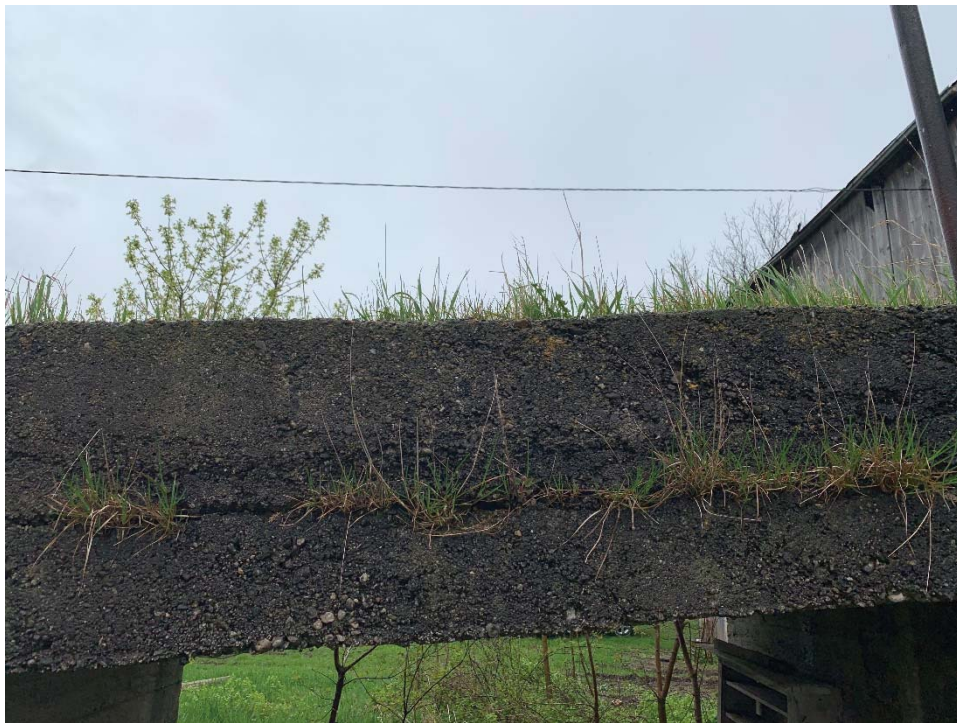
Figure 2.0 – Photo of Existing Ramp Structure with Severe Delamination
