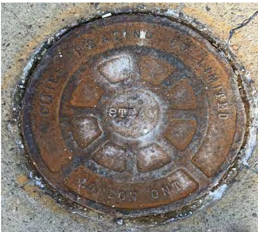
Plate 13: CHC manhole cover, located outside 171 Queens Avenue
