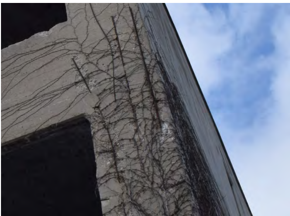
Plate 31: Exposed rebar, looking north
