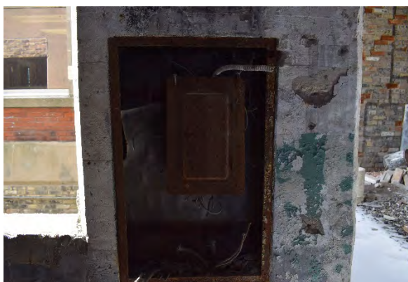
Plate 67: Electrical box, looking west
