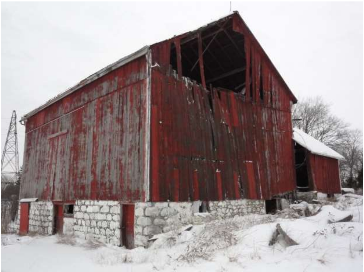
Image 4: View of barn, east-south corner illustrating gangway, rubble foundation and lower stable level (2019-02-14).
