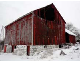
View of barn, east-south corner illustrating gangway, rubble foundation and lower stable level
