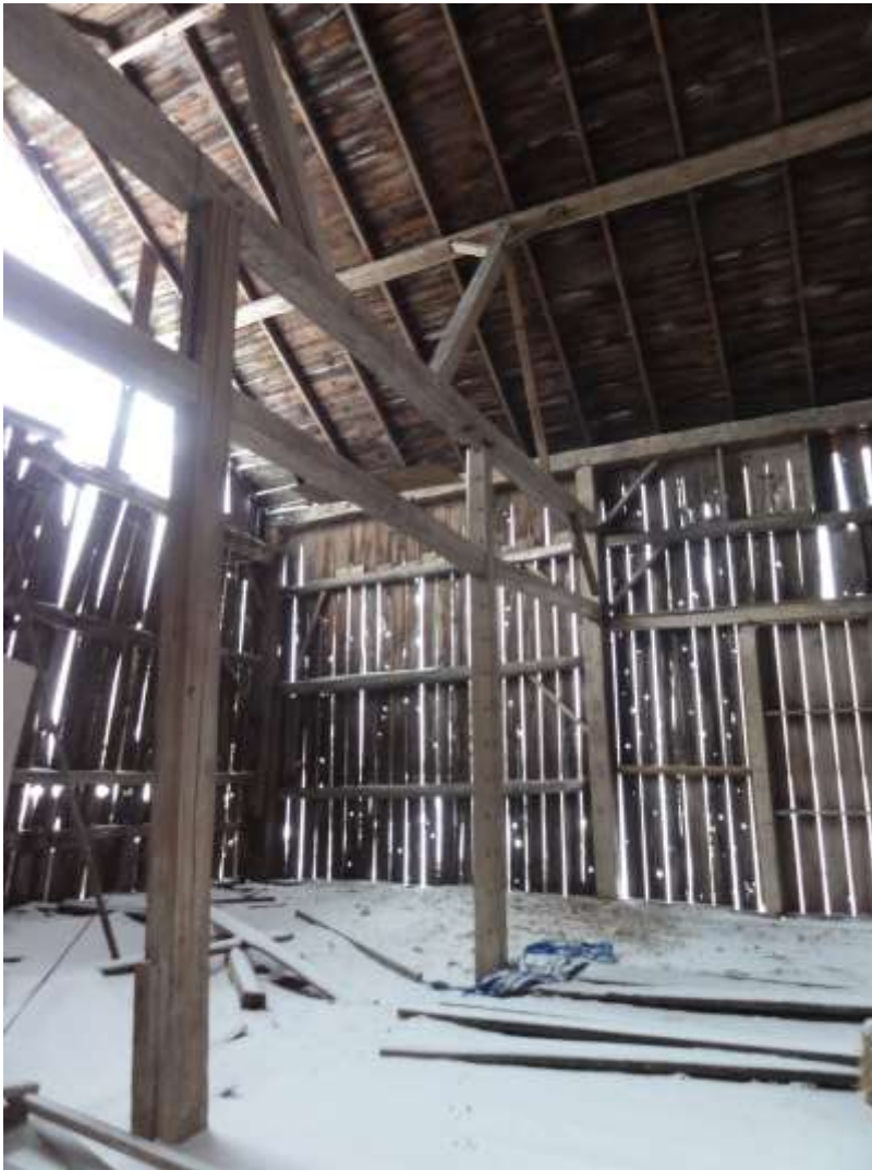
Image 7: View of barn interior illustrating damaged exterior bent and cladding, east face (2019-02-14).
