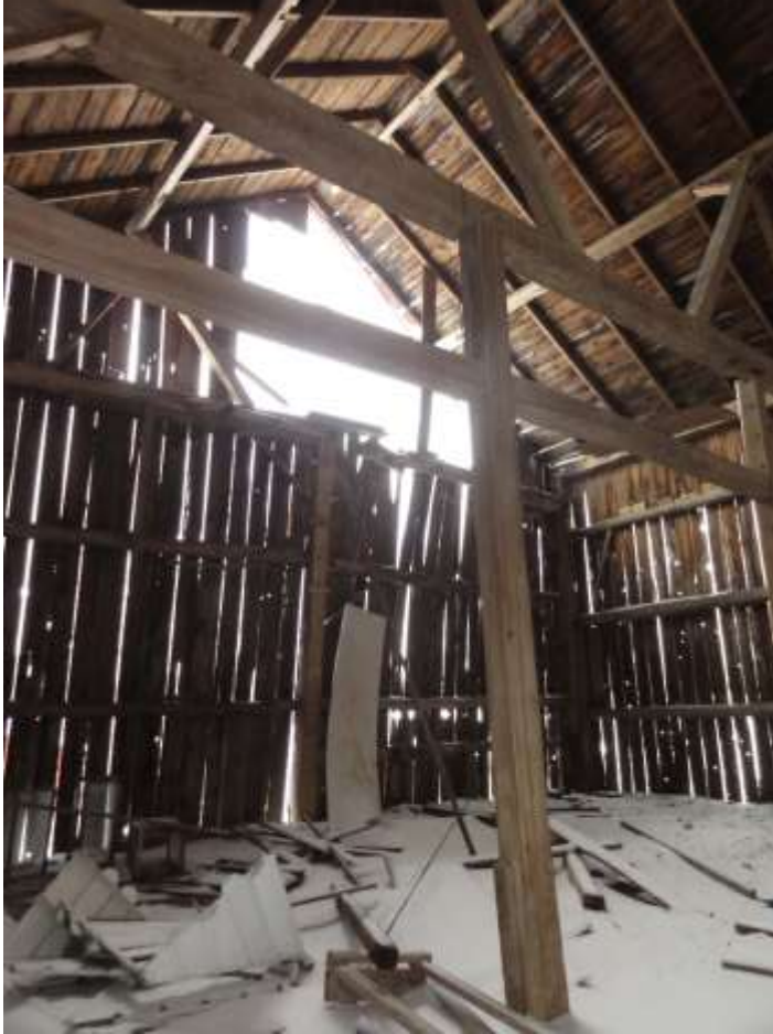
Image 9: View of barn interior illustrating damaged exterior bent and cladding, east face (2019-02-14).
